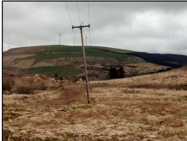
Pole leaning in bog area (possibly due to very soft founding strata)
