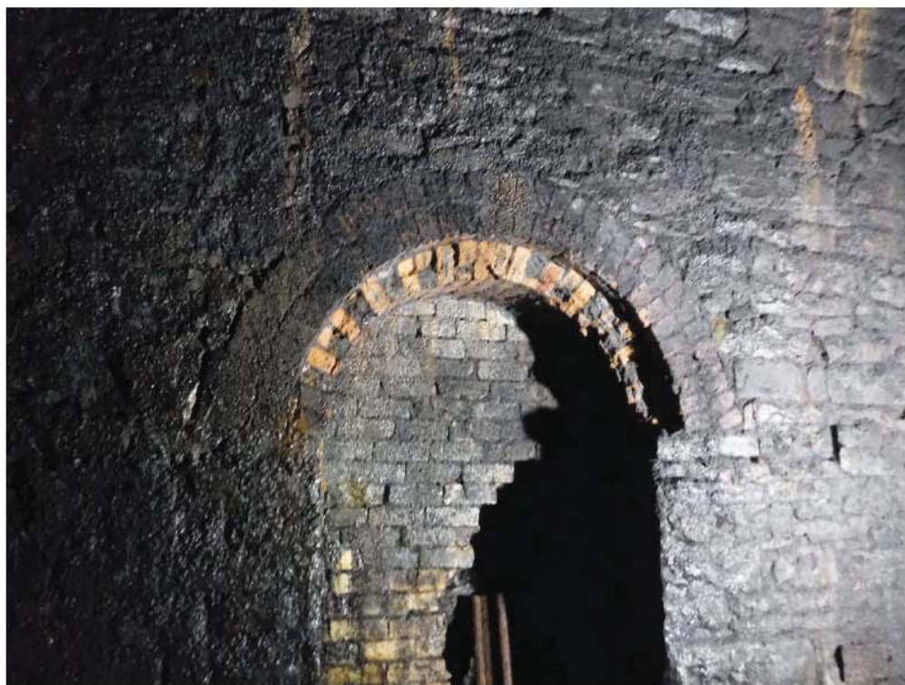
Photo No.20: 010+02 Refuge Up, Brickwork, Arch, spalled and missing bricks, depth 100mm, area 1.5sq.m.
