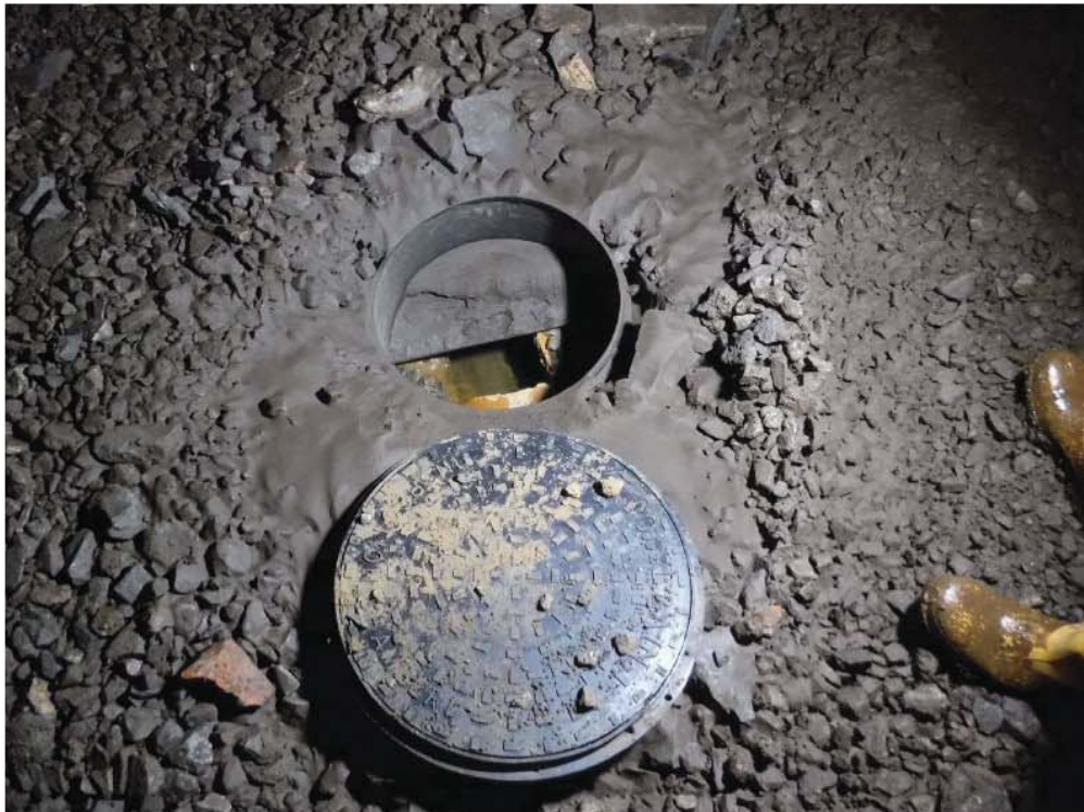
Photo No.33: 043+17 Solum Up & Down, Open Catch-pit to six-foot blocked, new flooding from 040+15 to 050+11 flowing northwards. Water subsided, new chamber, shallow mud/silt.
