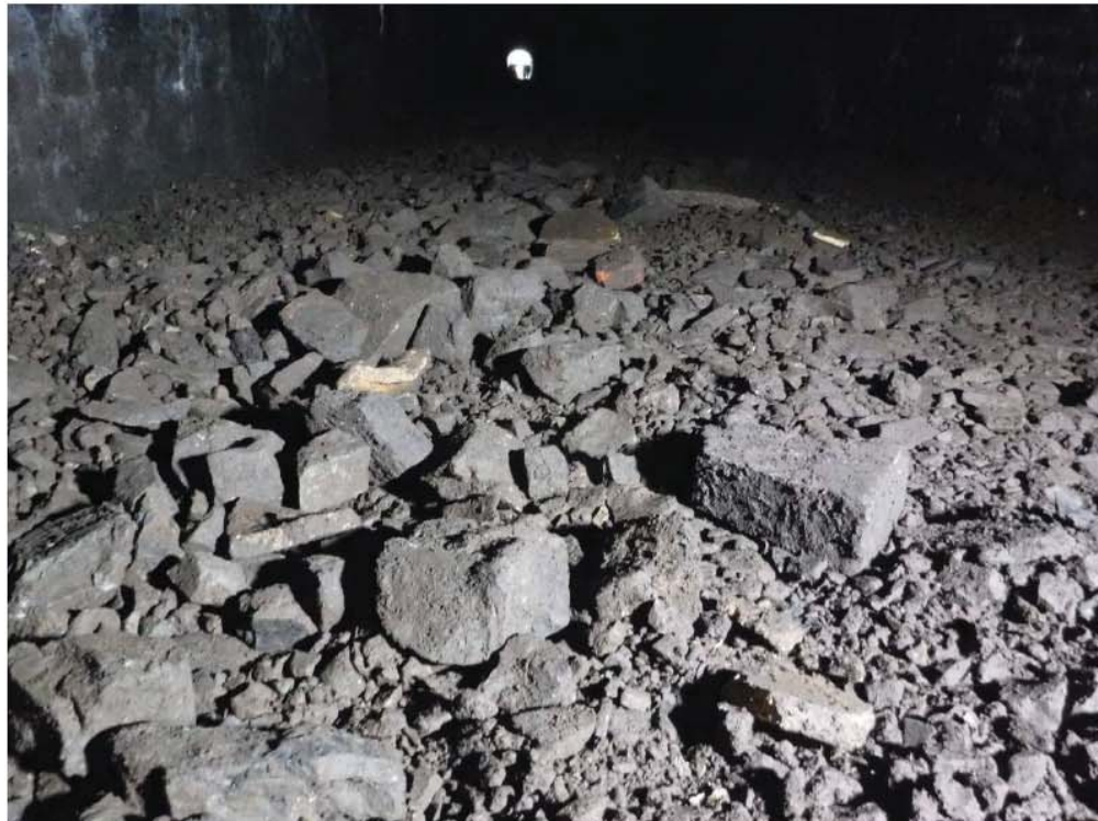
Photo No.11: Full Length of Tunnel, Solum Up & Down, drainage WIP, large ballast, bricks & smashed track drainage pipes churned up during excavation works, poor underfoot conditions, hazard.
