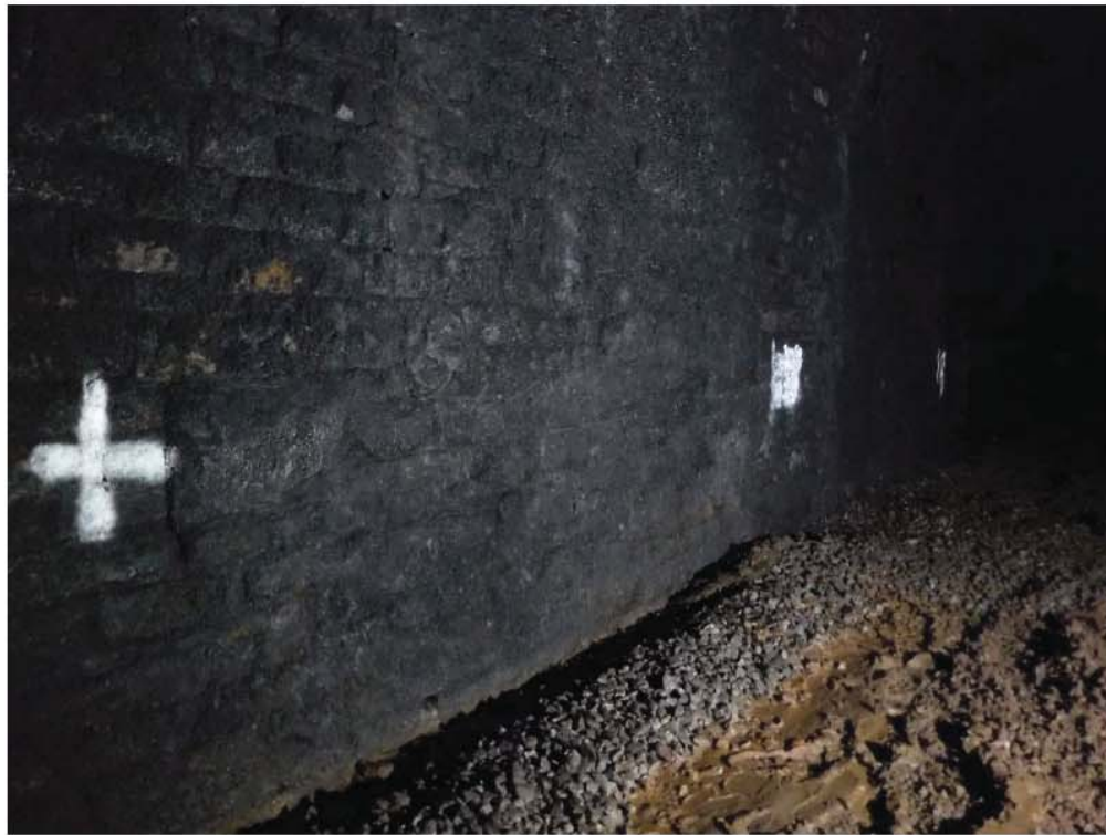
Photo No.10: Full Length of Tunnel, Sidewall Up, unnecessary & unsightly graffiti, large spray paint numbers and numbers sprayed over ostensibly to try to correct an initial measuring.
