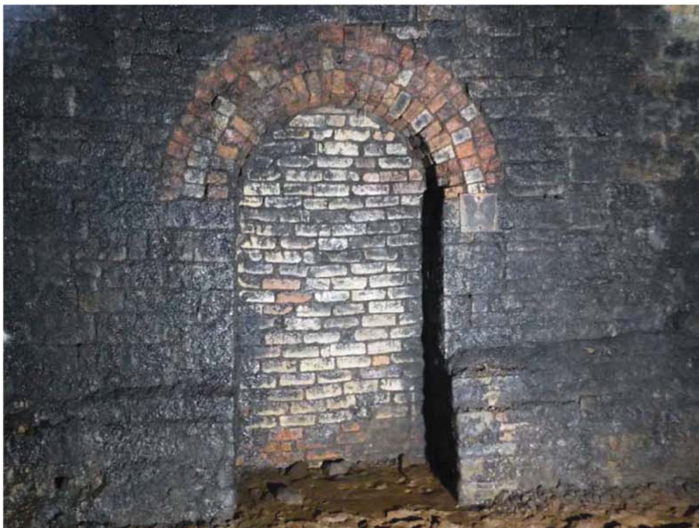
Photo No.21: 011+16 Refuge Up, Brickwork, Arch, spalling, depth 75mm, area 1sq.m., damp, light (archive photo).
