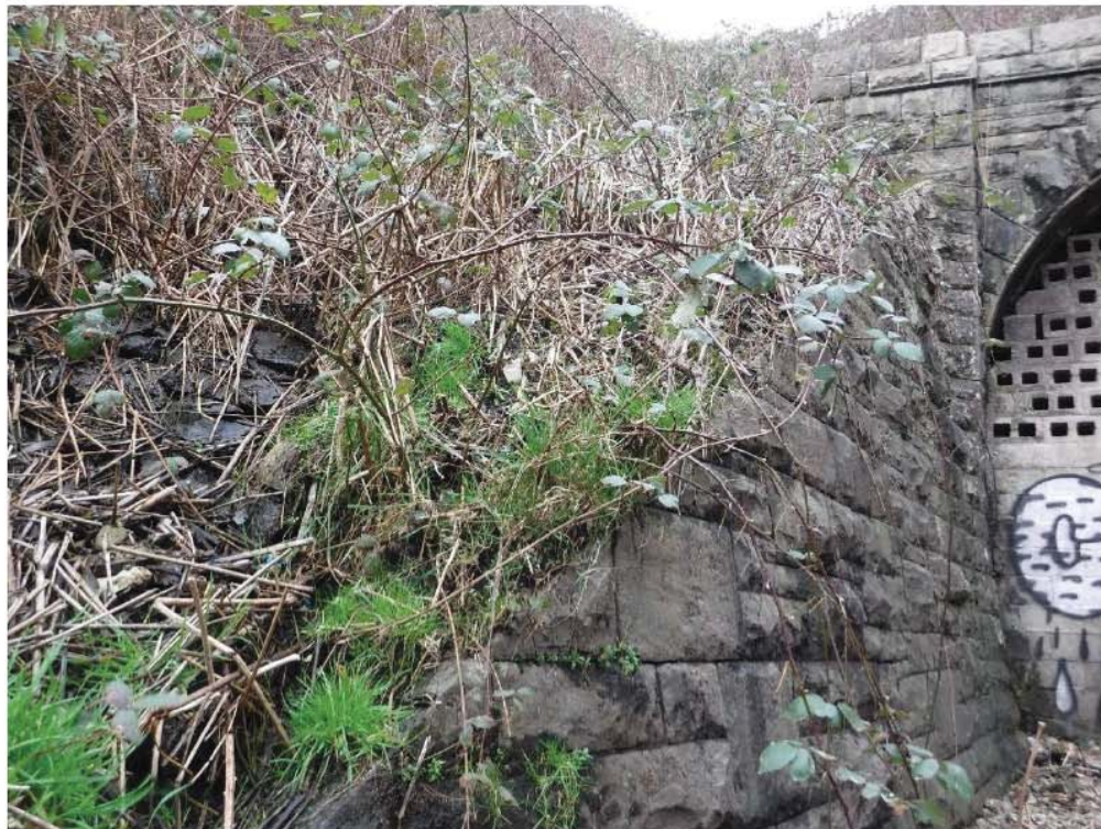
Photo No.1: Bridgend Portal Down, Wingwall, Copings missing and loose blocks, area 8sq.m.
