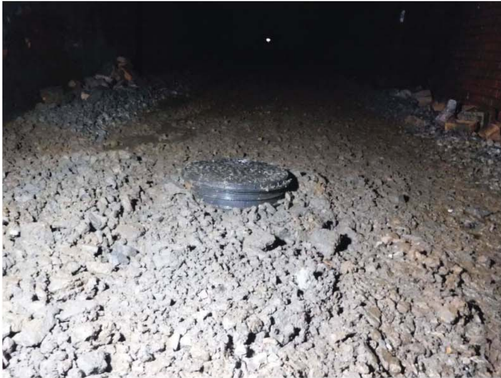
Photo No.28: 000+00 to 038+20 Solum Up & Down, drainage WIP, catch-pits and/or earthenware pipes broken out, new inspection chambers fitted mostly at 1ch centres, some covers missing or displaced.
