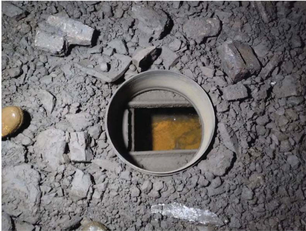
Photo No.24: 000+00 to 038+20 Solum Up & Down, drainage WIP, catch-pits and/or earthenware pipes broken out, new inspection chambers fitted mostly at 1ch centres, some covers missing or displaced.
