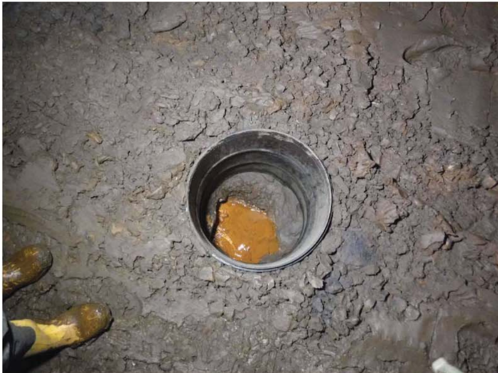
Photo No.25: 000+00 to 038+20 Solum Up & Down, drainage WIP, catch-pits and/or earthenware pipes broken out, new inspection chambers fitted mostly at 1ch centres, some covers missing or displaced.
