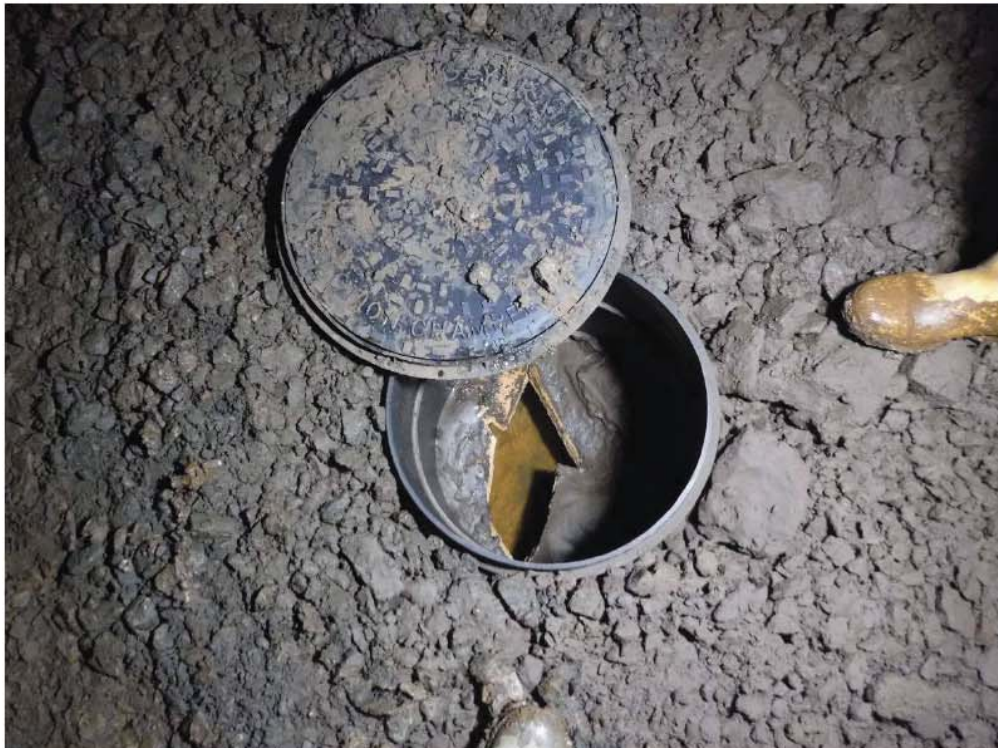
Photo No.29: 000+00 to 038+20 Solum Up & Down, drainage WIP, catch-pits and/or earthenware pipes broken out, new inspection chambers fitted mostly at 1ch centres, some covers missing or displaced.
