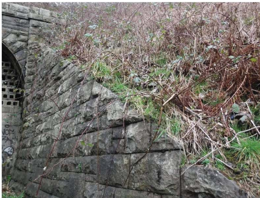
Photo No.2: Bridgend Portal Up, Wingwall, Copings missing and loose blocks, area 8sq.m.
