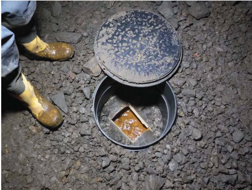
Photo No.26: 000+00 to 038+20 Solum Up & Down, drainage WIP, catch-pits and/or earthenware pipes broken out, new inspection chambers fitted mostly at 1ch centres, some covers missing or displaced.
