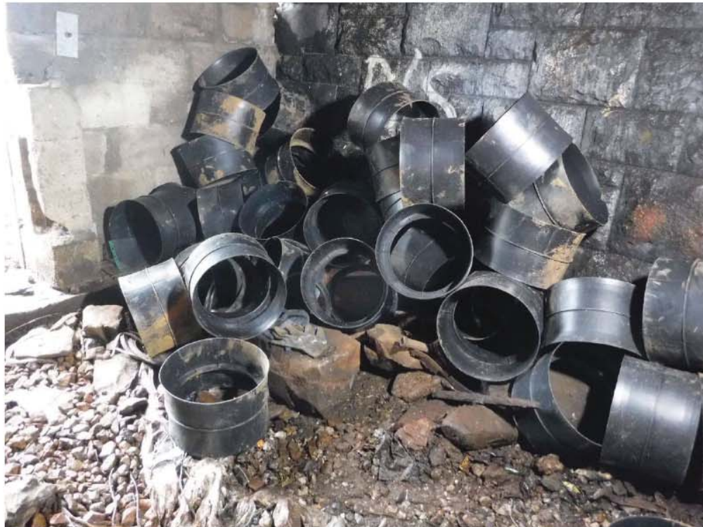
Photo No.15: Bridgend Portal, Solum Down, drainage WIP, new construction materials found in cess.
