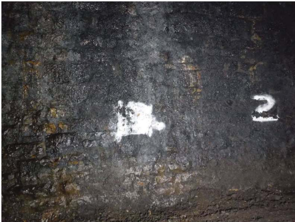
Photo No.7: Full Length of Tunnel, Sidewall Up, unnecessary & unsightly graffiti, large spray paint numbers and numbers sprayed over ostensibly to try to correct an initial measuring.
