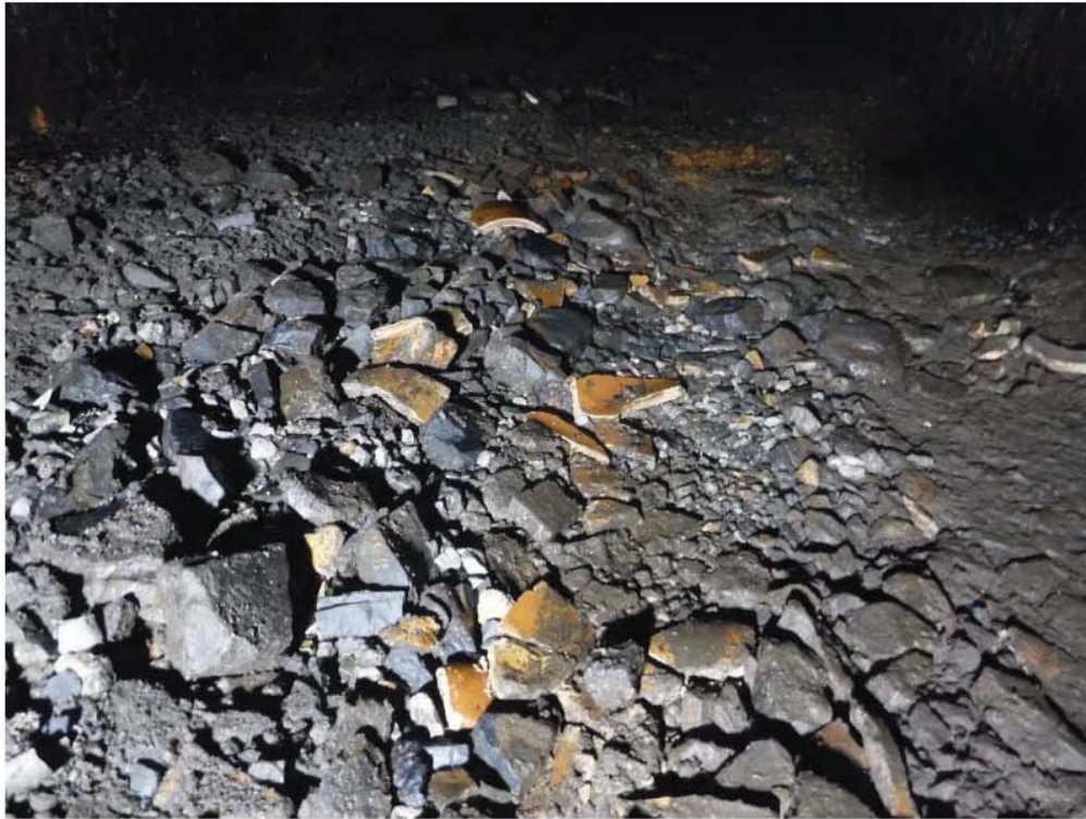
Photo No.12: Full Length of Tunnel, Solum Up & Down, drainage WIP, large ballast, bricks & smashed track drainage pipes churned up during excavation works, poor underfoot conditions, hazard.
