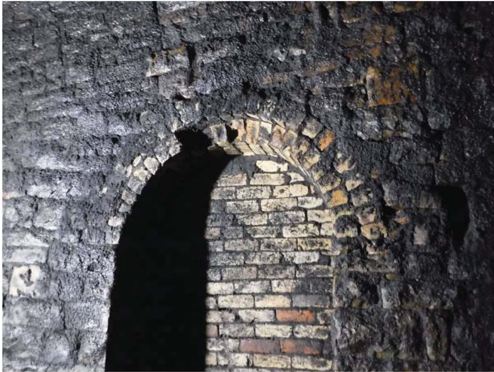
Photo No.22: 016+07 Refuge Up, Brickwork, Arch, hollow, area 1sq.m., with missing bricks, depth 100mm, area 0.25sq.m., medium.
