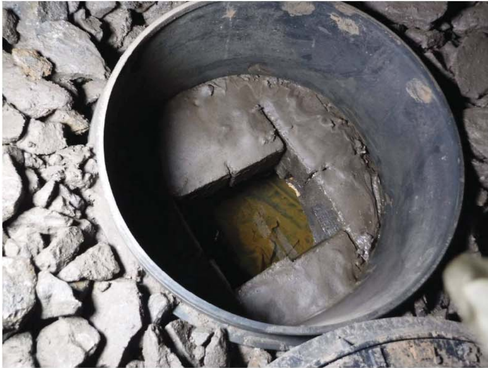
Photo No.30: 000+00 to 038+20 Solum Up & Down, drainage WIP, catch-pits and/or earthenware pipes broken out, new inspection chambers fitted mostly at 1ch centres, some covers missing or displaced.
