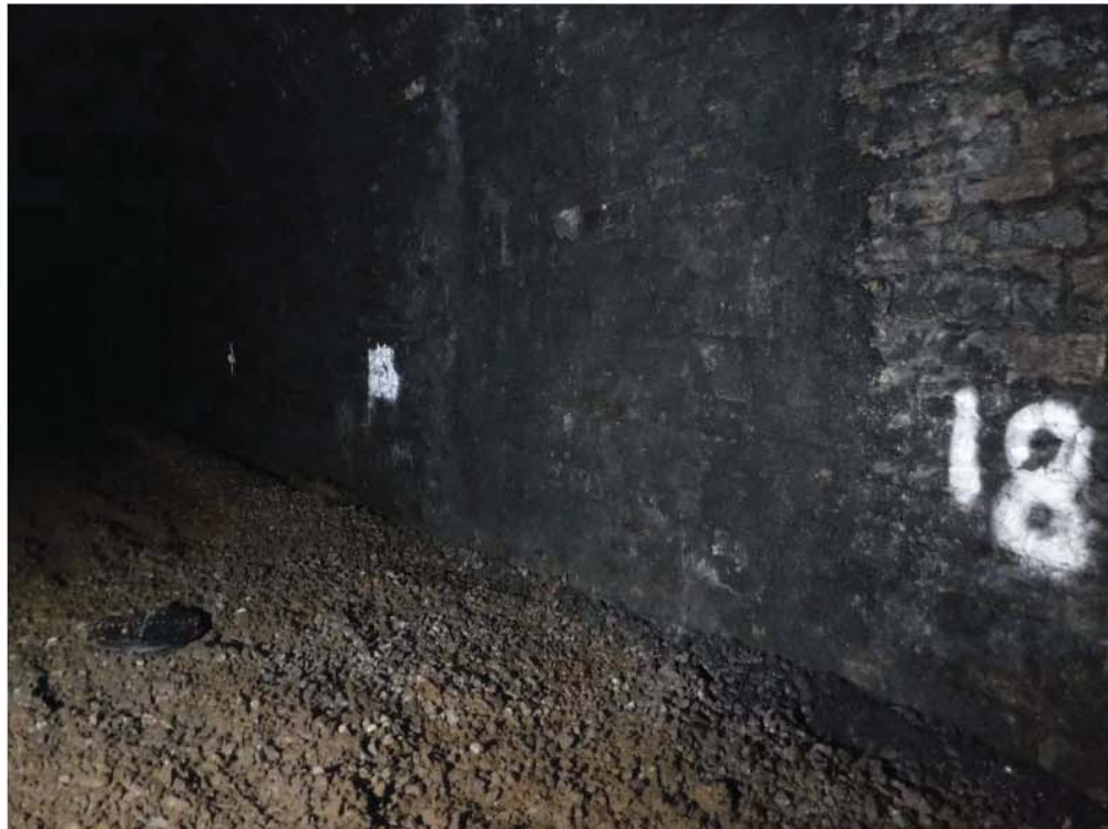
Photo No.9: Full Length of Tunnel, Sidewall Up, unnecessary & unsightly graffiti, large spray paint numbers and numbers sprayed over ostensibly to try to correct an initial measuring.
