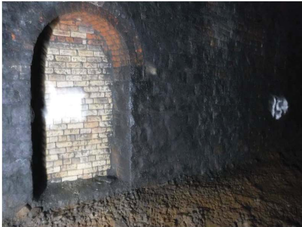
Photo No.8: Full Length of Tunnel, Sidewall Up, unnecessary & unsightly graffiti, large spray paint numbers and numbers sprayed over ostensibly to try to correct an initial measuring.
