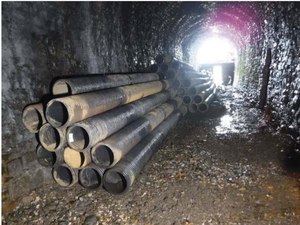
Photo No.19: Bridgend Portal, Solum Down, drainage WIP, old metal door dumped in tunnel hidden by a new stockpile of pipes.
