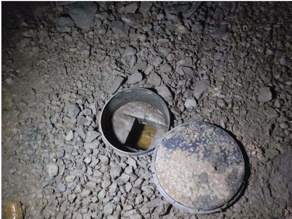
Photo No.31: 000+00 to 038+20 Solum Up & Down, drainage WIP, catch-pits and/or earthenware pipes broken out, new inspection chambers fitted mostly at 1ch centres, some covers missing or displaced.
