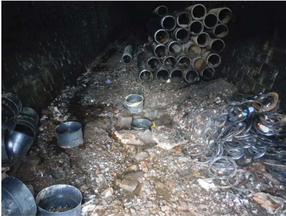
Photo No.18: Bridgend Portal, Solum Down, drainage WIP, old metal door dumped in tunnel hidden by a new stockpile of pipes.
