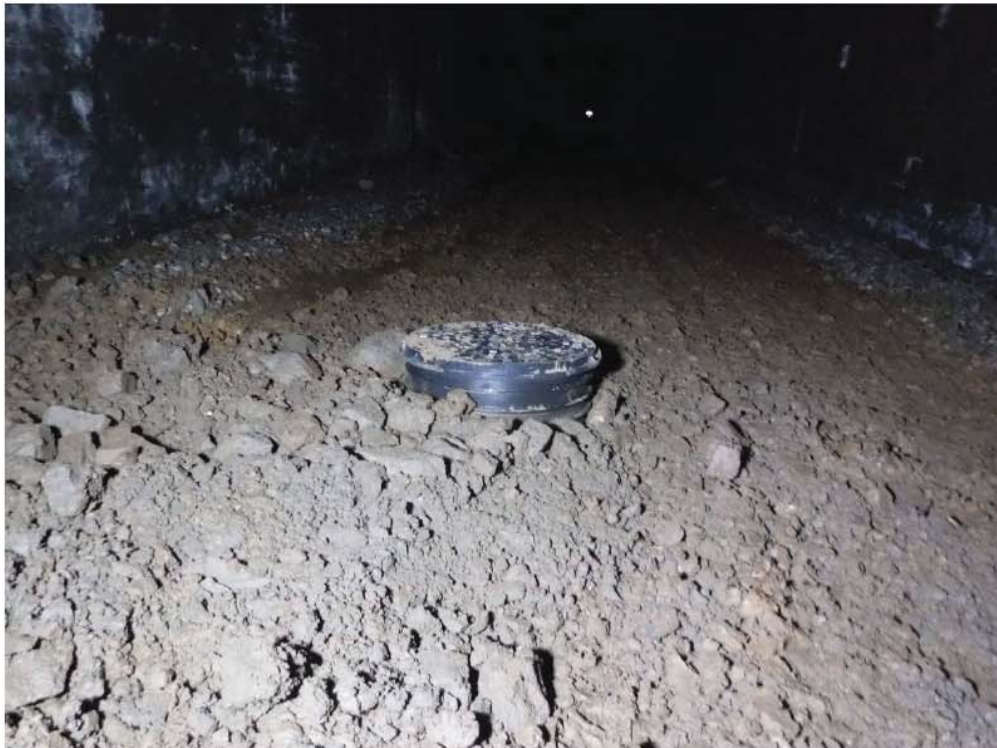
Photo No.27: 000+00 to 038+20 Solum Up & Down, drainage WIP, catch-pits and/or earthenware pipes broken out, new inspection chambers fitted mostly at 1ch centres, some covers missing or displaced.
