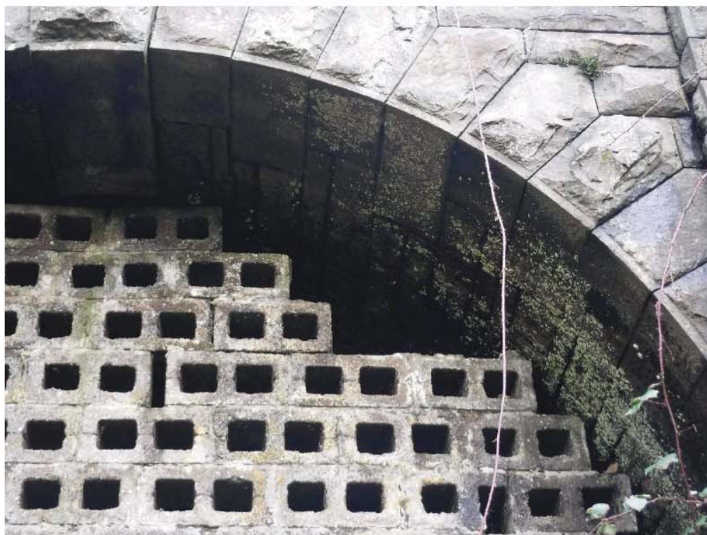
Photo No.3: Bridgend Portal Up, missing & loose blockwork, gap allows easy trespass access into tunnel.
