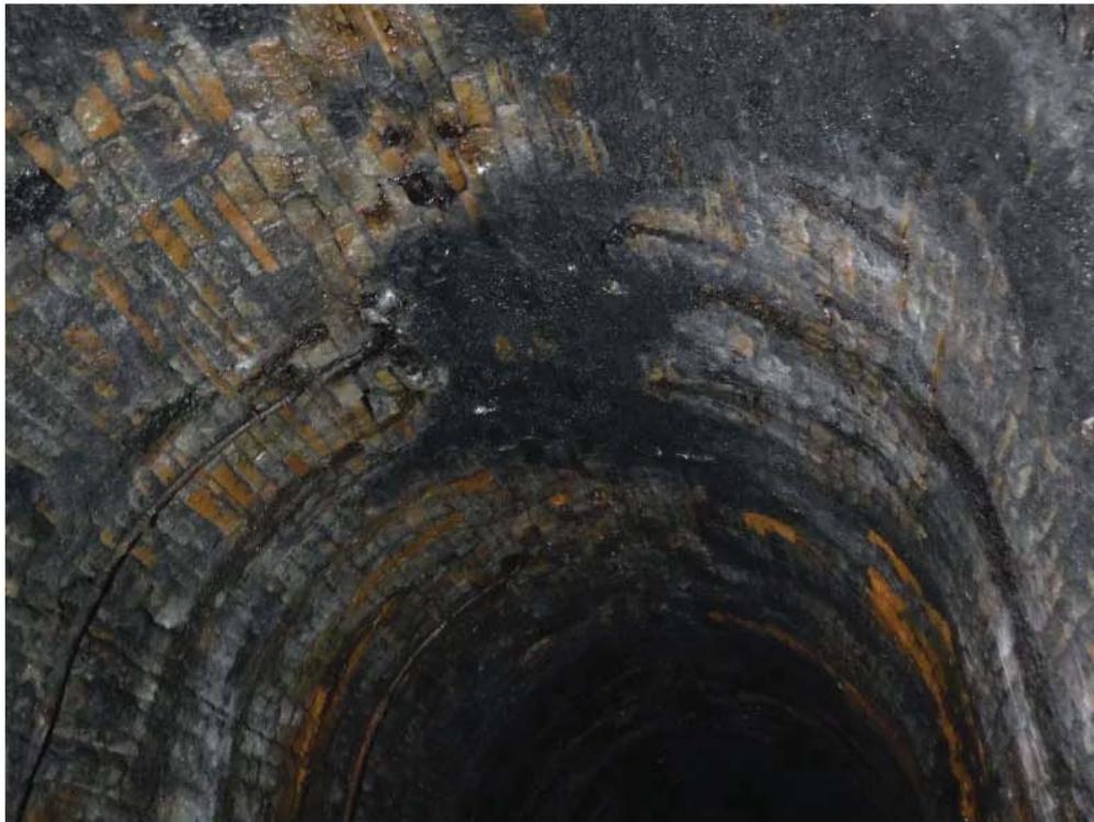
Photo No.23: 016+18 Sidewall & Haunch Down, Stonework, 2No. downpipes fitted to Haunch with running water. Possible Hidden Shaft.
