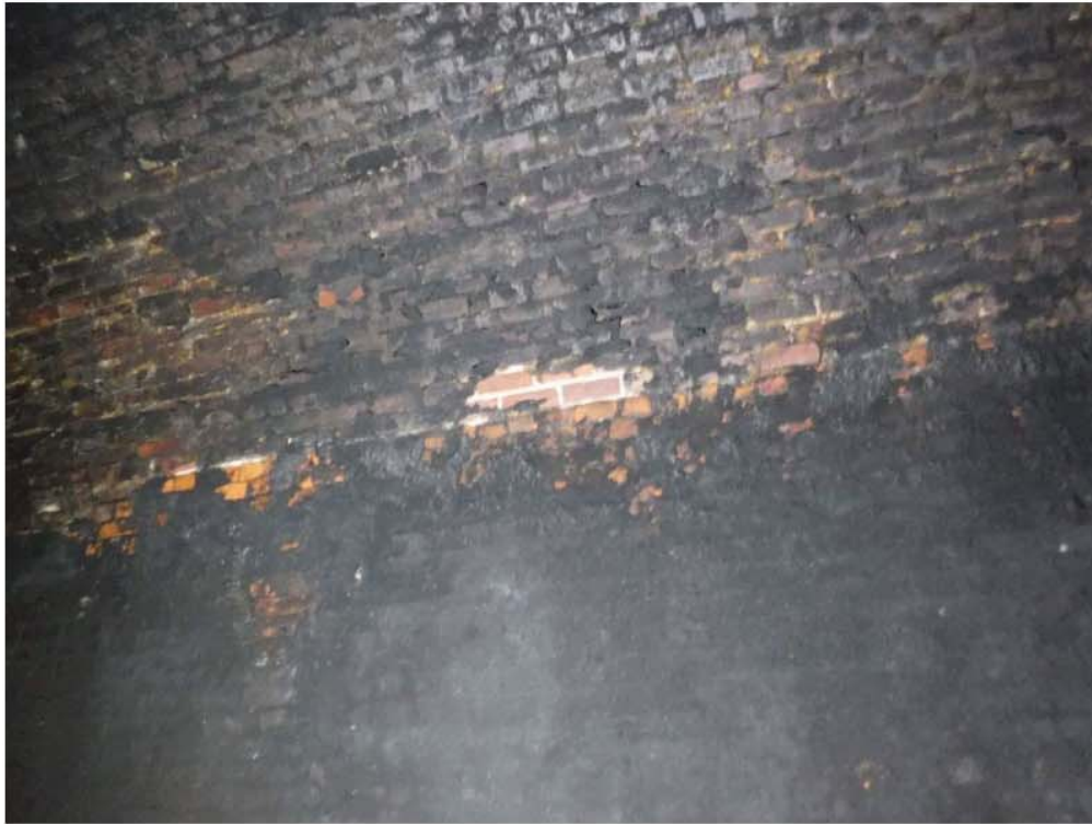
Photo No.32: 042+13 to 043+20 Low Haunch Up & Down, Brickwork, longitudinal cracking, width 1mm, length 27m. Various bricks crushed and spalled to downside, depth 25mm, area 3sq.m.
