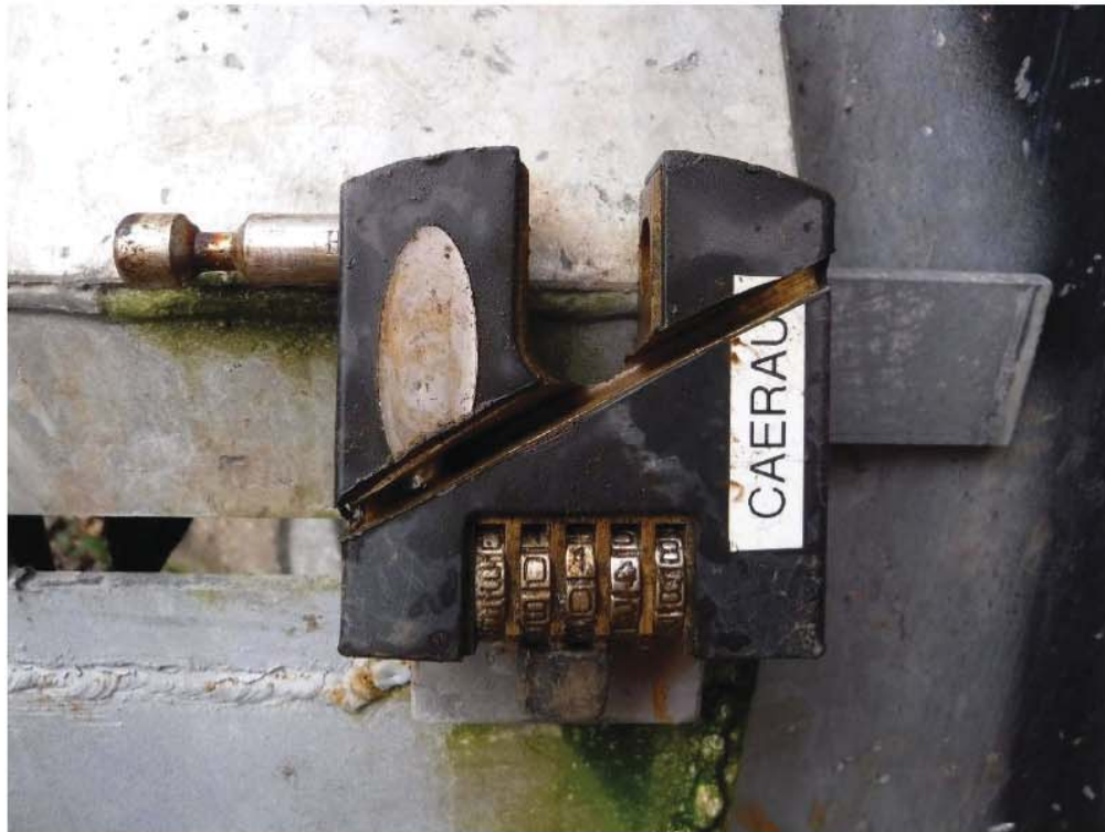
Photo No.4: Bridgend Portal, existing padlock found cut-off on the solum reason unknown, tumblers still operable.
