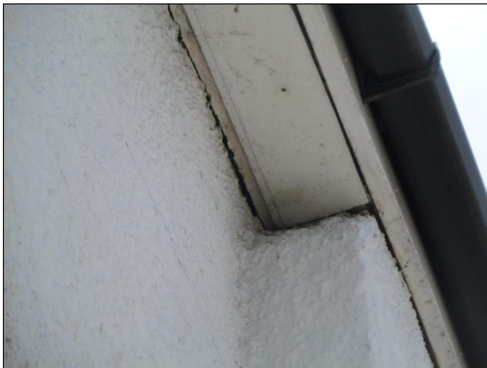
Photo 6: uPVC soffit with gaps on eastern elevation.
