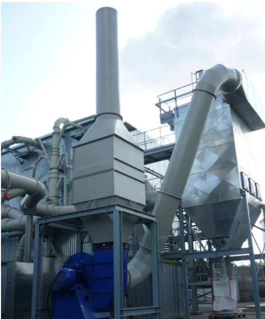
Filter housing (on the right) with ducting, fan (blue coloured), silencer and stack
