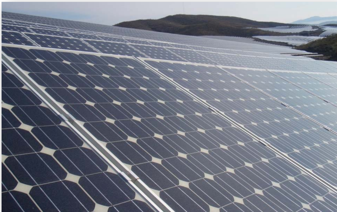
Plate 1: Typical Solar Panel
