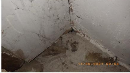
Gap in plasterboards in west eave storage area
