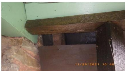
Gaps leading into the porch roof
