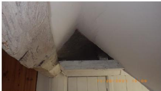
Gap above storage area D
