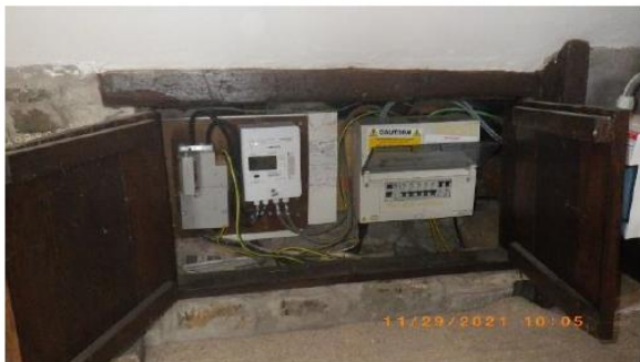
Inside meter cupboard E
