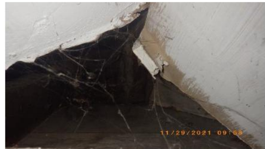
Gaps leading to the area below the roof tiles in storage area D
