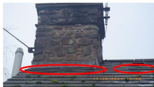
Uneven slates around the south chimney
