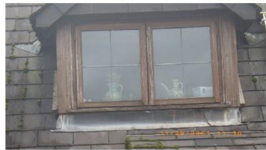
Gaps where dormer windows join with the roof
