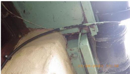
Gap in soffit on the west elevation of the house
