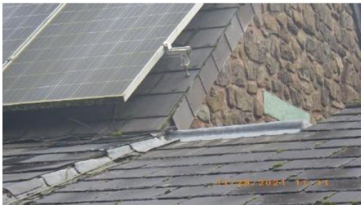
Raised lead and tiles along join with the south and west extensions
