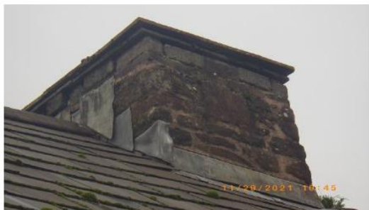
Gaps in north chimney and under lead flashing
