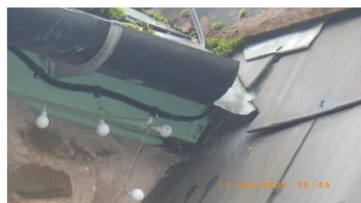
Slipped tiles on the house porch
