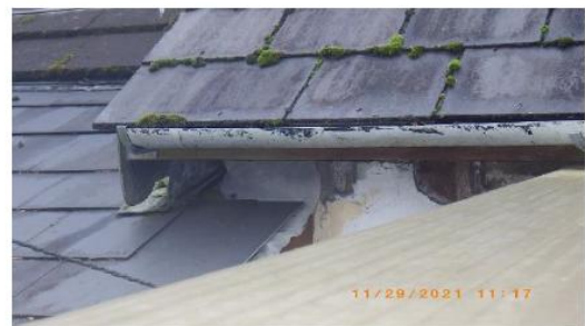
Exposed tile edges gaps in render on north side of the west extension
