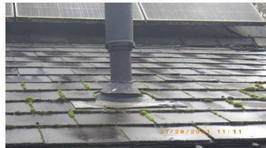
Uneven slates around the flue on the west elevation
