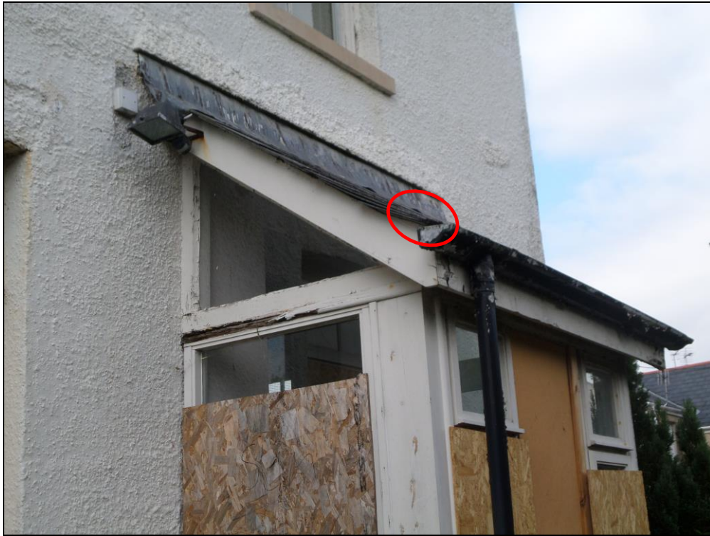
Photo 9: Small gaps under rear porch roof (view looking north).
