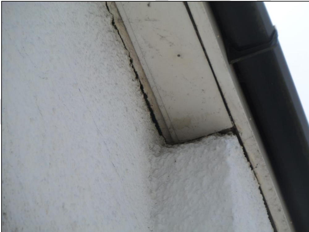
Photo 6: uPVC soffit with gaps on eastern elevation.
