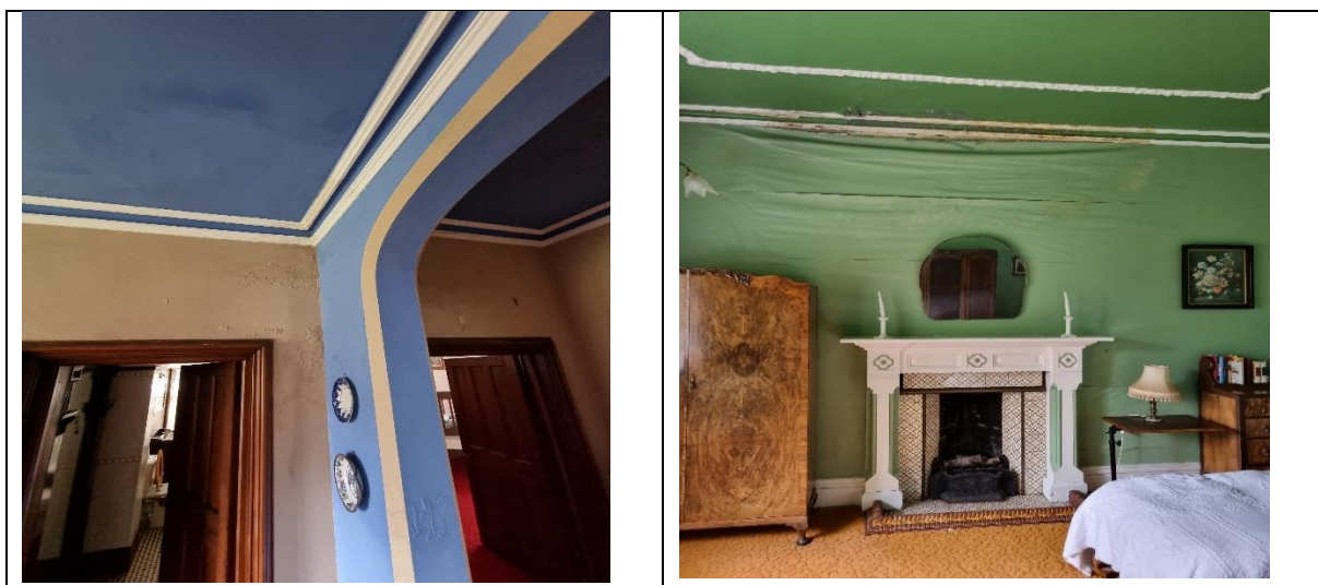
Fig.21 Water ingress damage to walls and ceilings
