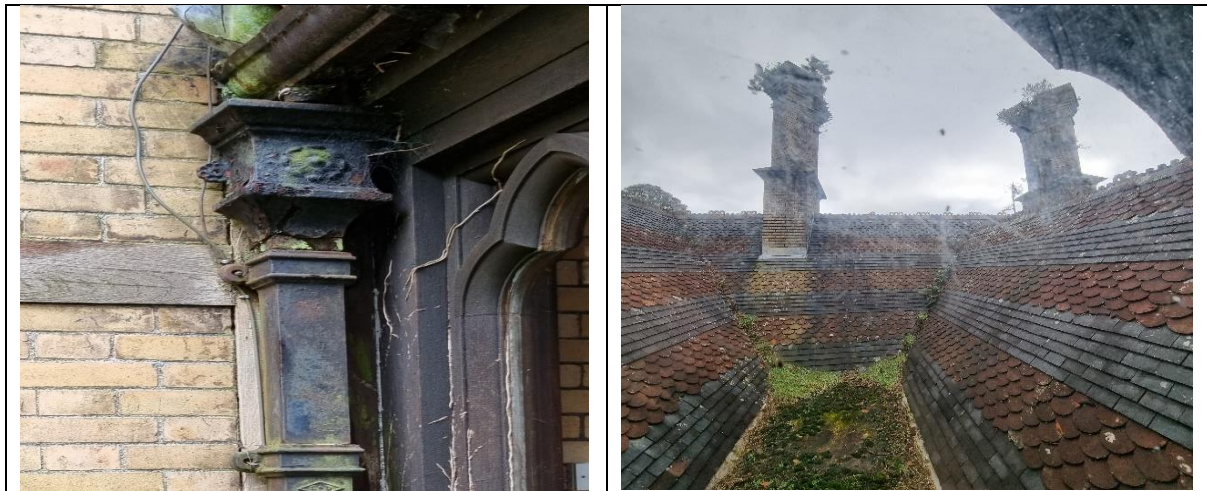
Fig.19 Split cast iron guttering and blocked drains on the roof
