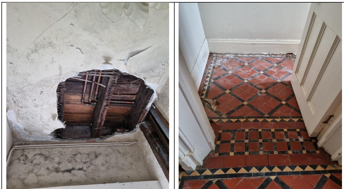
Fig.22 Water ingress damage to ceilings and tiled floors
