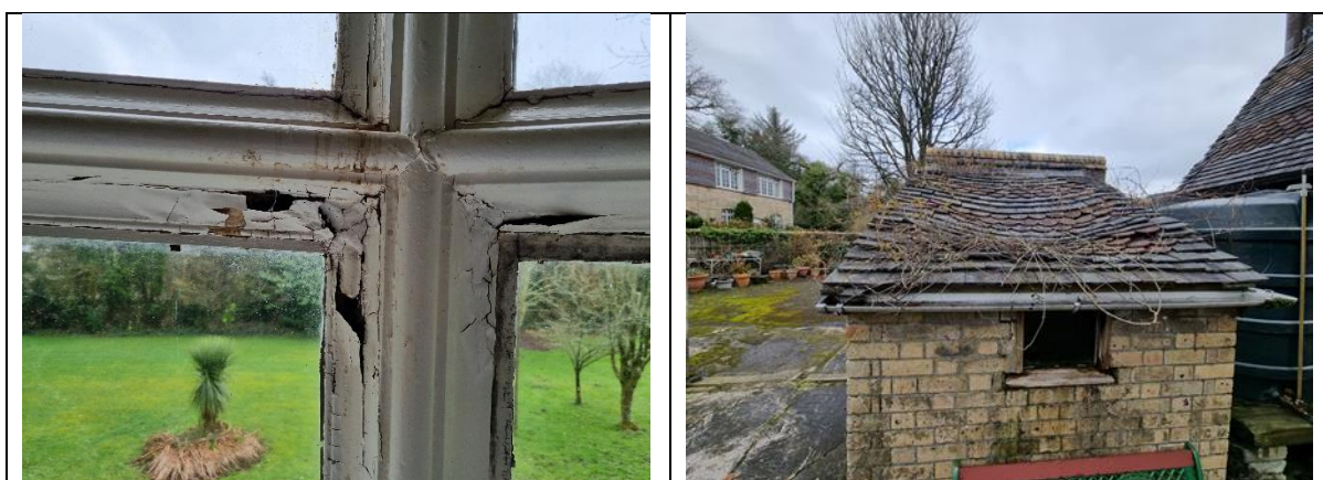
Fig.22 Water ingress damage to ceilings and tiled floors
