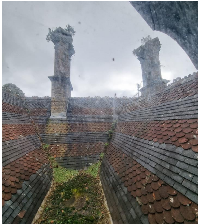
Fig.7 Centre gutter with foliage growth to chimneys
