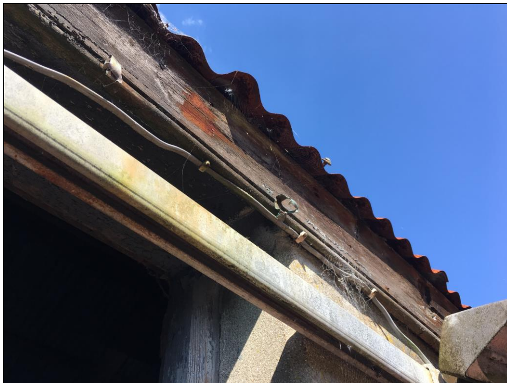
Photo 2: Gaps beneath fascias and corrugated metal roof on eastern elevation (view looking west).
