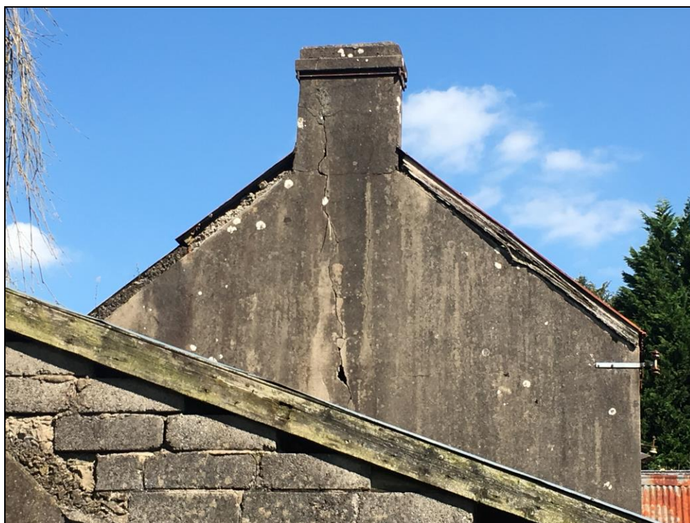
Photo 3: Southern gable end with rotten fascias, vertical crack down chimney breast and droppings identified on wall at eastern extent of elevation (View looking north).
