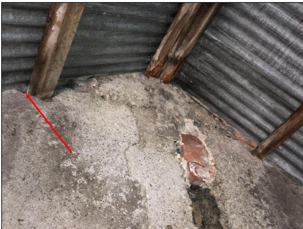
Photo 10: Southern gable end of interior with roost location and crack in chimney breast (view looking south).
