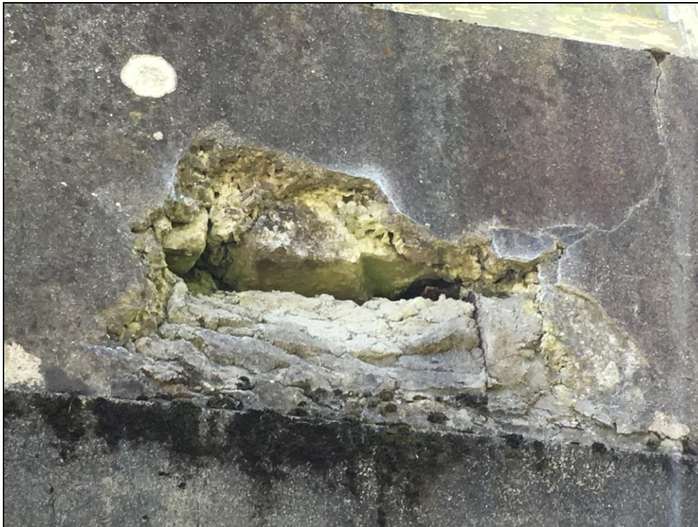
Photo 8: Crack in lintel on eastern elevation.
