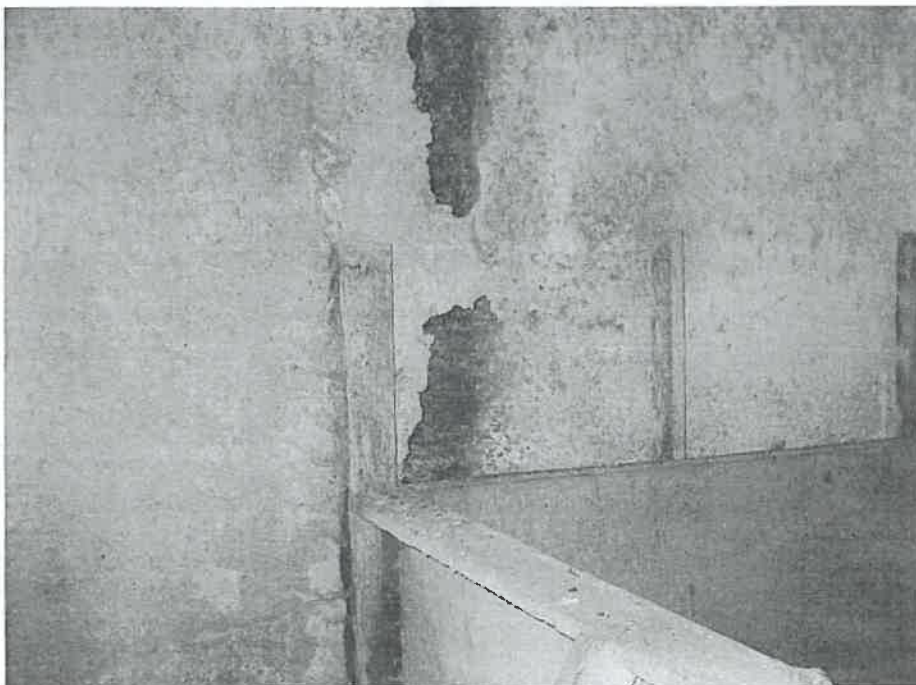
Photograph number 14-Sulphate damage to the gable wall
