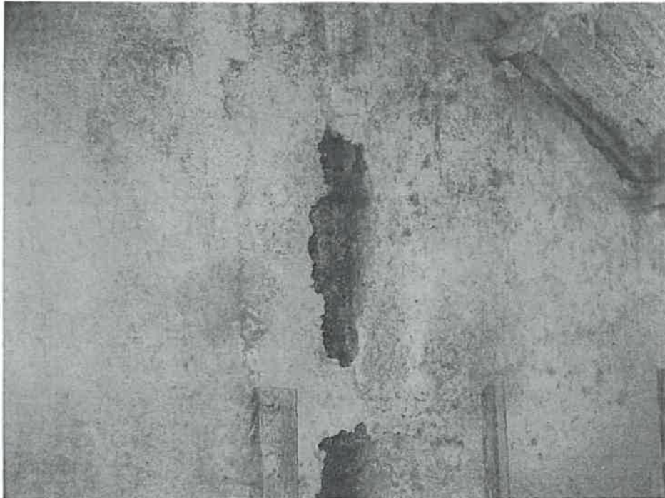
Photograph number 13-Sulphate damage to the gable wall
