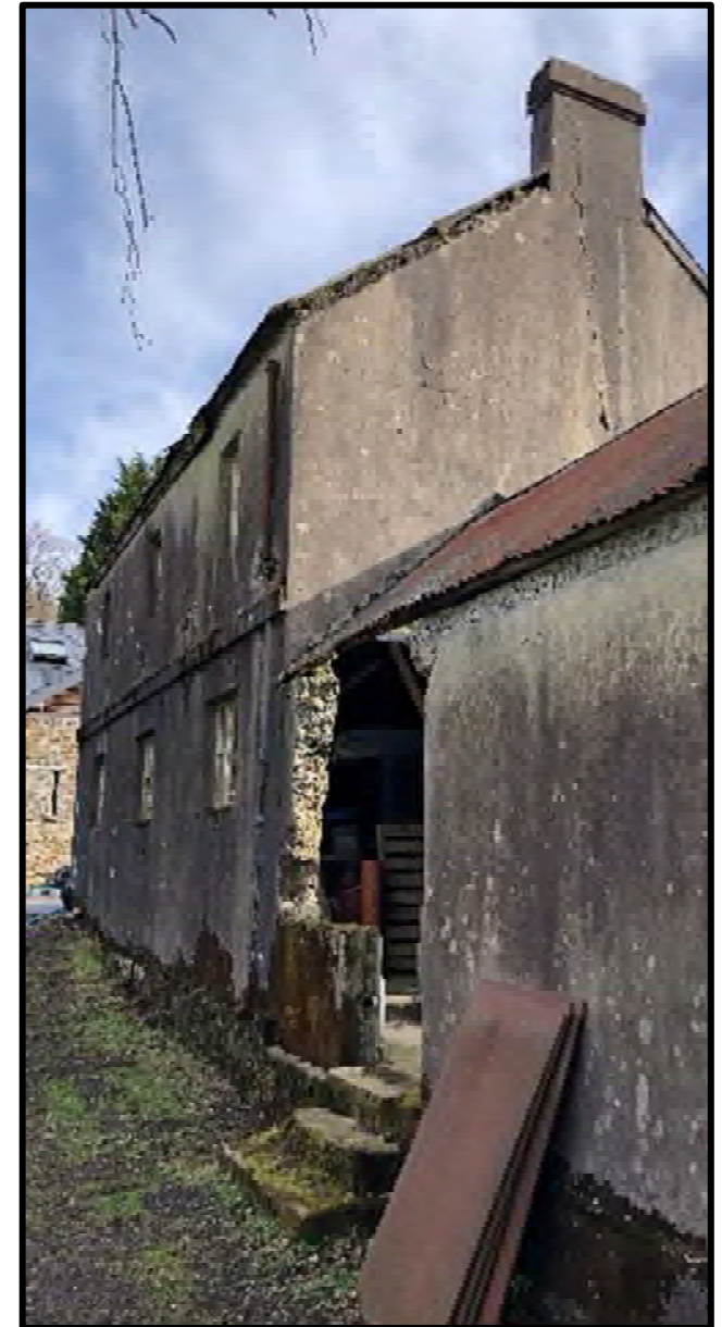
The photographs above show the current condition of the existing mass concrete walls – some areas have collapsed and large cracks have developed elsewhere
