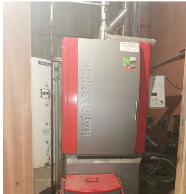
Plas Farm's existing wood pellet district heating system
