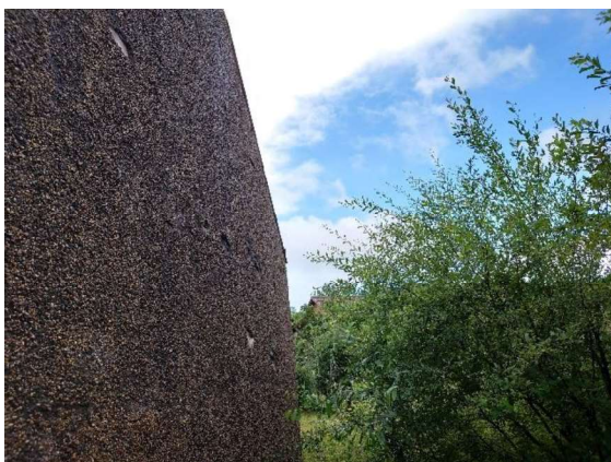
Photograph 3: Areas of exposed brickwork where concrete render has fallen off.
