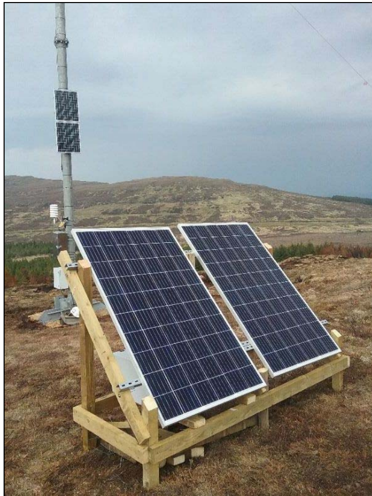
Photo 1: Typical Solar Power Supply Array
