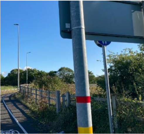
Photo 2-9 - Existing advanced directional signage hides the footway status sign that also indicates incorrect status
