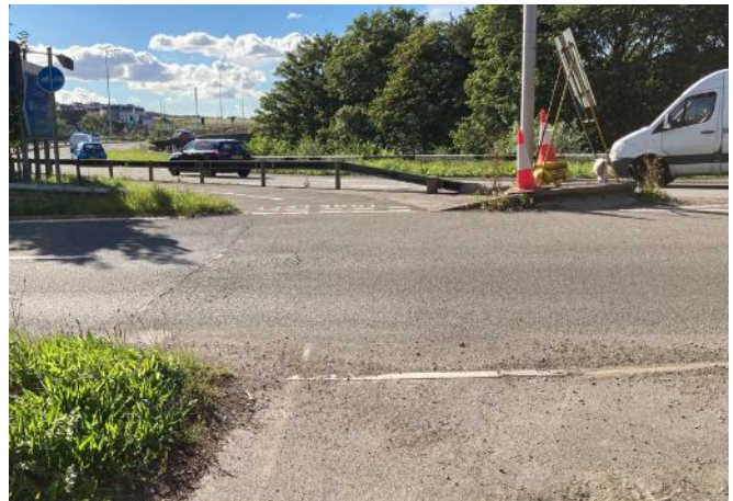
Photo 2-27 - The crossing point across the eastbound on-slip is not aligned, lacks tactile paving and shows signs of minor ponding
