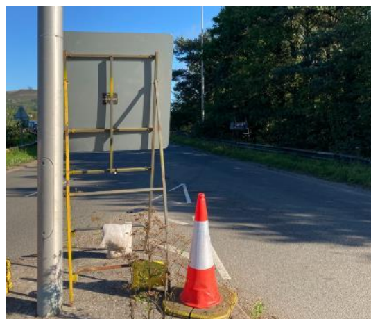
Photo 2-23 - Temporary signage completely blocks visibility between motor vehicles and segregated path users (looking towards A465 from the southern side of the eastbound on-slip crossing)
