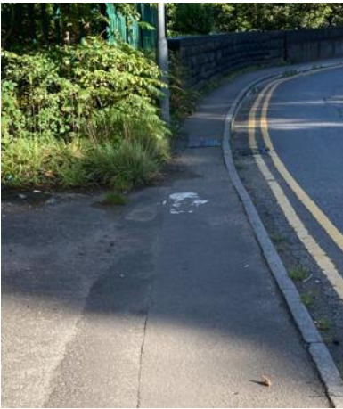
Photo 2-32 - Narrow footway (approx. 0.3m) across railway line on Pen-Y-Heol
