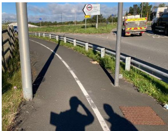
Photo 2-15 - Pinch point on segregated path due to sign posts and unsuitable utility cover for cyclist tyres.
