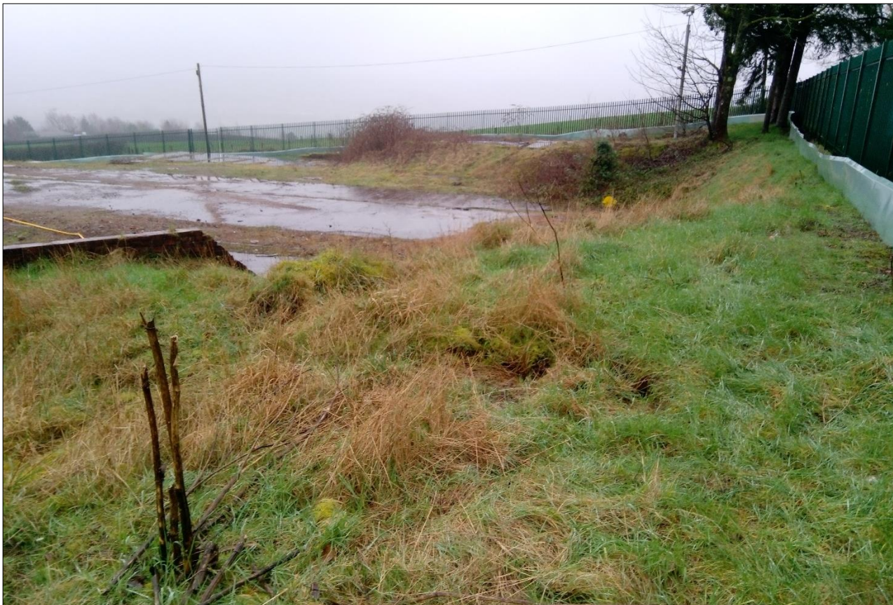
Figure 10. View on top of embankment immediately behind winged wall. Slight depression visible from ground surface level.
