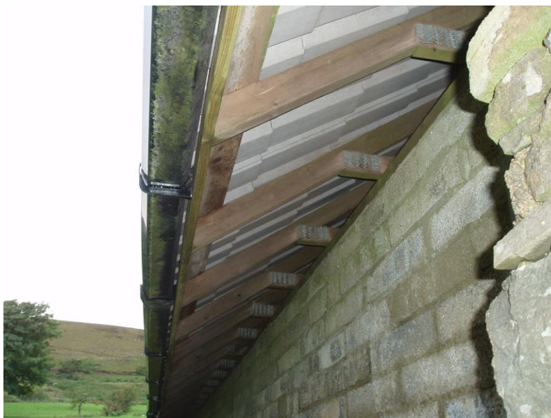
Gap between the new roof and the walls
