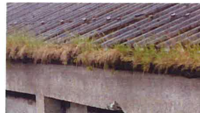
Close up of overgrowth (June 2017)
