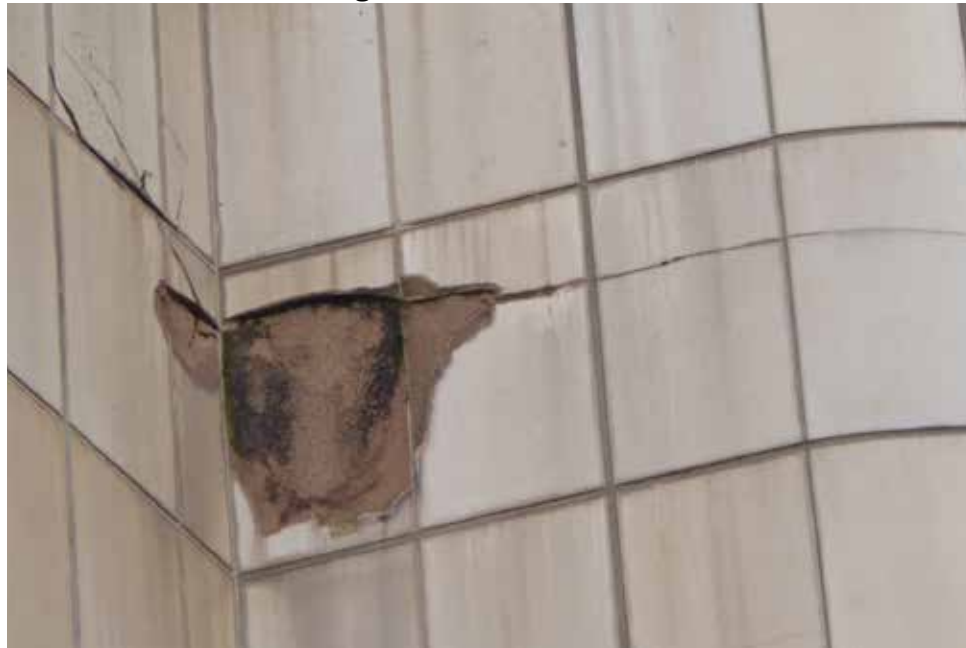
B Faience Tiling probably needing replacement
