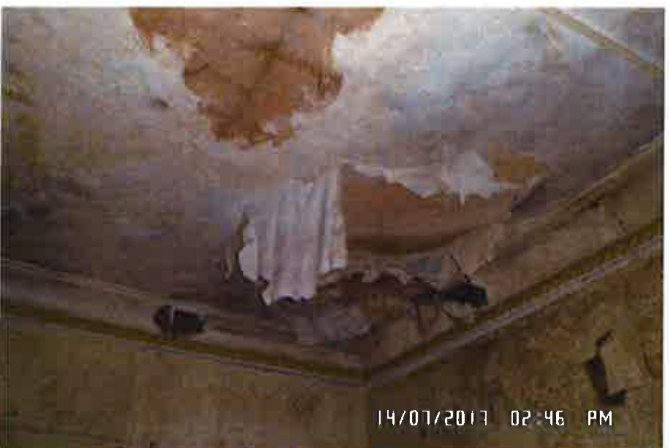
Cracked ceiling slab/damp, July 2017
