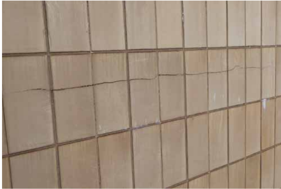
A Cracks in Faience Tiling
