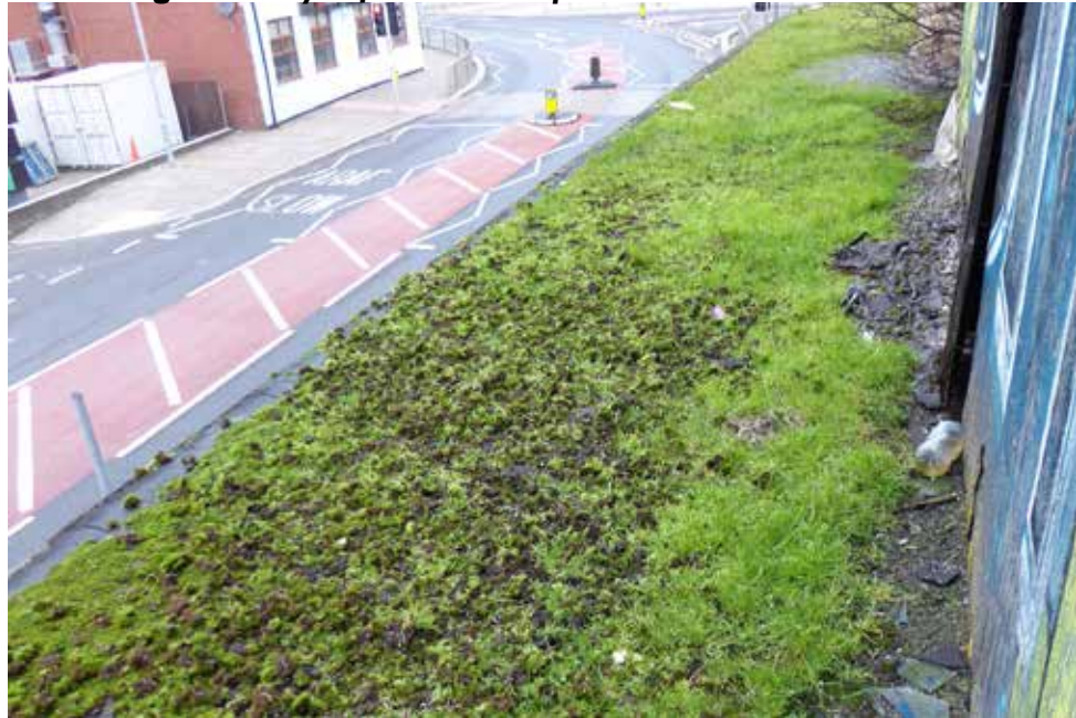
S Canopy Bitumen Roof to be Replaced
