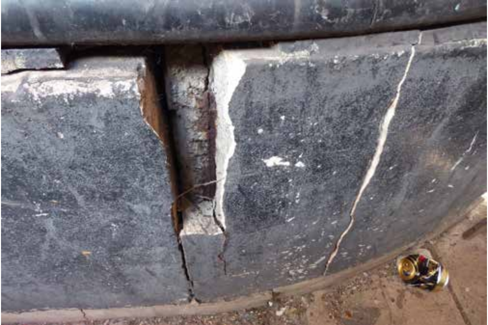
N Example of Damage to Masonry
