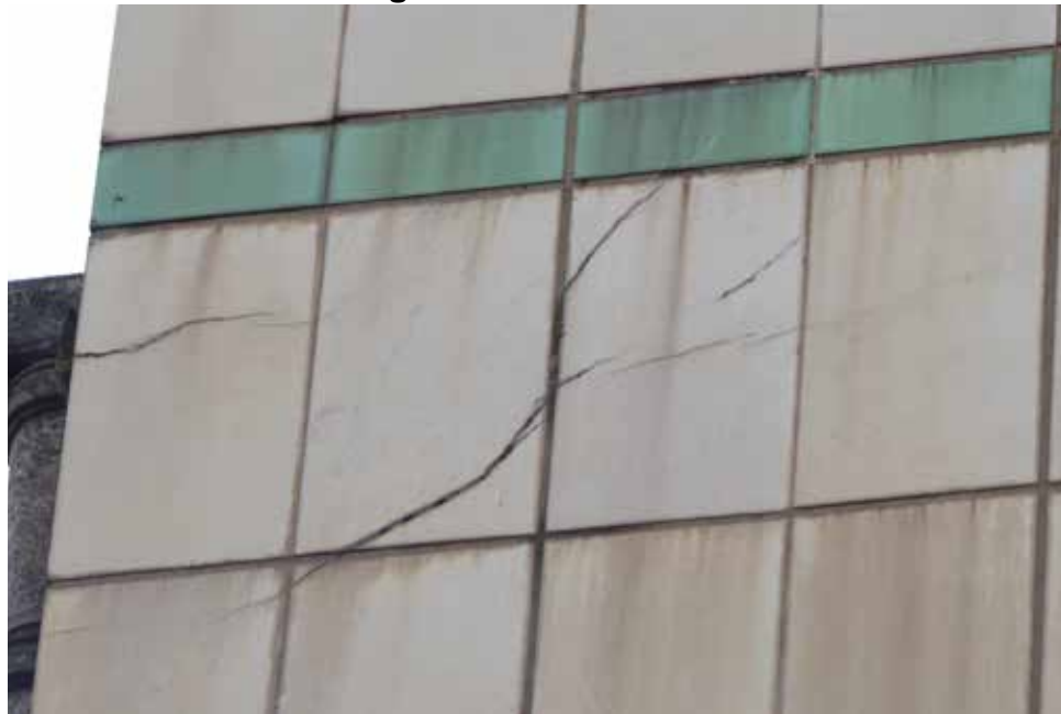
A Cracks in Faience Tiling
