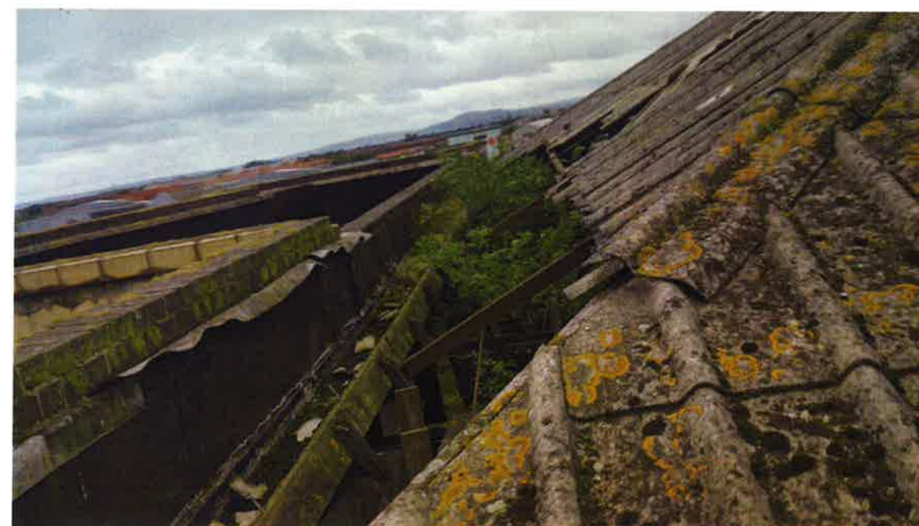
Broken section of asbestos cement roof sheeting, exposed steel trusses (rusted) to the elements (Photograph taken from MEWP July 2017)
