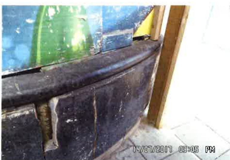
Additional cracking July 2017
