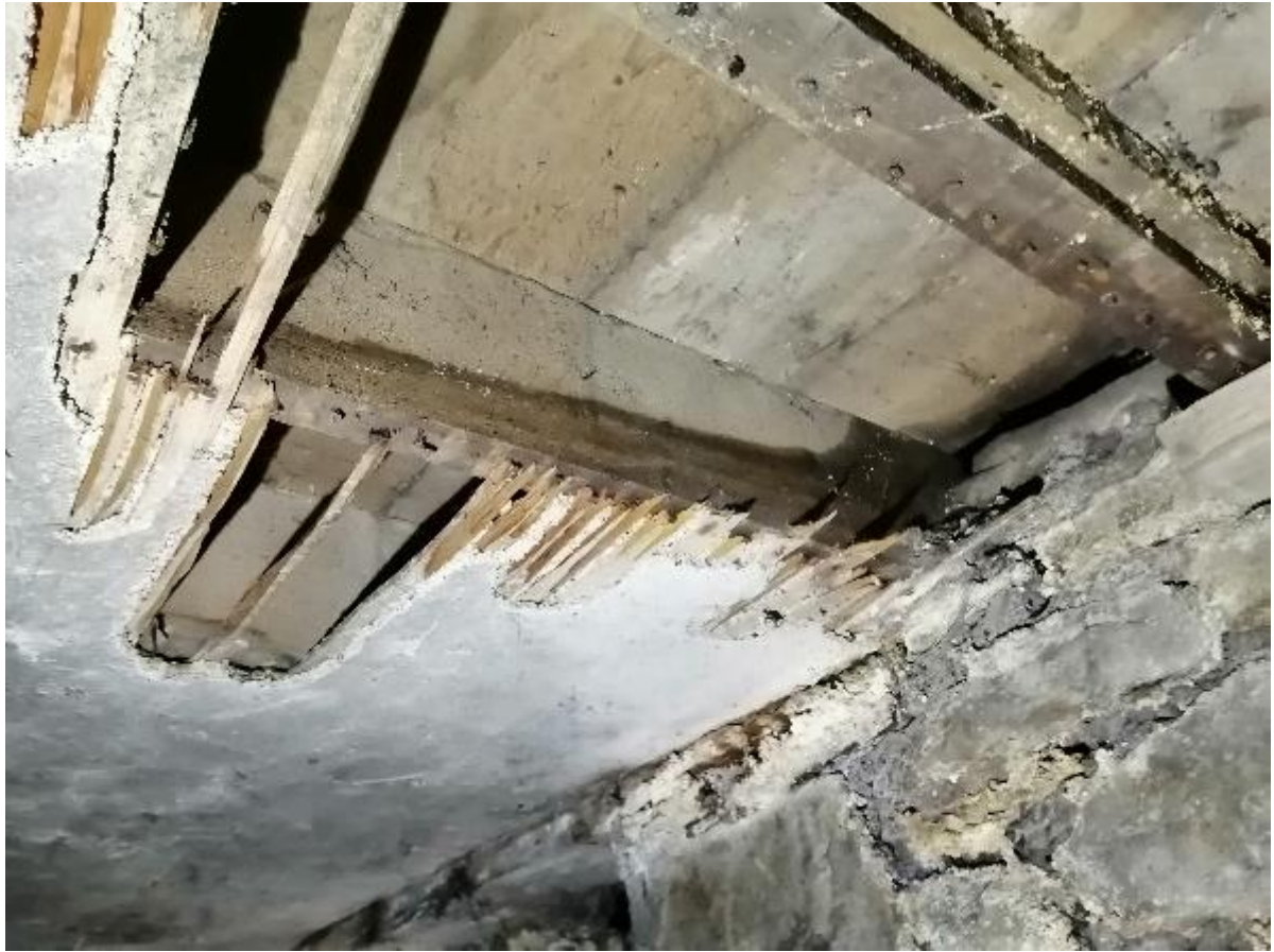
Photo 67 – Damp to Ends of Floor Joists (Basement Room 4)
