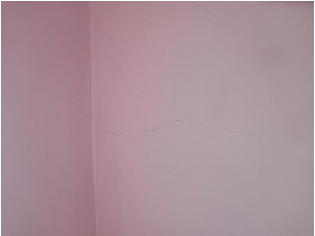
Photo 32 – Wall Plaster Crack (Bathroom)
