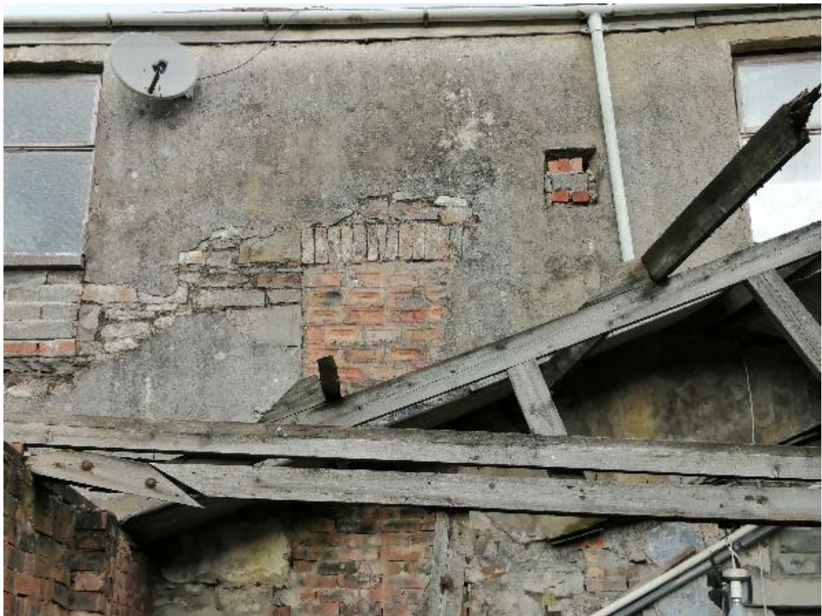
Photo 7 – Missing Render (Rear Wall Elevation)
