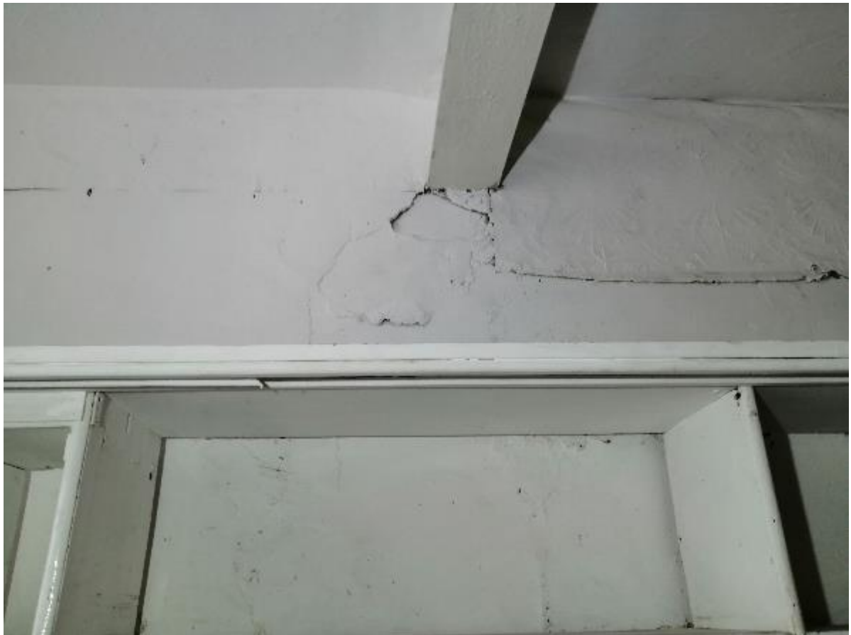
Photo 53 – Cracked and Detached Plaster (Living Room 2)
