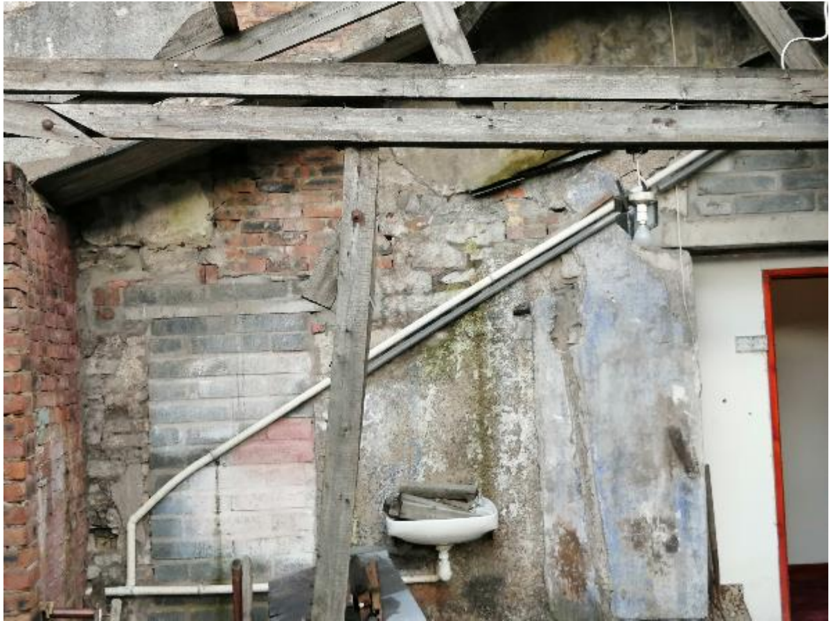
Photo 8 – Missing Render (Rear Wall Elevation)
