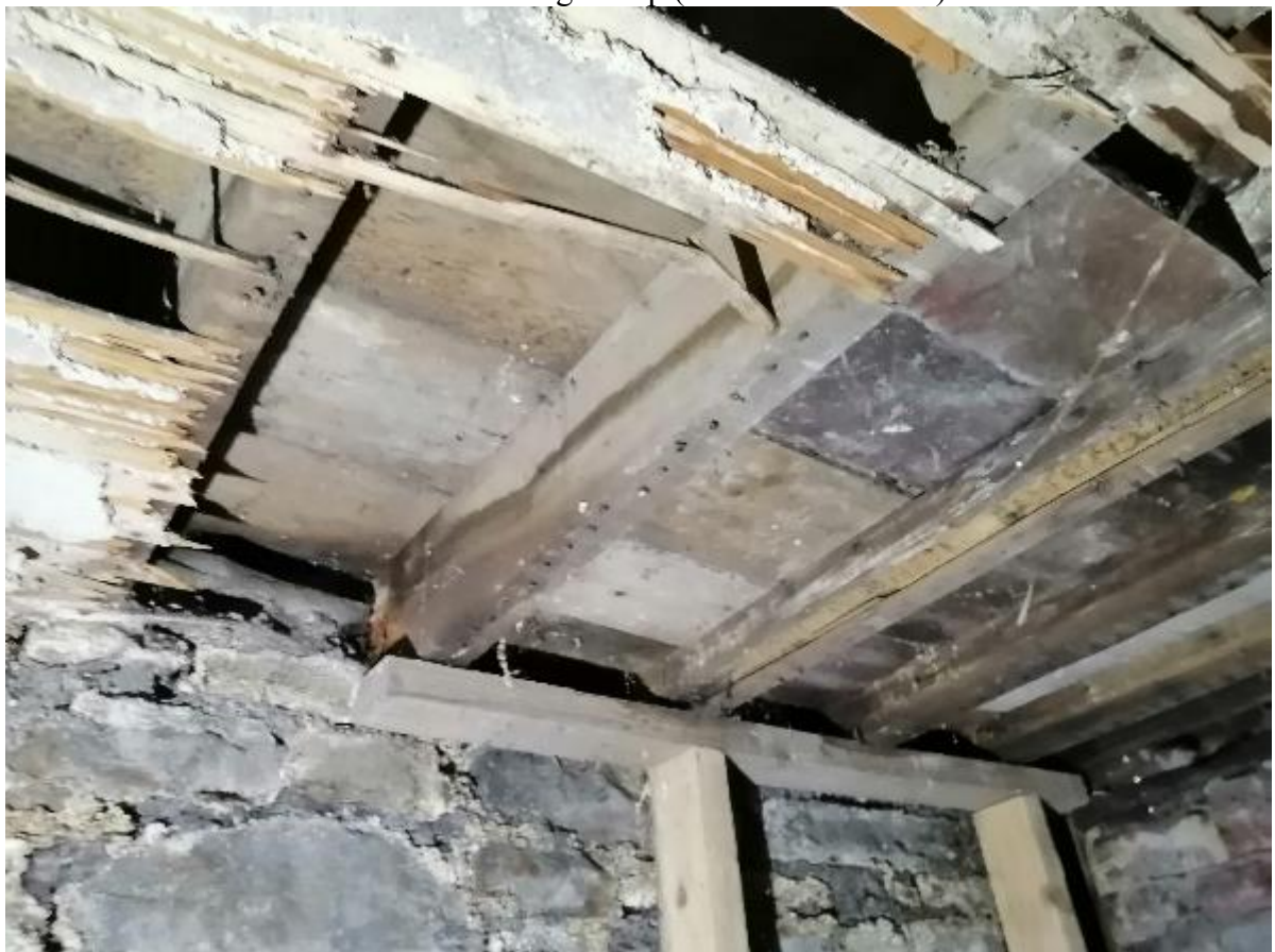
Photo 66 – Damp to Ends of Floor Joists (Basement Room 4)
