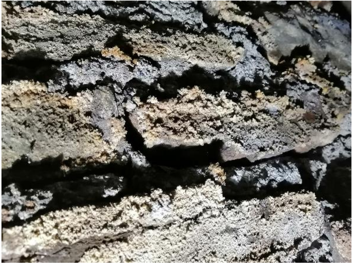
Photo 71 – Penetrating Damp (Basement Room 4)
