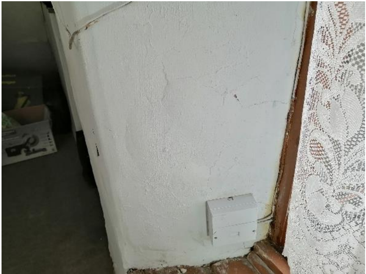
Photo 48 – Detached Plaster (Storeroom)
