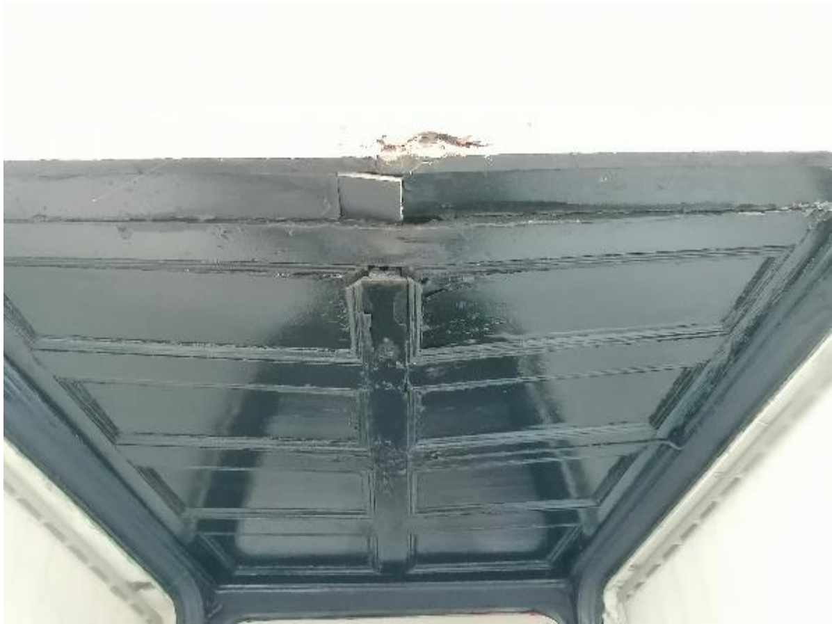
Photo 10 – Bowing to Entrance Ceiling (Front Wall Elevation)
