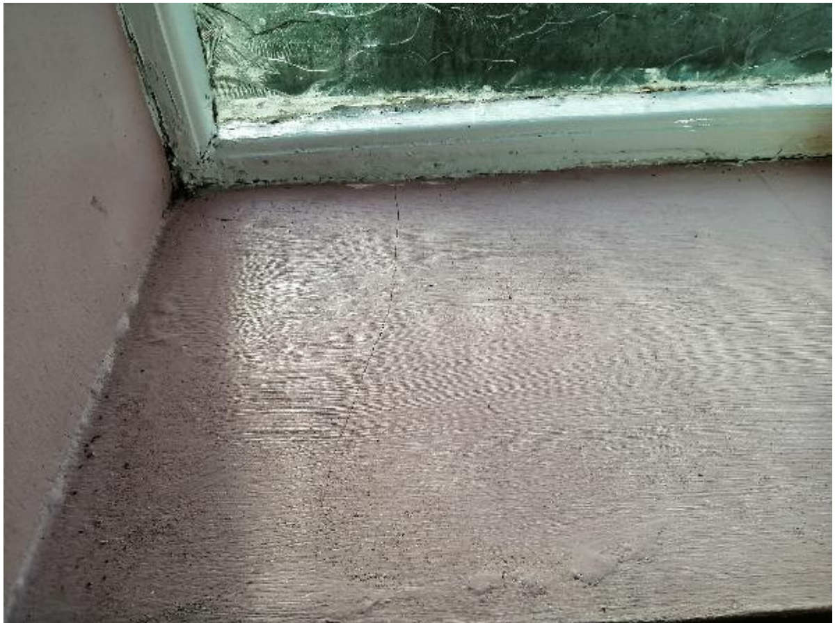
Photo 33 – Crack to Windowsill (Bathroom)
