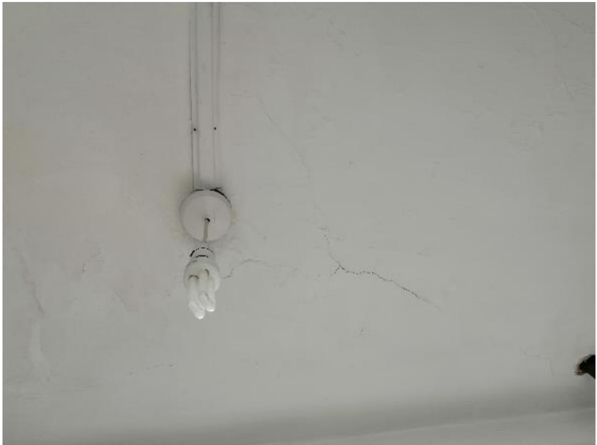
Photo 51 – Ceiling Cracking (Storeroom)
