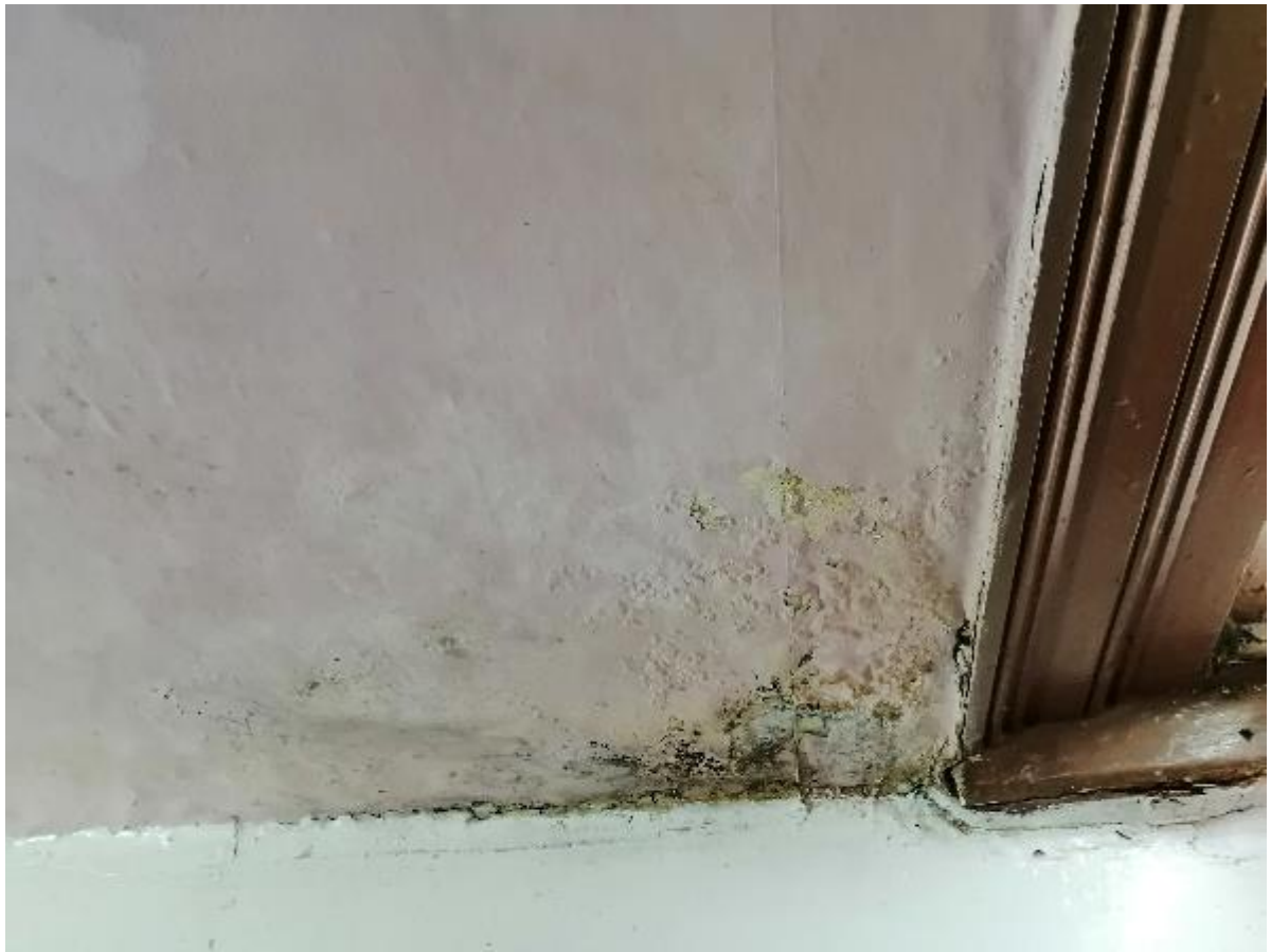
Photo 38 – Penetrating Damp (Bedroom 3)
