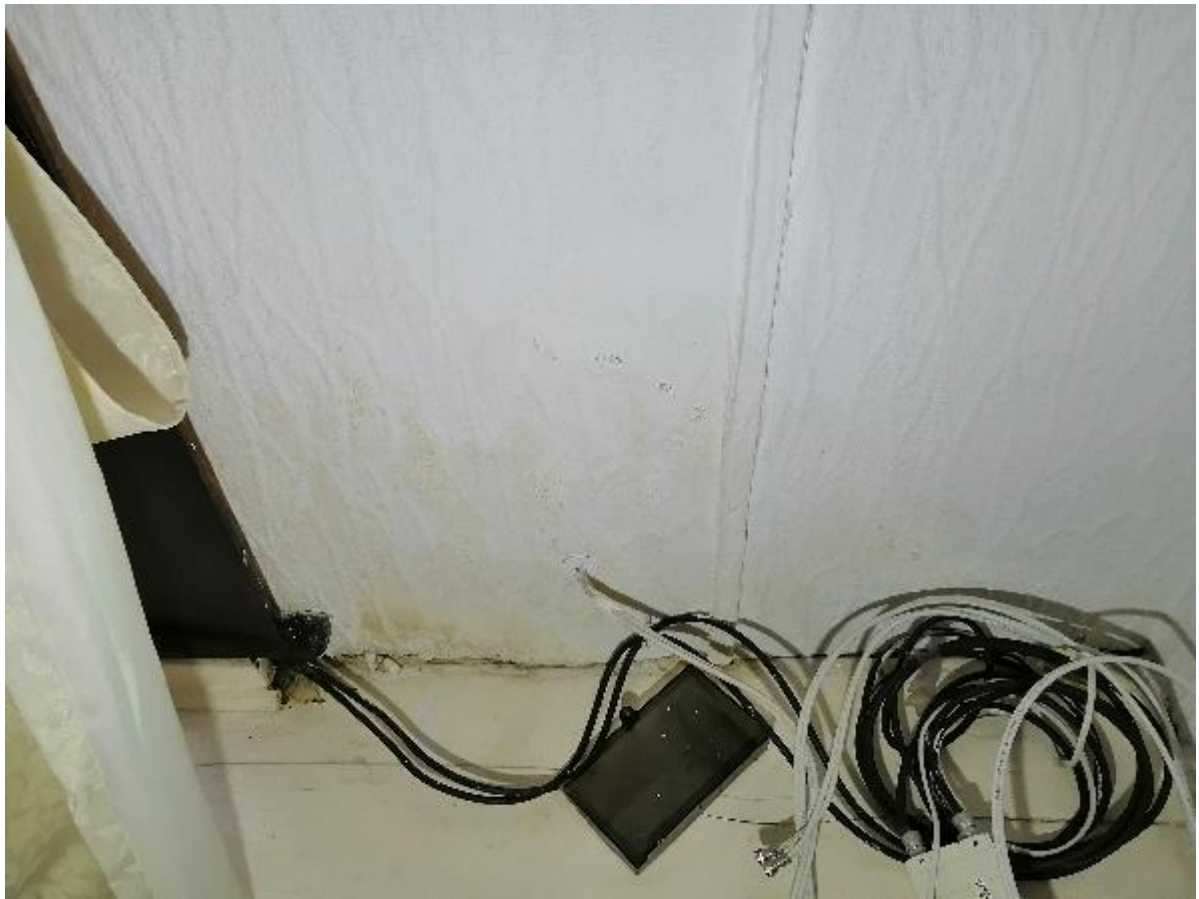
Photo 36 – Penetrating Damp (Bedroom 1)
