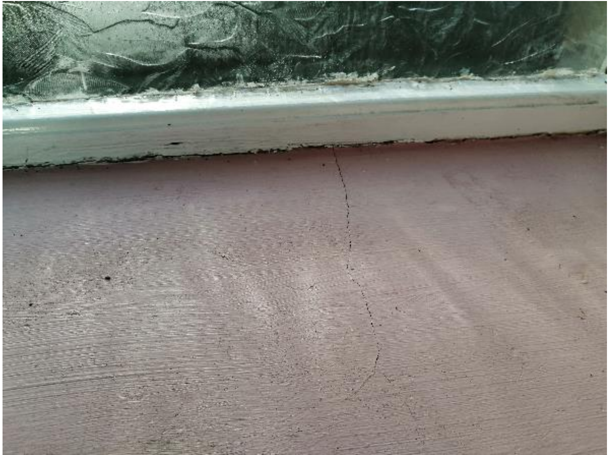
Photo 34 – Crack to Windowsill (Bathroom)
