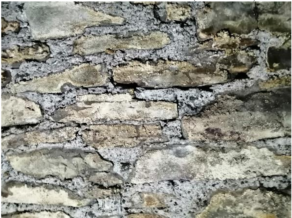
Photo 70 – Penetrating Damp (Basement Room 4)
