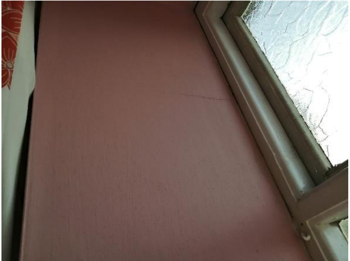
Photo 30 – Wall Plaster Crack (Bathroom)
