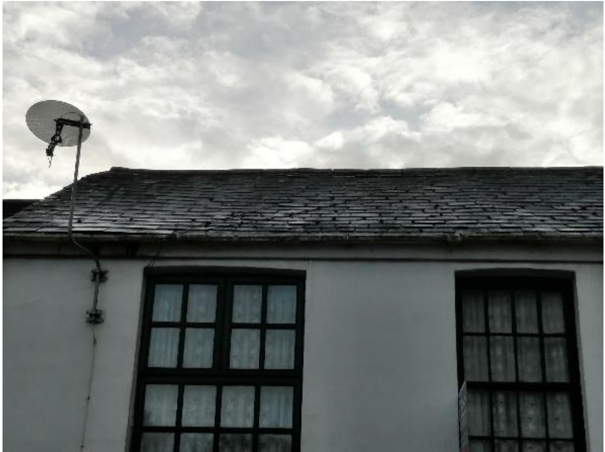
Photo 3 – Bowing to Roof (Front Roof Profile)
