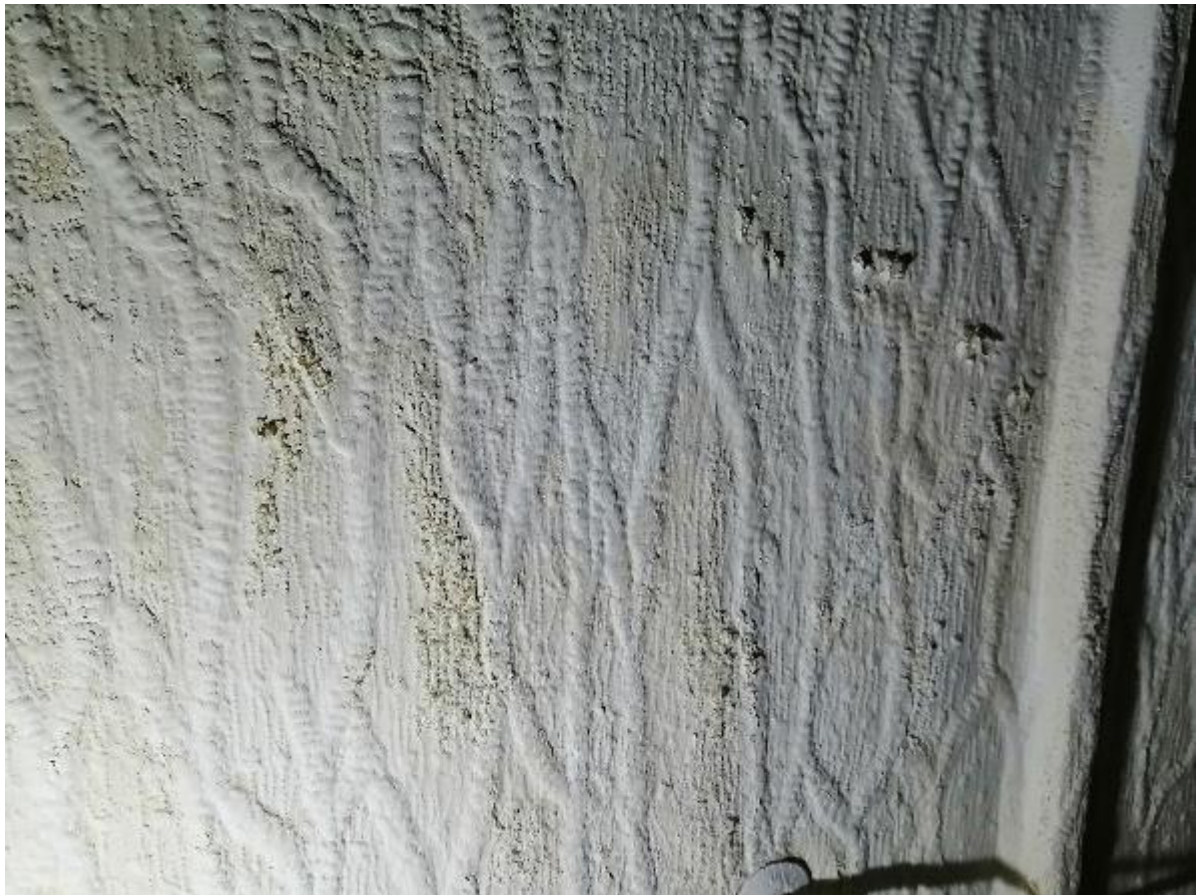
Photo 37 – Penetrating Damp (Bedroom 1)
