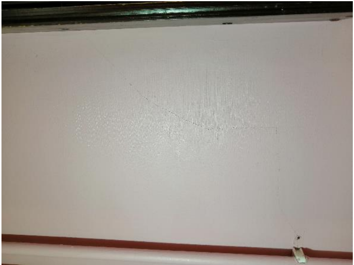
Photo 28 – Wall Plaster Crack (Bathroom)
