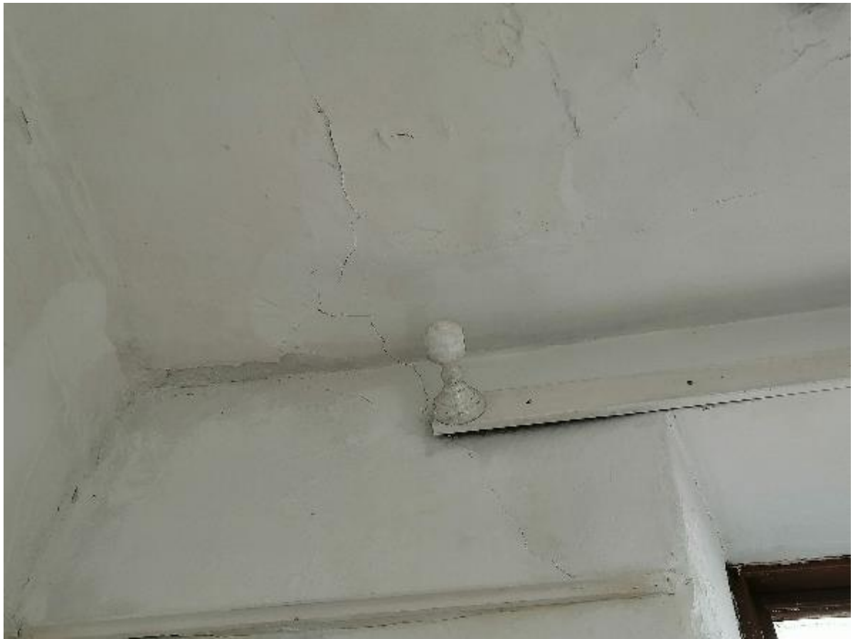
Photo 50 – Cracking to Wall and Ceiling (Storeroom)
