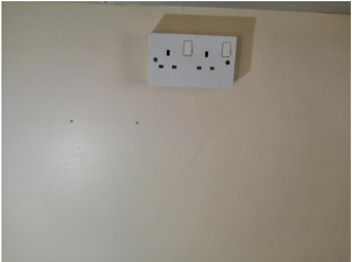
Photo 25 – Wall Plaster Cracking (Kitchen)
