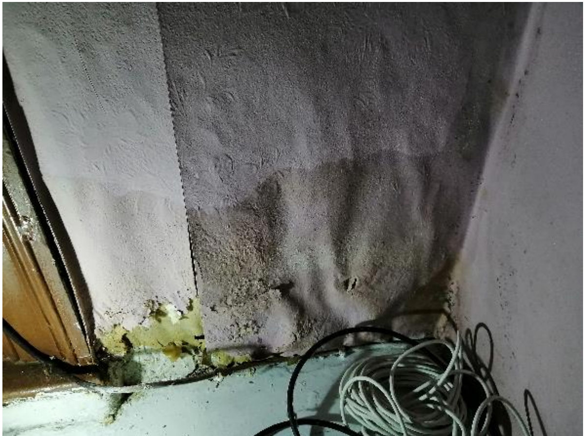
Photo 39 – Penetrating Damp (Bedroom 3)
