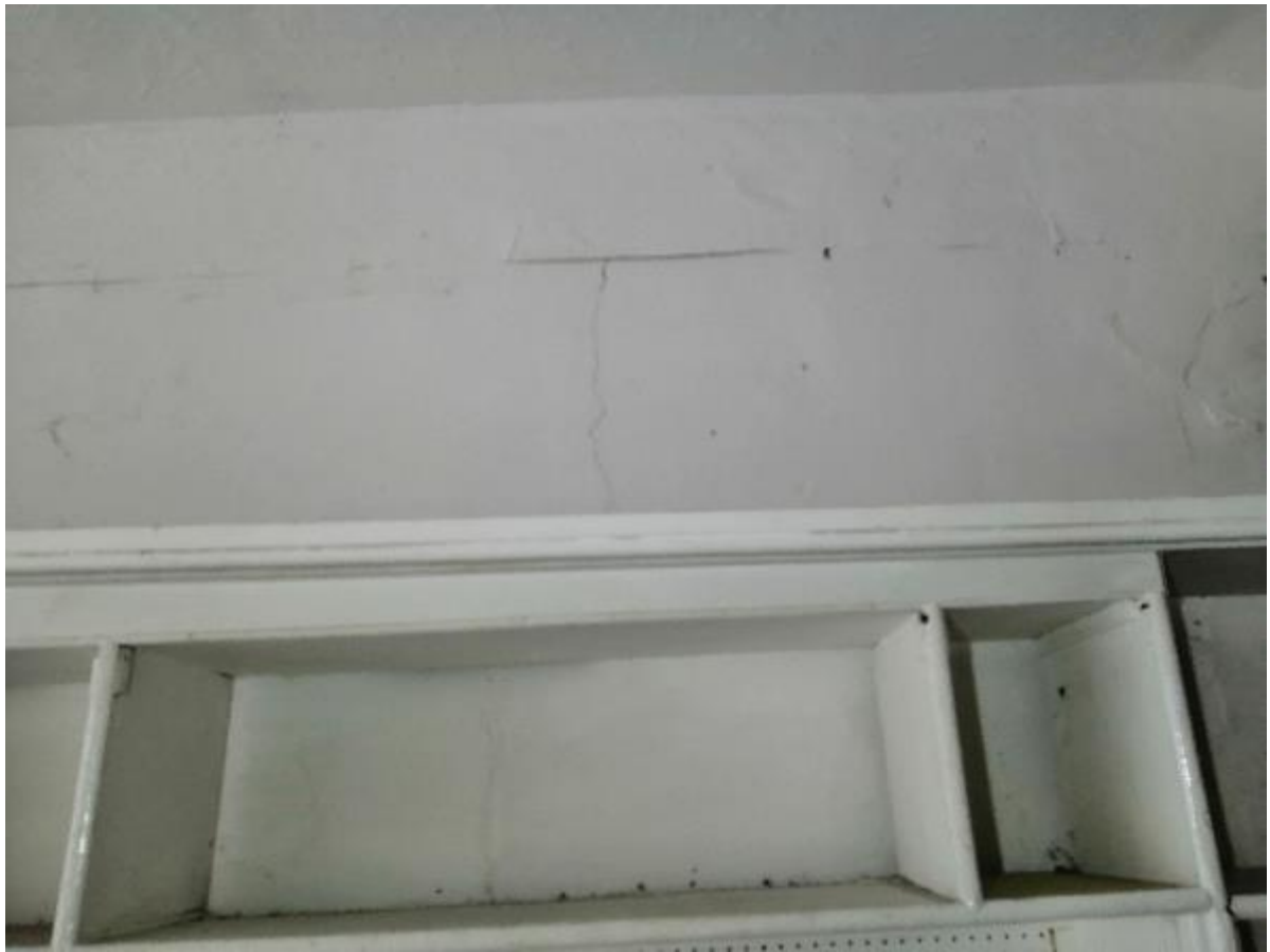
Photo 52 – Wall Plaster Crack (Living Room 2)
