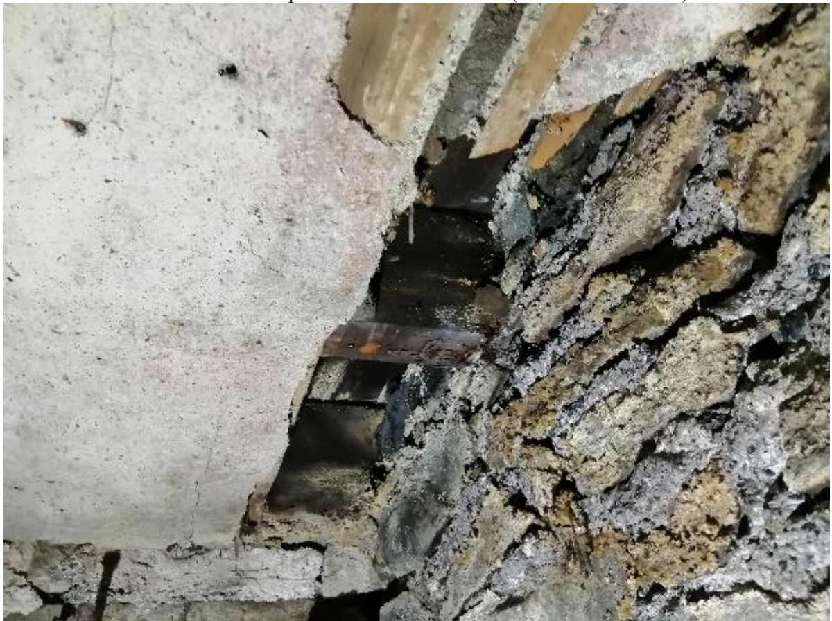
Photo 68 – Damp to Ends of Floor Joists (Basement Room 4)
