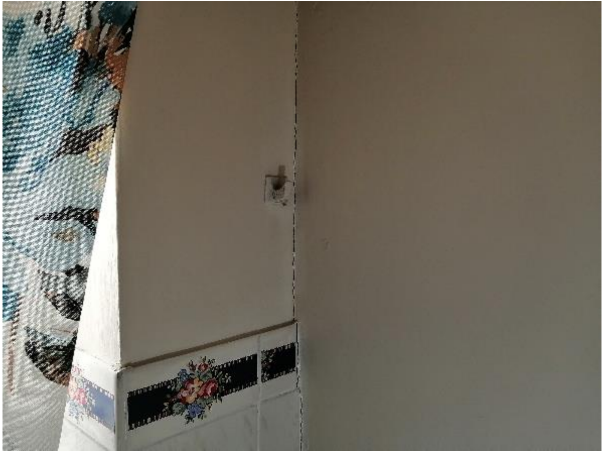
Photo 22 – Cracking to Edge of Studwork Wall (Kitchen)
