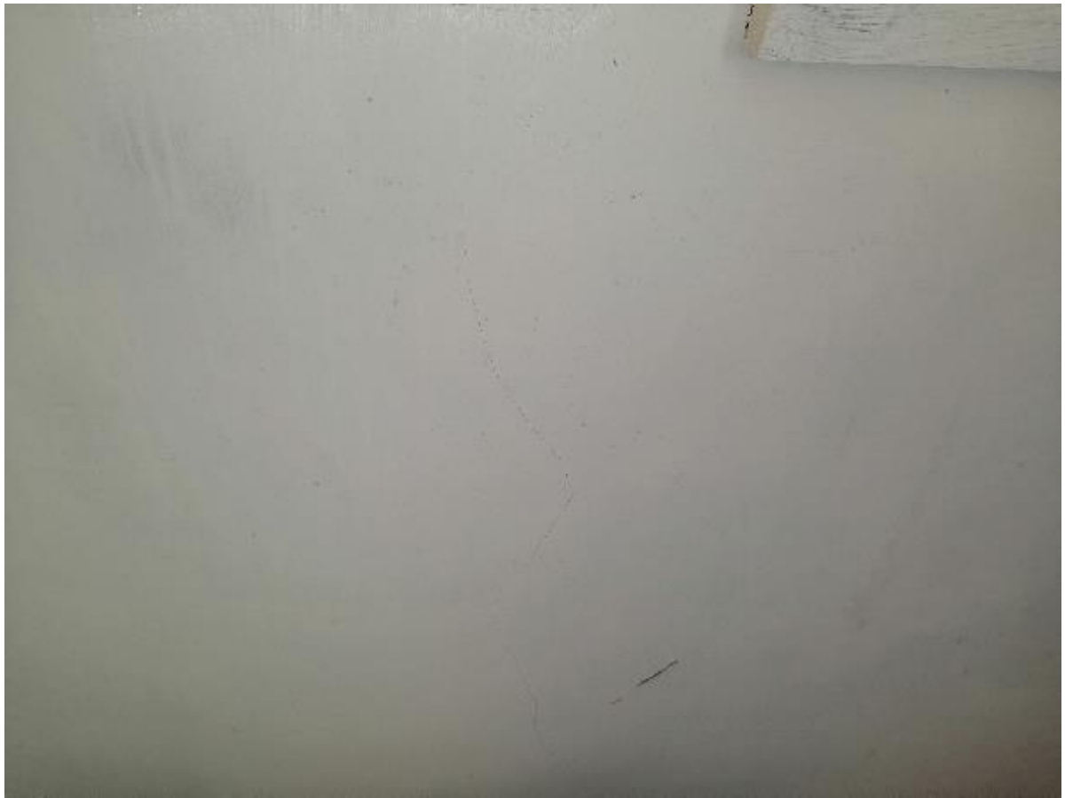
Photo 24 – Wall Plaster Cracking (Kitchen)
