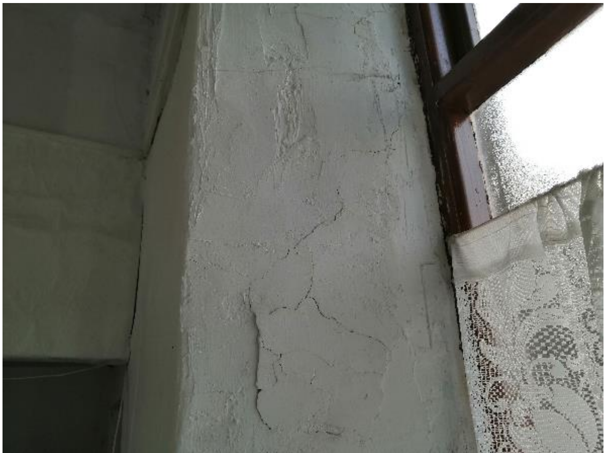
Photo 49 – Cracked and Detached Plaster (Storeroom)
