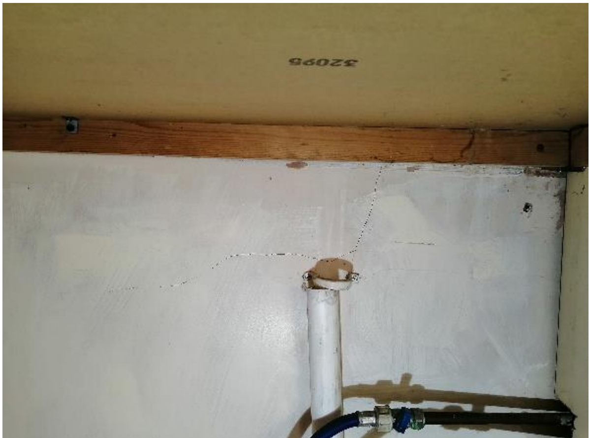
Photo 23 – Wall Plaster Cracking (Kitchen)
