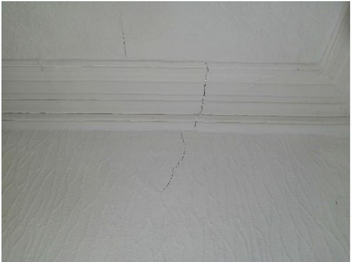
Photo 27 – Cracking to Studwork Wall (Bedroom 1)
