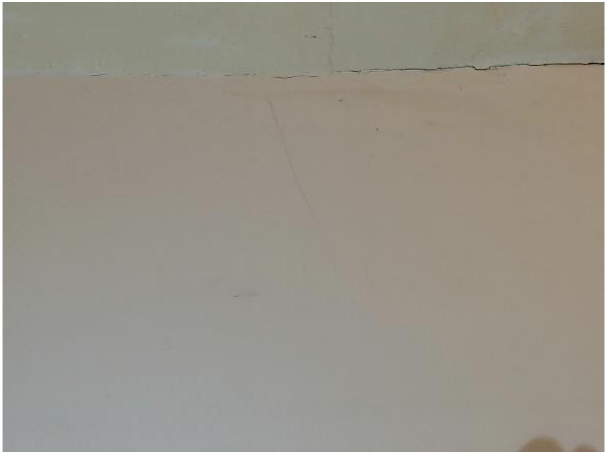
Photo 47 – Cracking to Studwork Wall (Base of Stairs)
