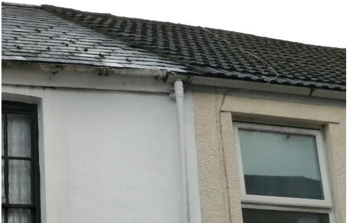
Photo 4 – Defective Guttering (Front Roof Profile)
