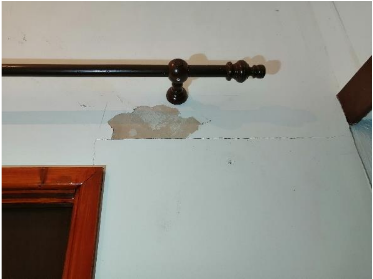
Photo 46 – Cracking to Studwork Wall (Base of Stairs)
