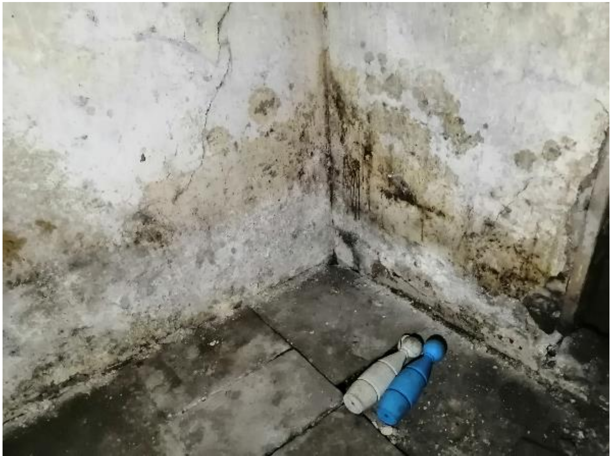
Photo 65 – Rising Damp (Basement Room 3)
