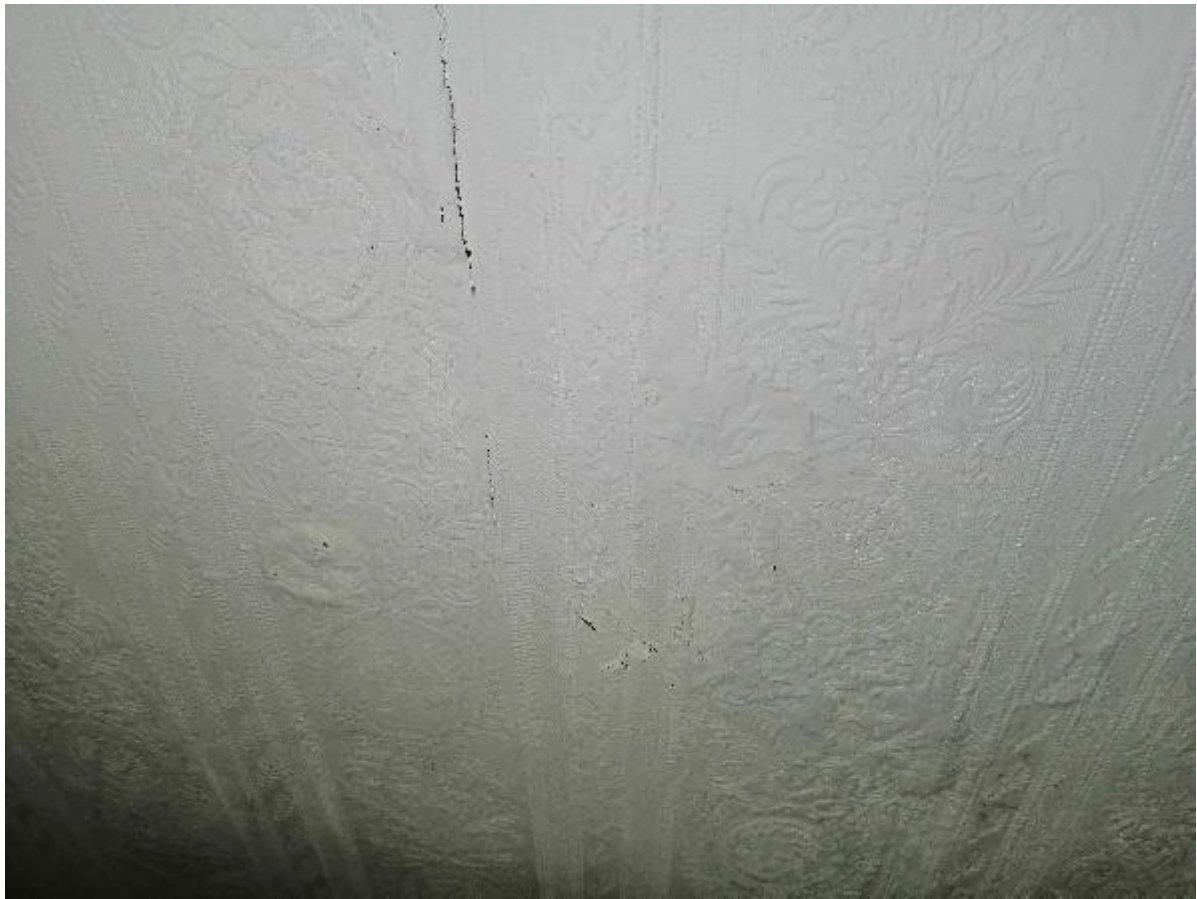
Photo 40 – Penetrating Damp (Landing)
