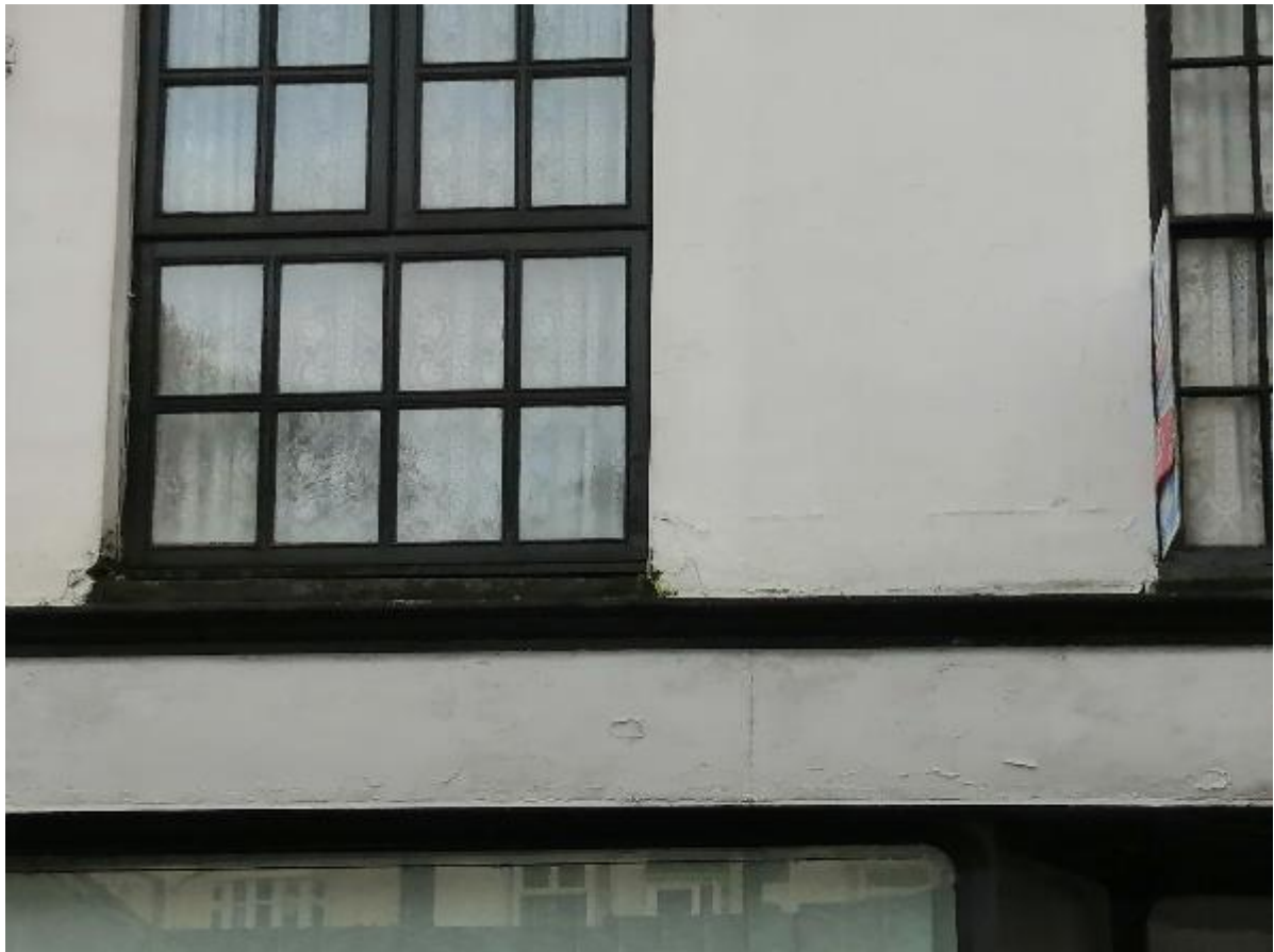
Photo 9 – Render Cracking to Both Sides of the Window (Front Wall Elevation)
