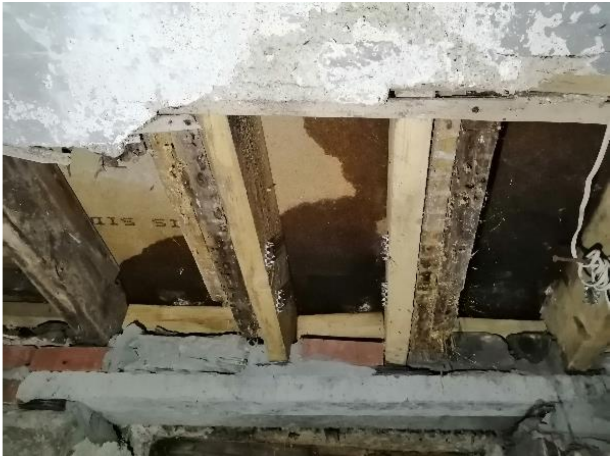
Photo 64 – Damp to Floorboards and Joists (Basement Room 2)
