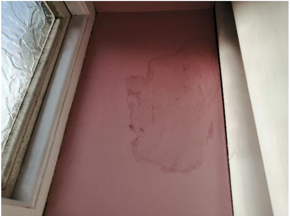
Photo 31 – Wall Plaster Crack (Bathroom)
