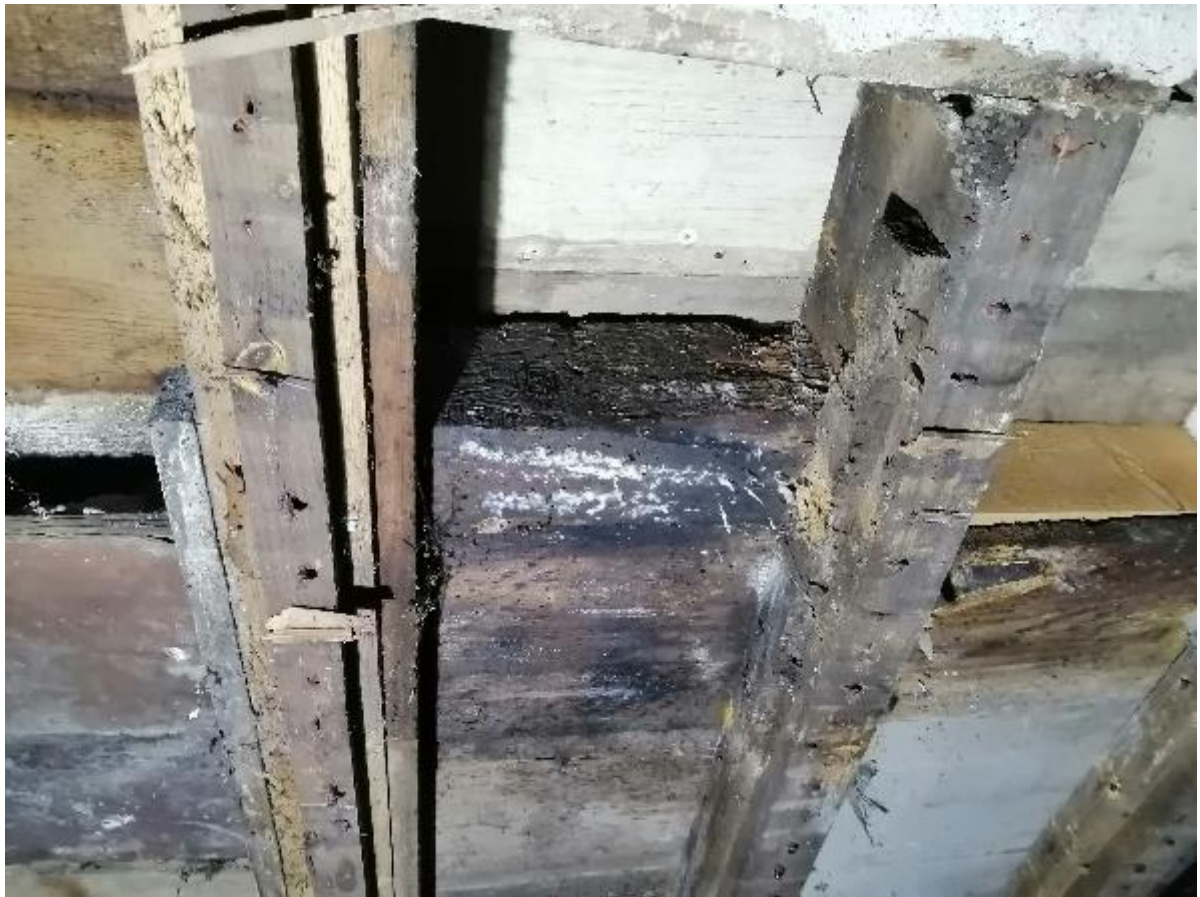
Photo 69 – Rot and Mould Growth to Floor Joists (Basement Room 4)
