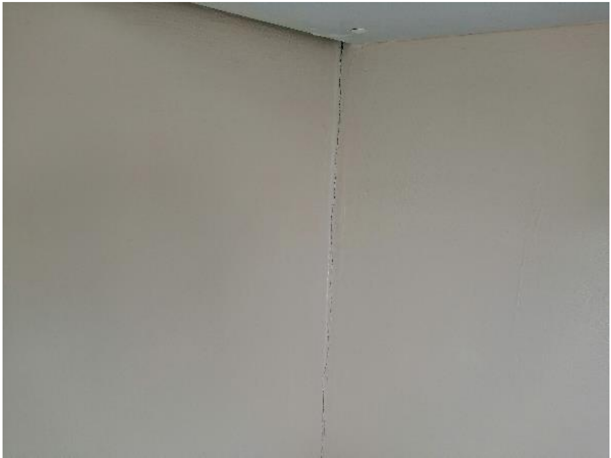
Photo 26 – Cracking to Edge of Studwork Wall (Kitchen)
