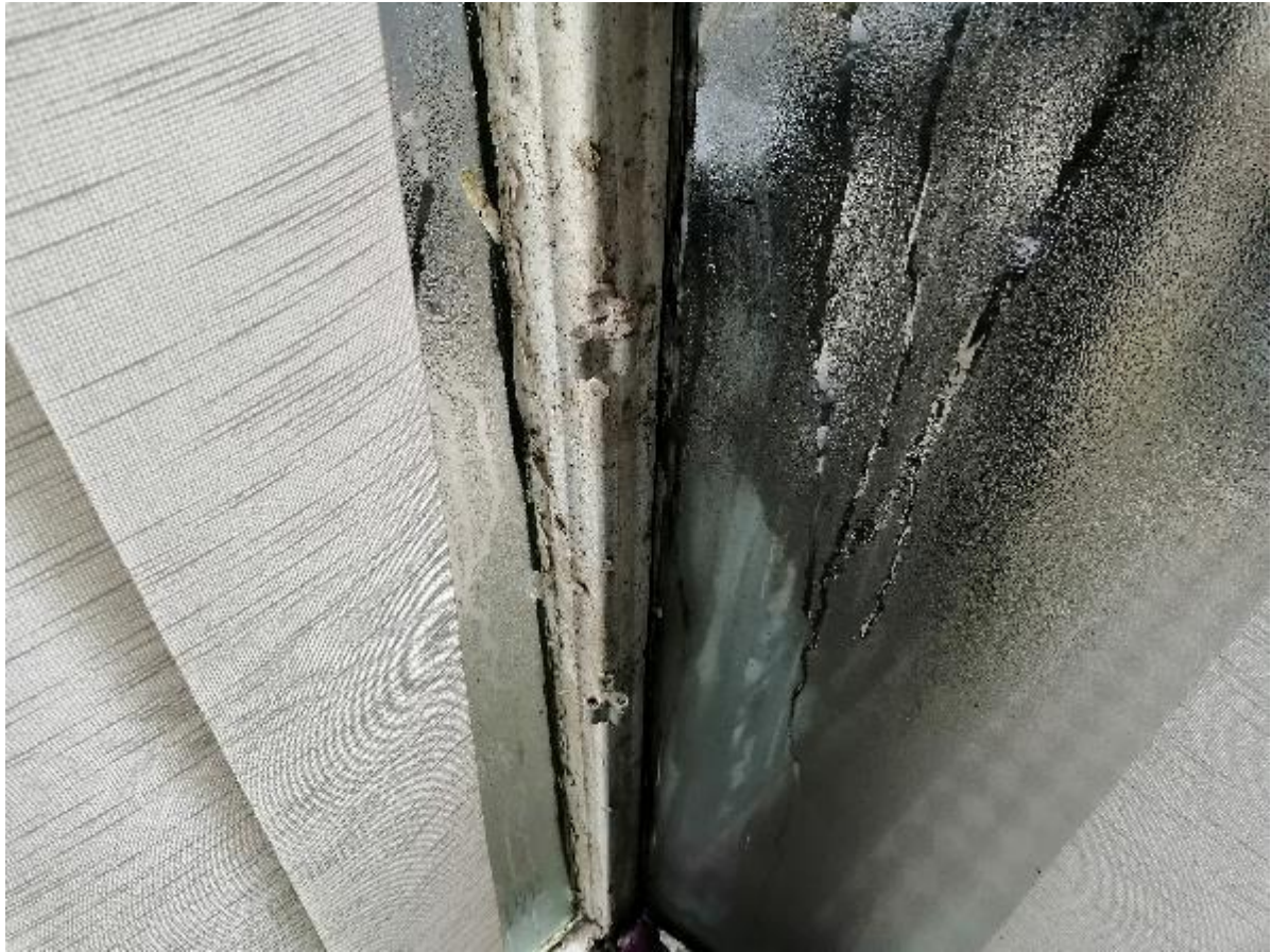
Photo 54 – Condensation Damp (Living Room 1)
