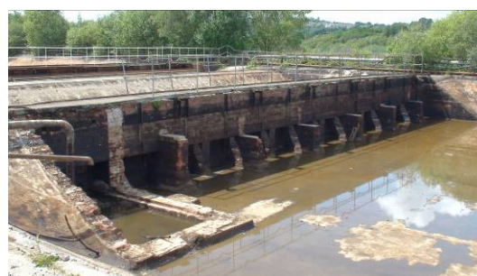
Example of brick structures – note hydrocarbon staining 29 June 2011
