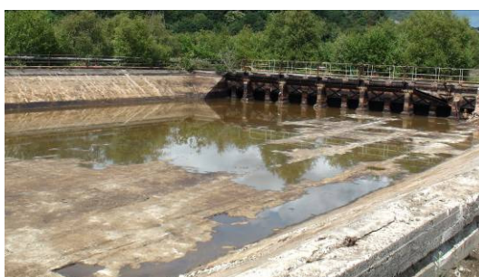
Chamber following sludge removal – note hydrocarbon staining on sides 29 June 2011
