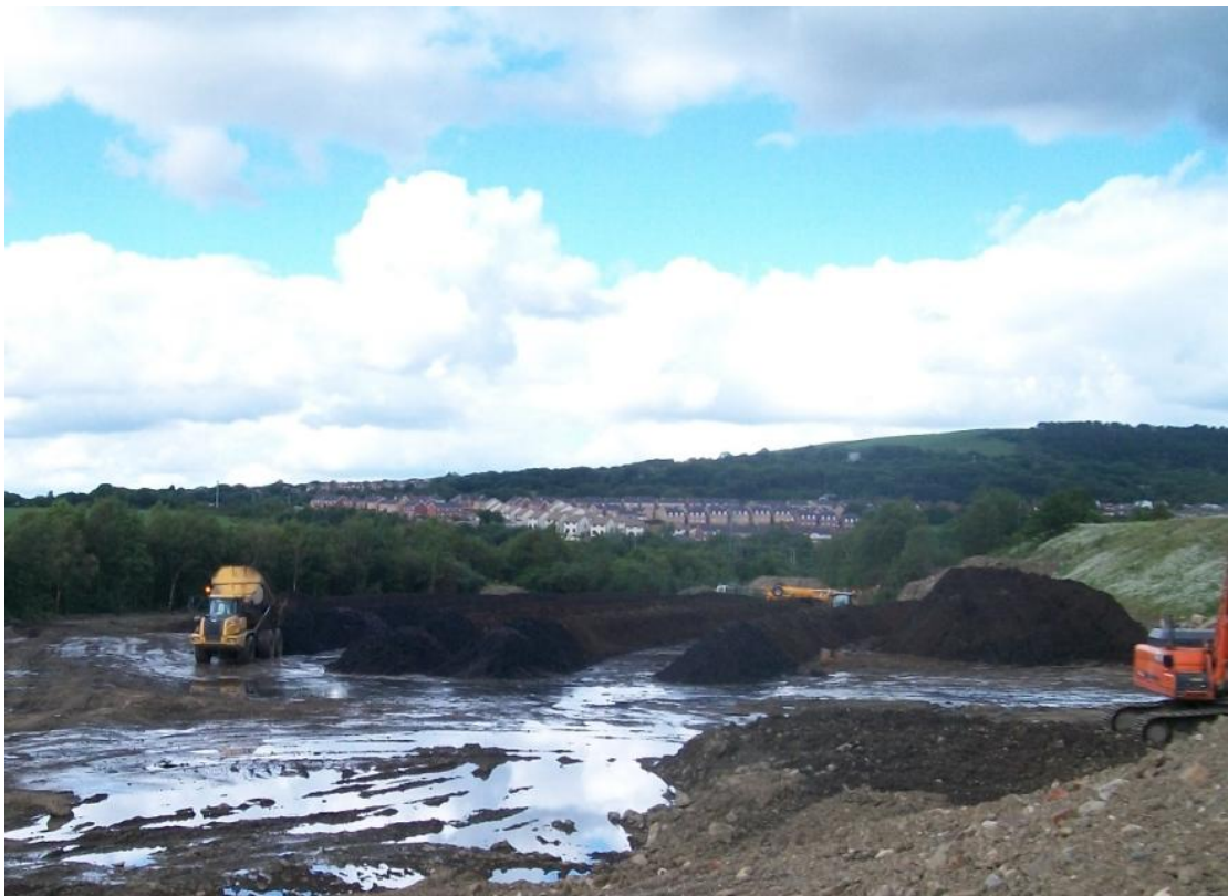
Photograph 6: Hydrocarbon impacted material on the Treatment pad
