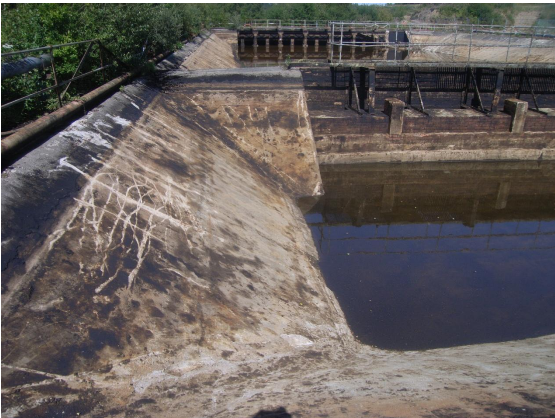
Photograph 8: Chamber 3 – Post remediation some light staining on concrete
