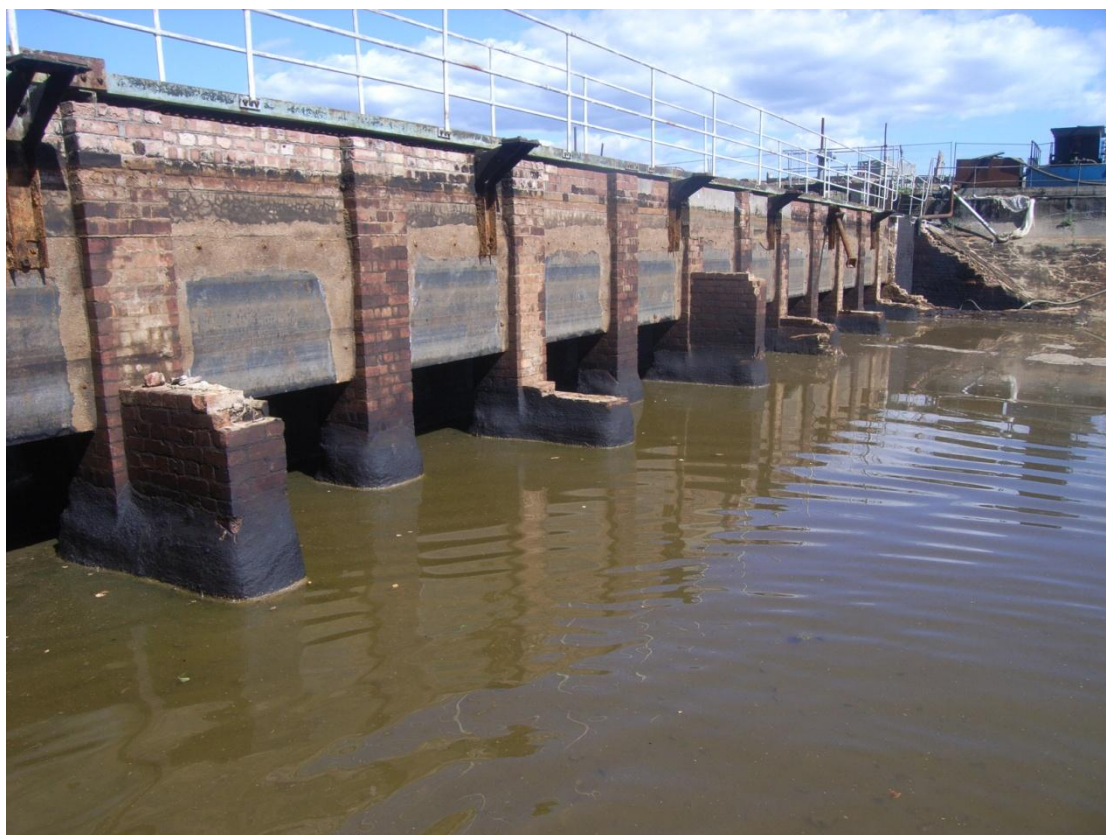
Photograph 6: Chamber 2 - Post remediation staining on lower brickwork
