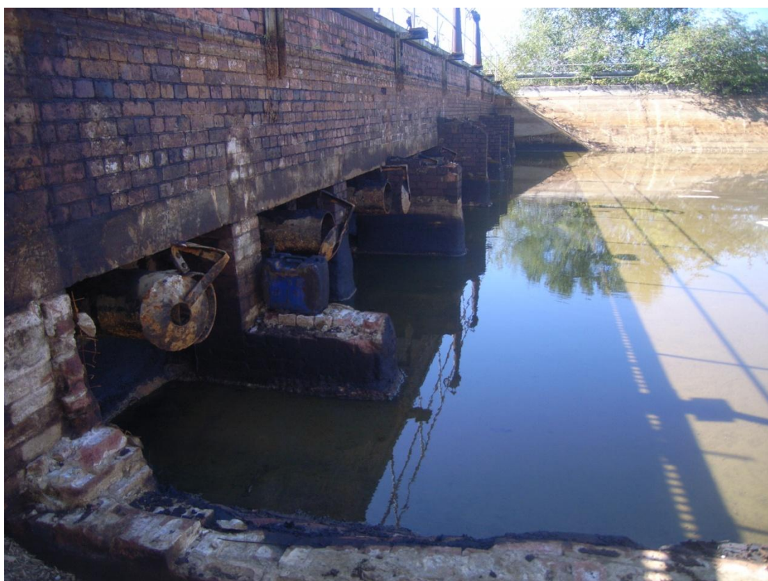
Photograph 4. Chamber 2 – Post remediation some staining on brickwork
