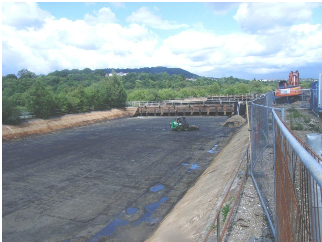
Photograph 3. Chamber 2 – Scrubbing unit in operation following sludge removal
