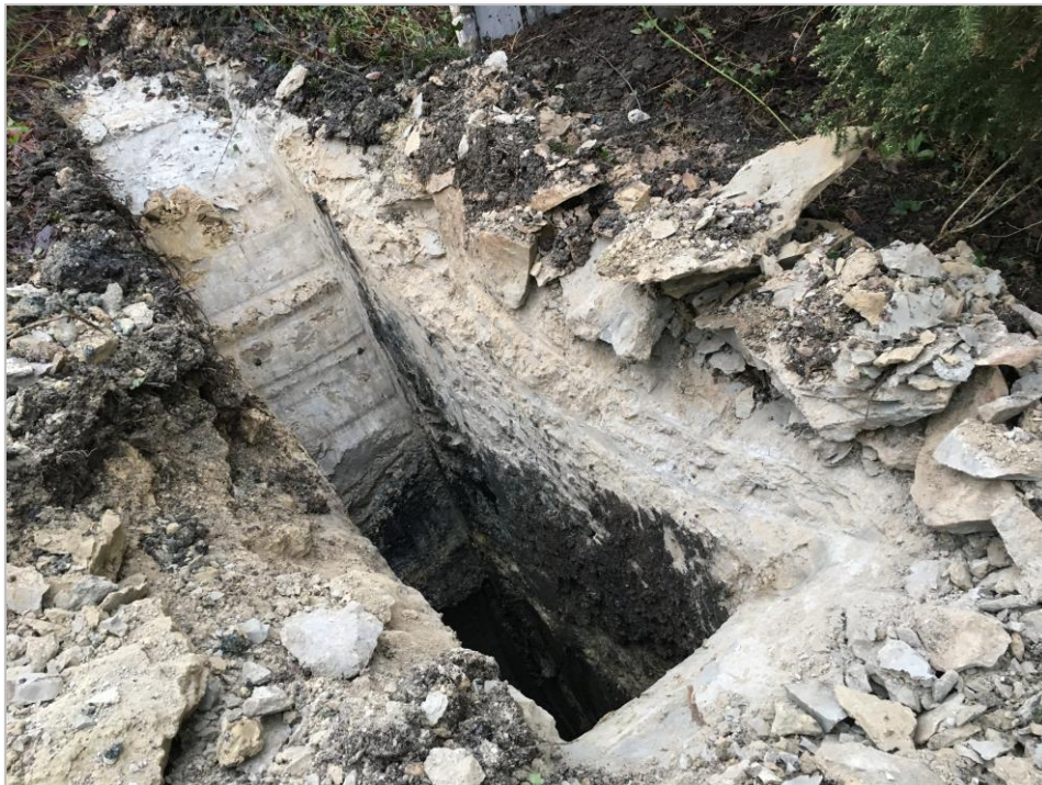
Photograph 18: TP10 excavation with possible china clay used in refinery processes and disposed of in the Tip
