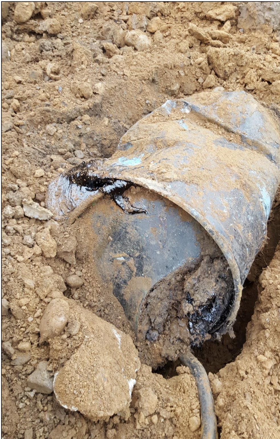
Photograph 3 TPE2740 – Excavation of largely intact barrel of free product from trial pit.
