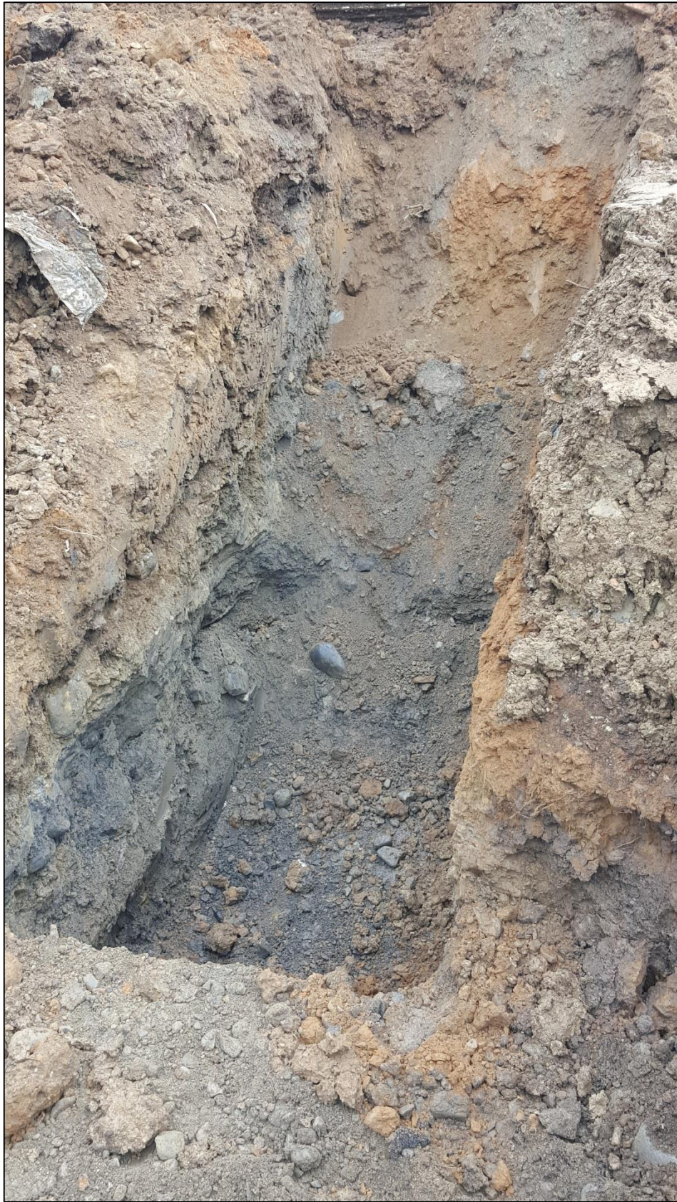
Photograph 2 TPE2739 – Minor free product at base of trial pit
