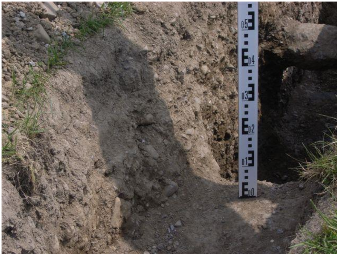
Photograph 12: Depth to concrete obstruction
