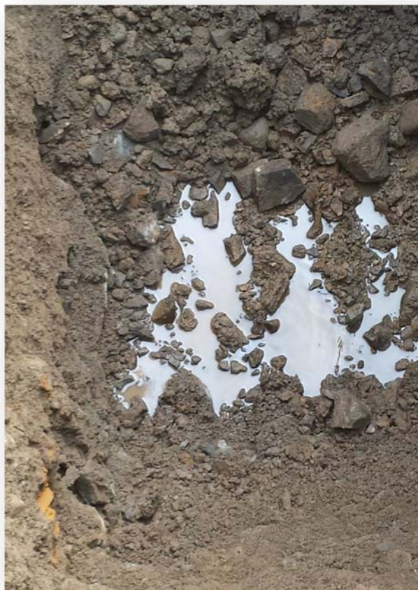
Photo 2: Groundwater seepage in the base of the excavation (reflection of the sky gives a shimmery appearance)
