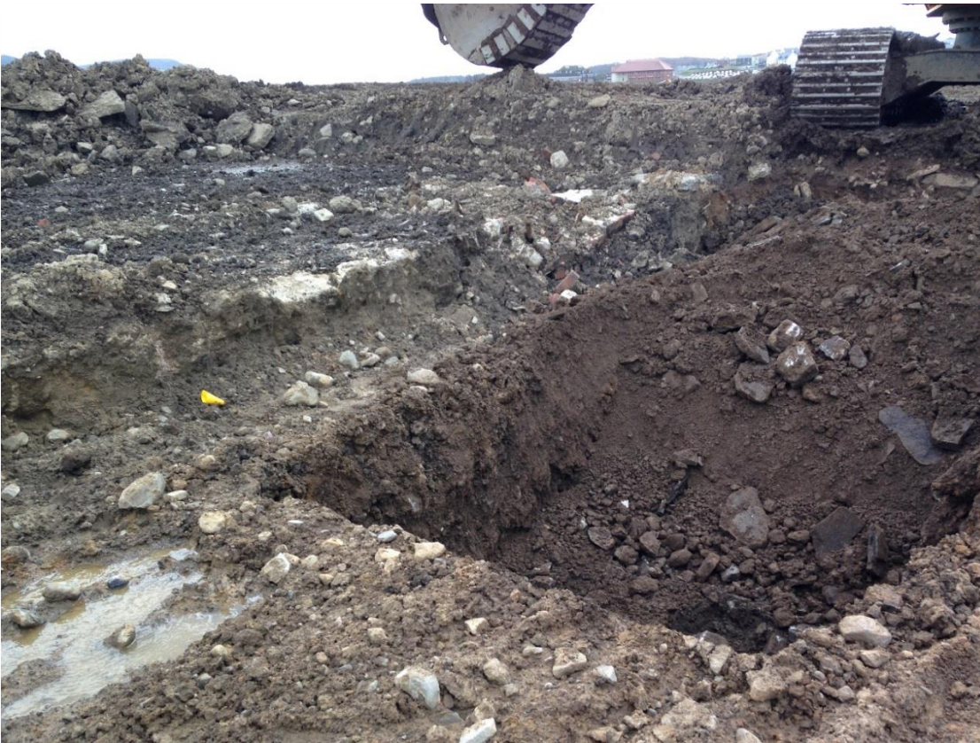
Photograph 4 NSW347 - investigation into VO 5,0 recorded during ground investigation. No free product encountered.
