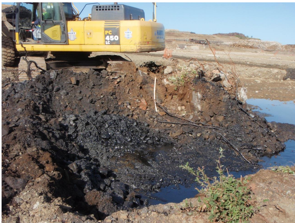
Photograph 12: Localised free product identified during the works
