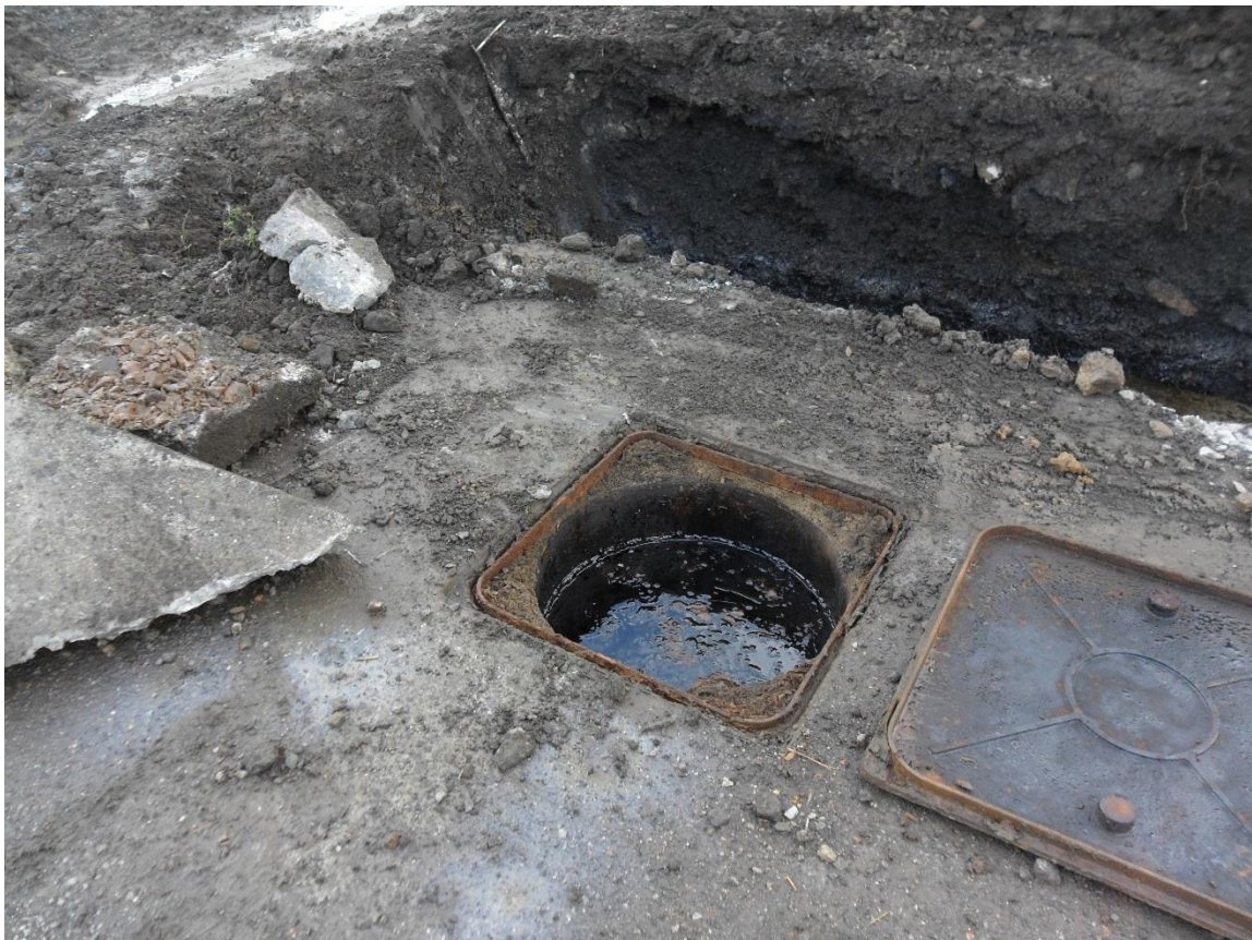
6) Recovery manhole exhibiting product and wax in the chamber
