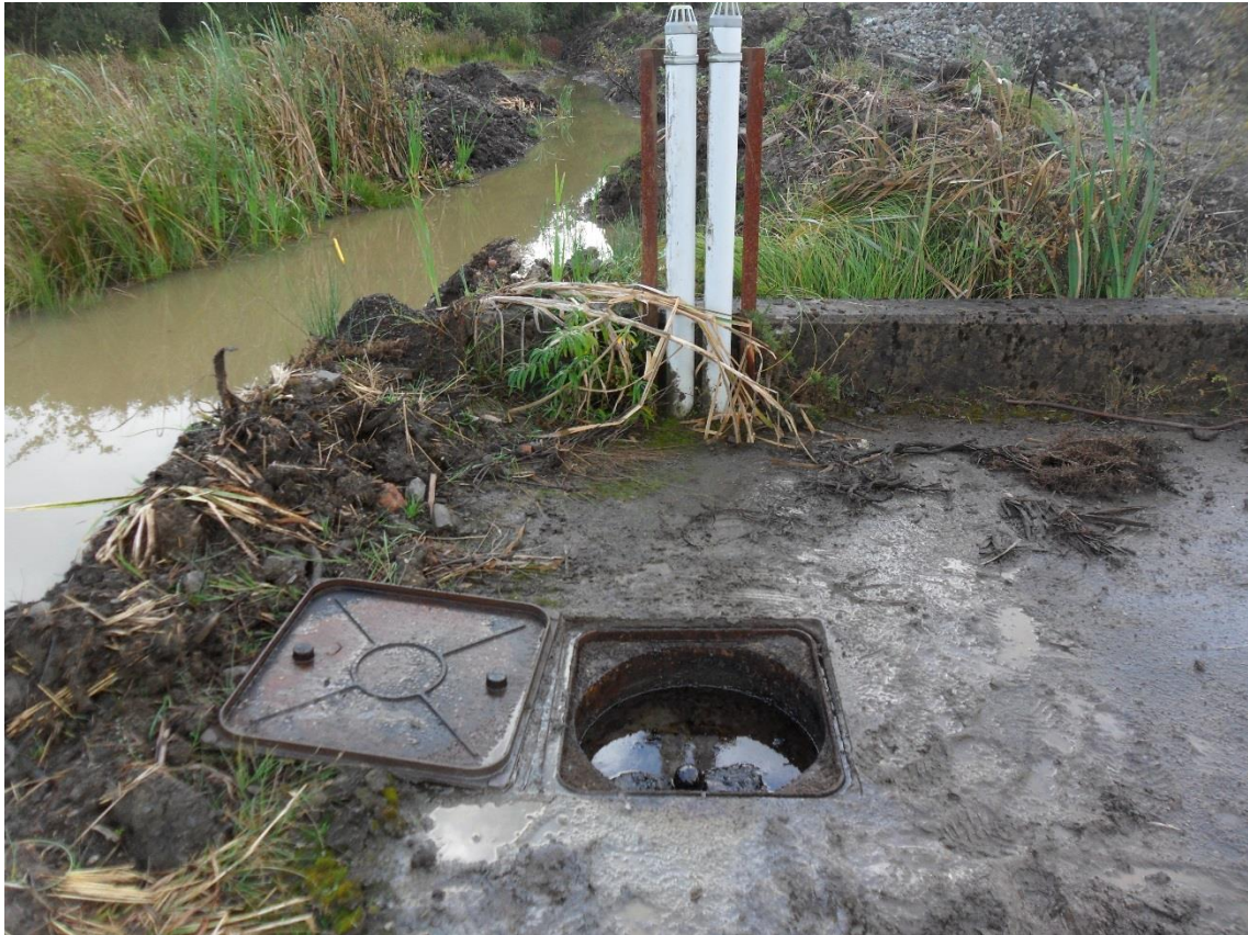
5) Recovery manhole exhibiting product and wax in the chamber
