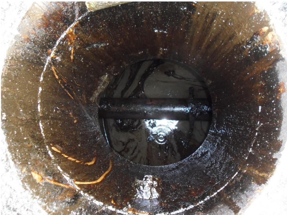
8) Photo looking in to the separator chamber. Free product on grey basal silts.
