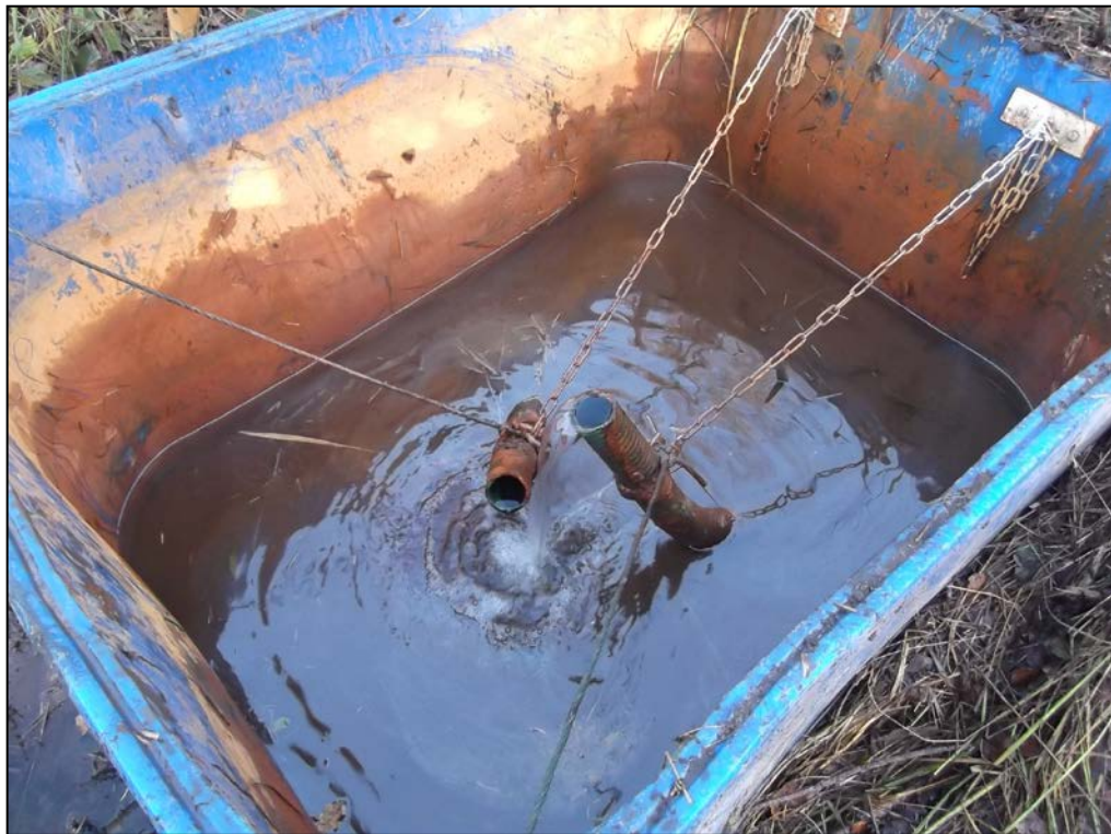
Photographs 4 and 5 – Operational outlet pipe from reed pond into separator
