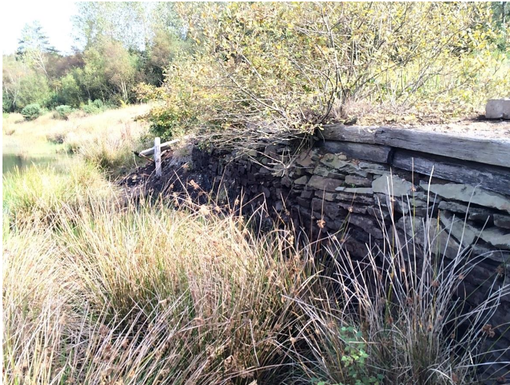
Photo 2 – September 2015, area of residual hydrocarbon staining adjacent stone wall
