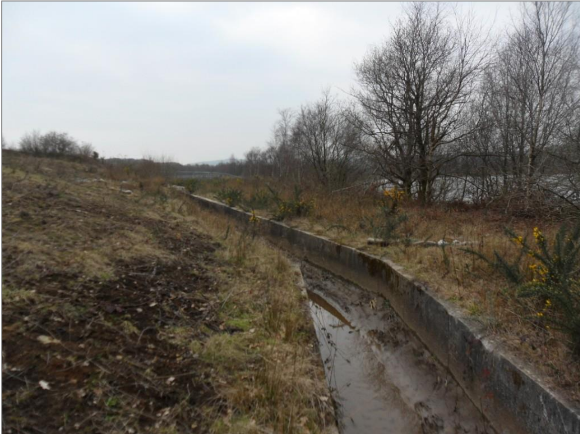
Photograph 18: Operational concrete drainage channel taking water from NSR API separators.
