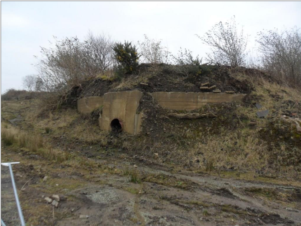
Photograph 23: Base of the former biological filter which contains significant amounts of plastic objects used within the filtering process.
