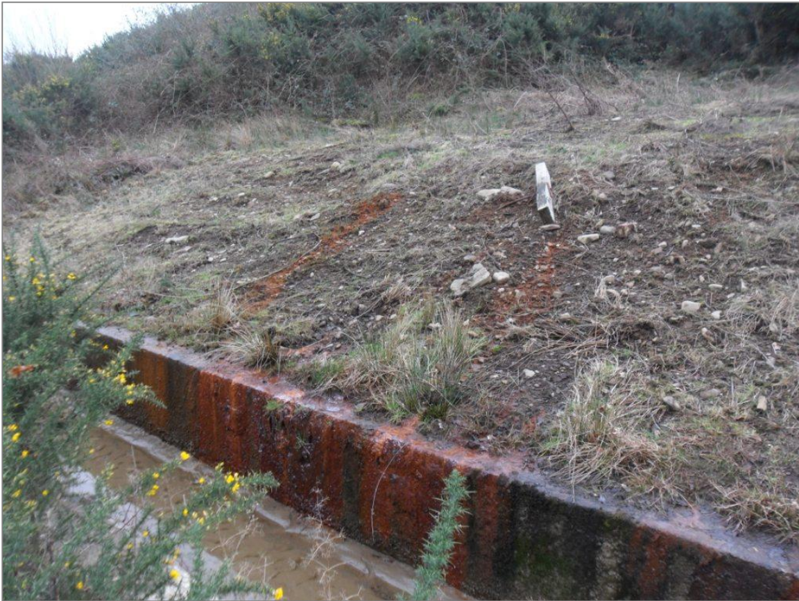
Photograph 19: Ochreous discharge into the concrete drainage channel.
