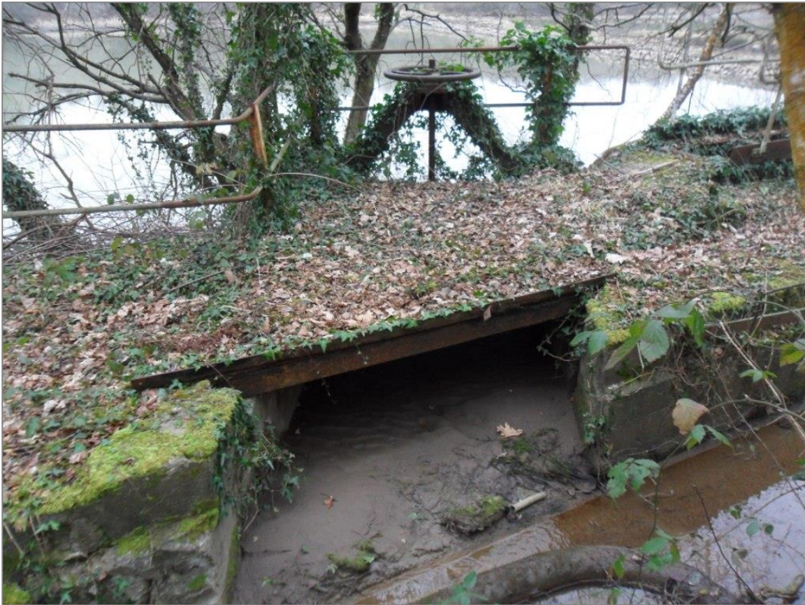
Photograph 13: Exceedance flow sluice gate.
