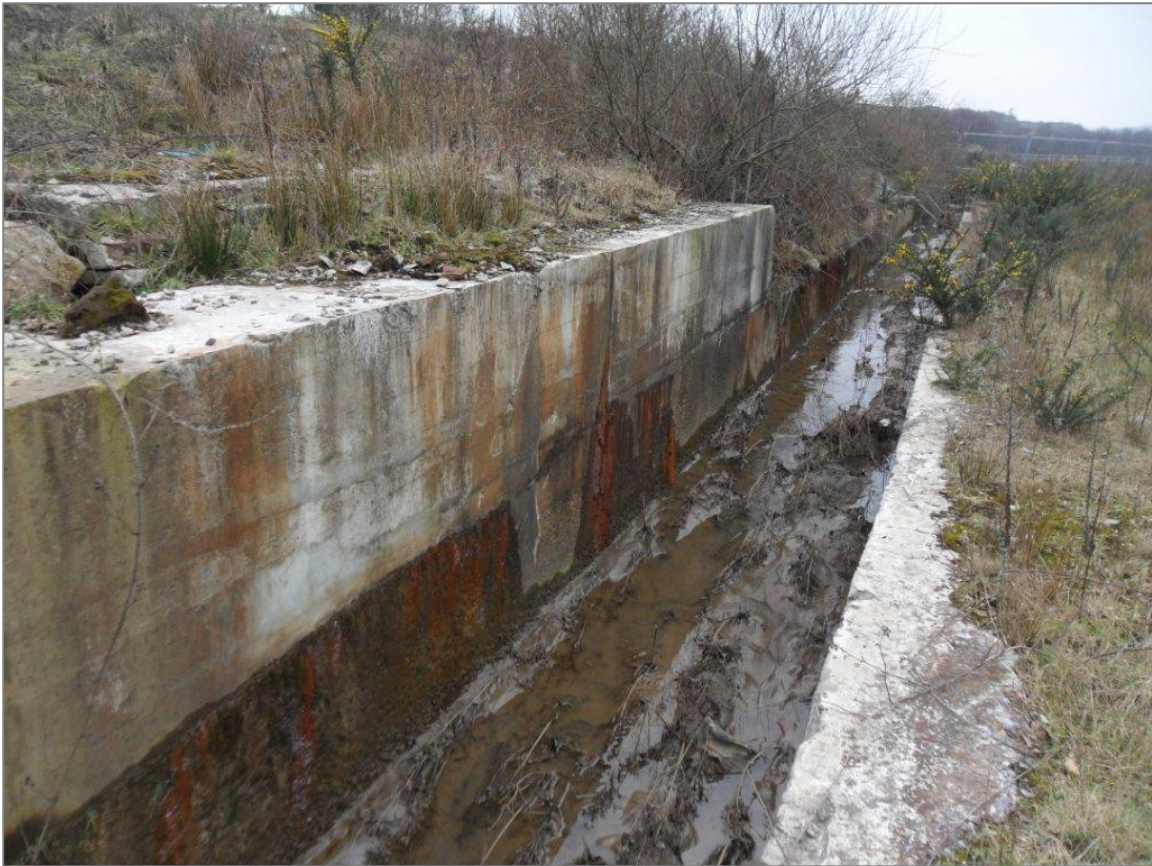
Photograph 21: Ochreous discharge into the concrete drainage channel from a thick concrete structure. Photo viewing towards the south west.
