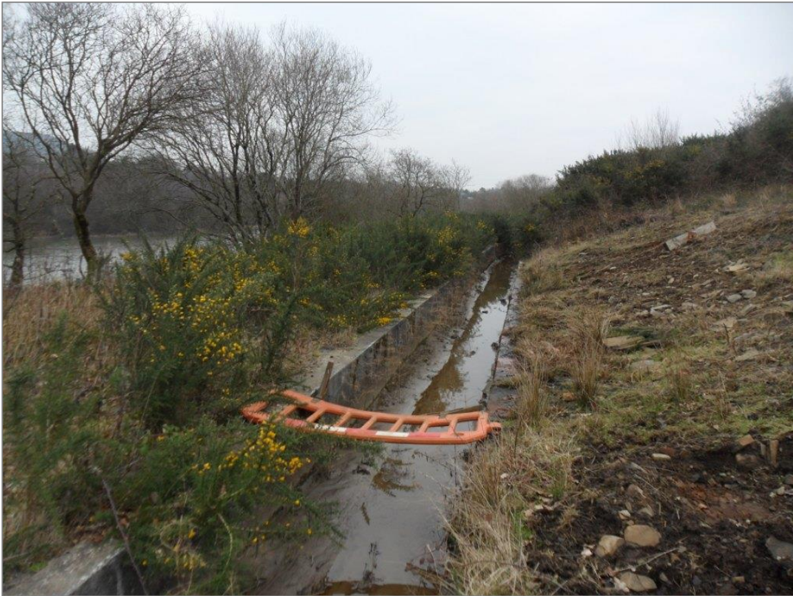
Photograph 17: Operational concrete drainage channel taking water from NSR API separators.
