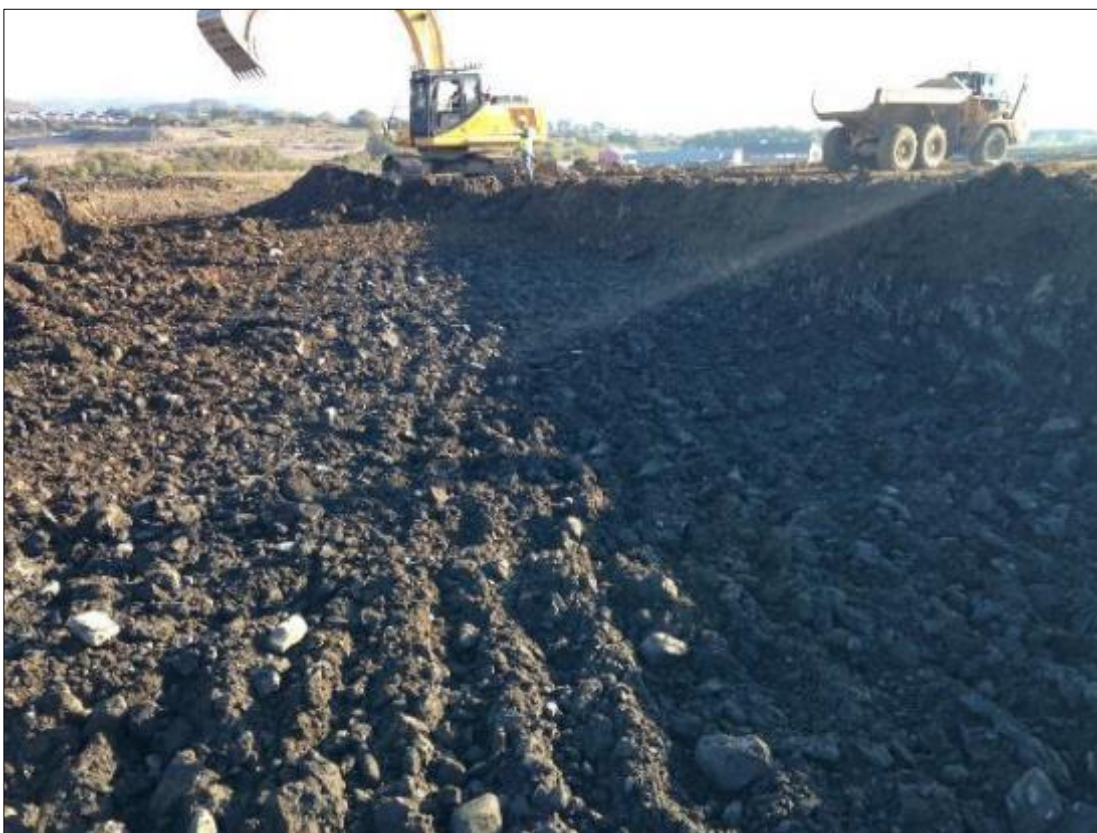
29) Underlying surface following removal of the visual and olfactory failures. Comprising predominantly natural soil (clayey sandy gravel/gravelly sandy clay)
