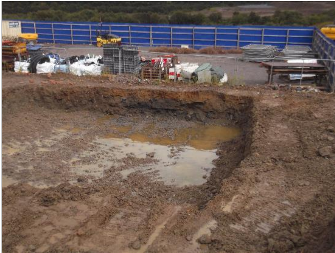
32) Looking north over IP4076 RBSL failure excavation. Pit was extended to 10m by 10m by 1.5m bgl.
