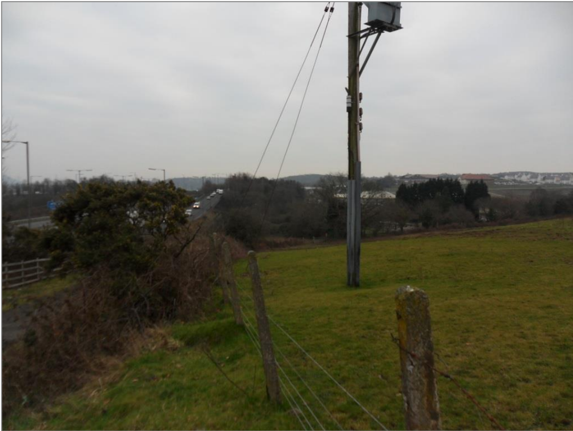
Photograph 3: Pole mounted transformer on the north site fields area..
