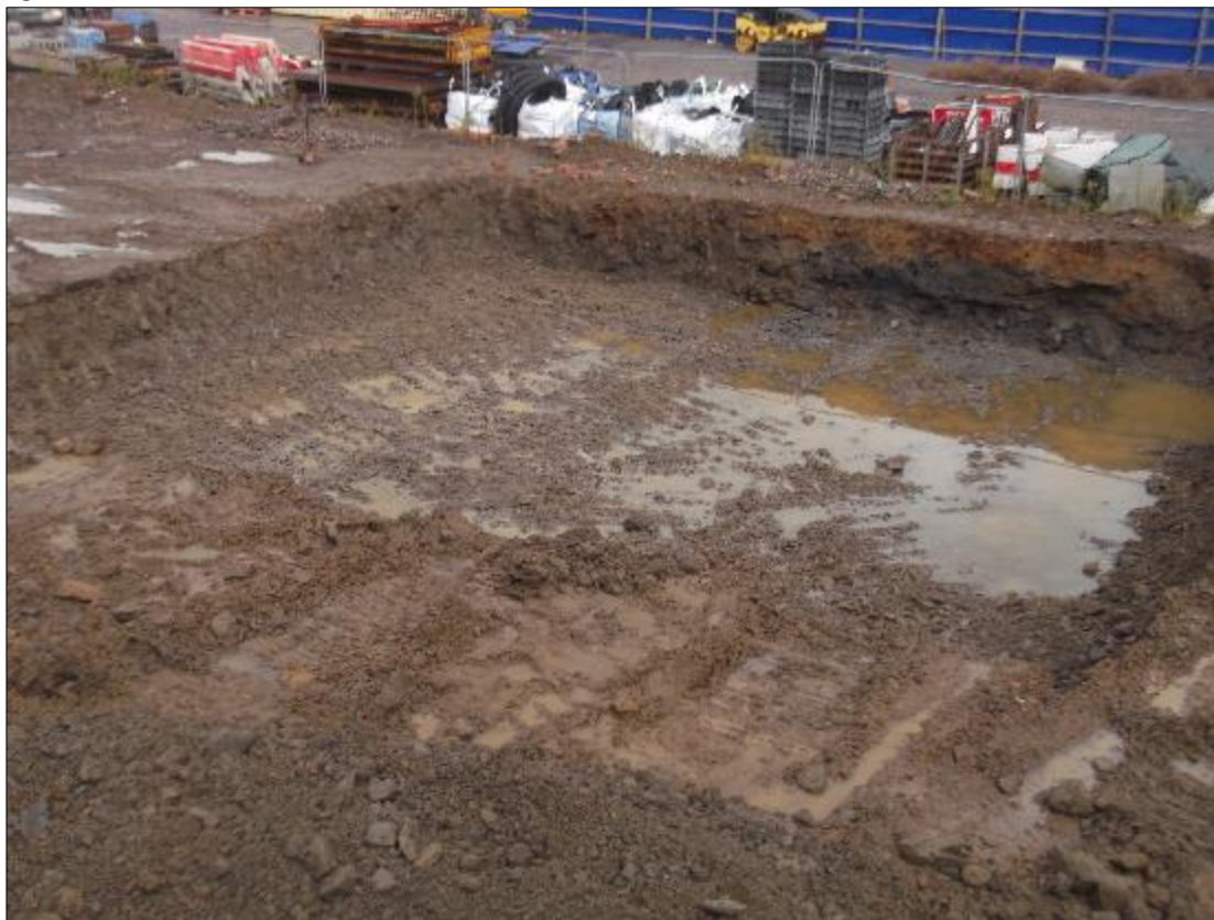
33) Looking north over IP4076 RBSL failure excavation.
