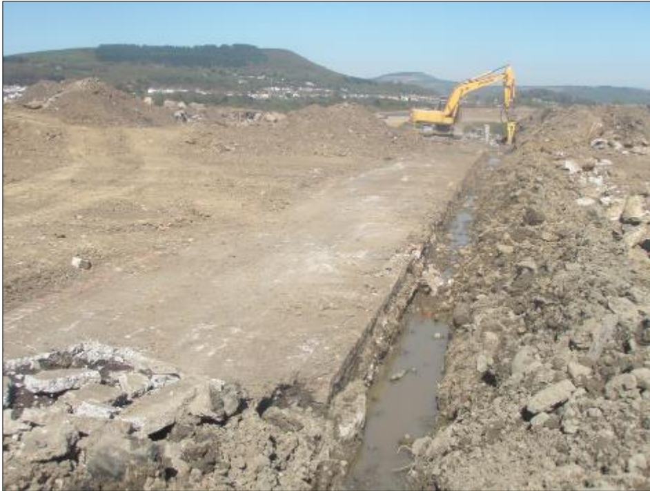
20) Concrete hardstanding (former piperun) exposed during reclamation, on breakout found to contain three metal pipe sections – see photo (21)
