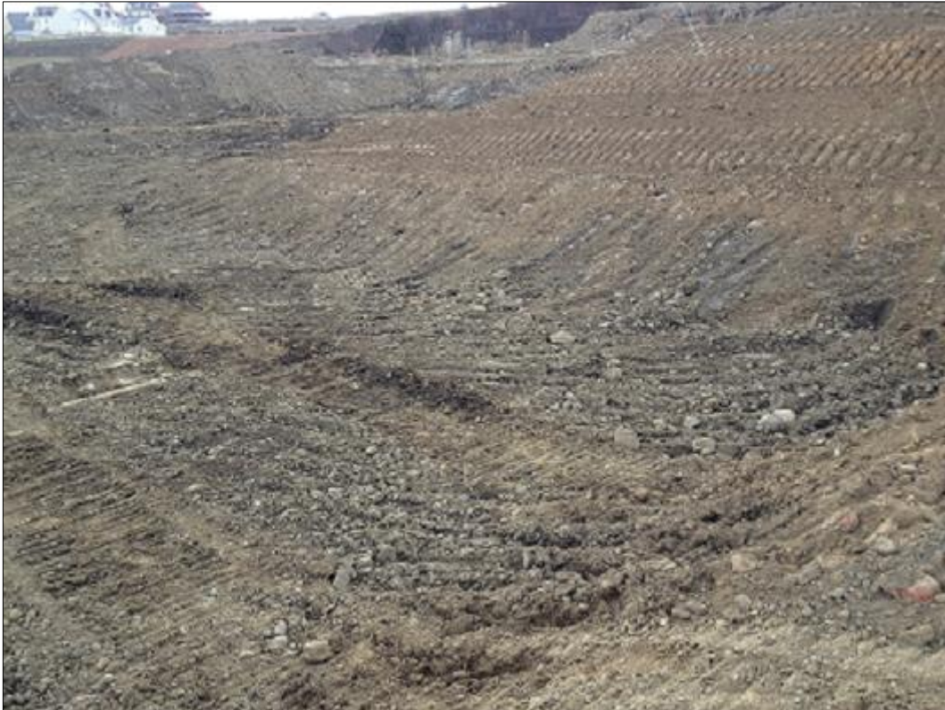
5) Area of removal of moderate surface Staining V/O 2/3 – See 5041216-ATK-REM-2118
