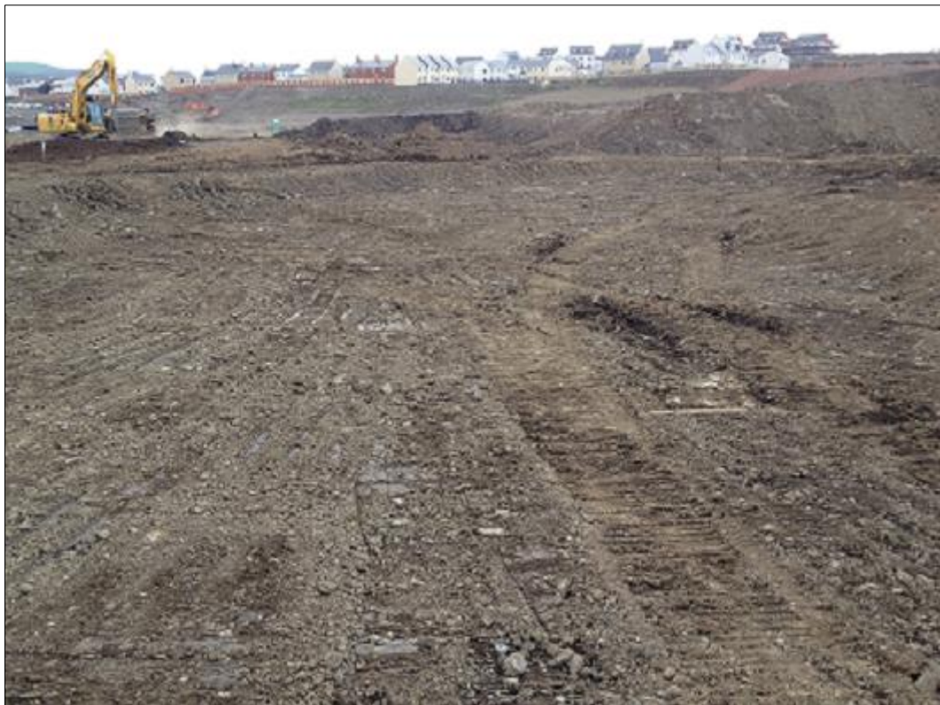
6) Area of removal of moderate surface Staining V/O 2/3 – See 5041216-ATK-REM-2118
