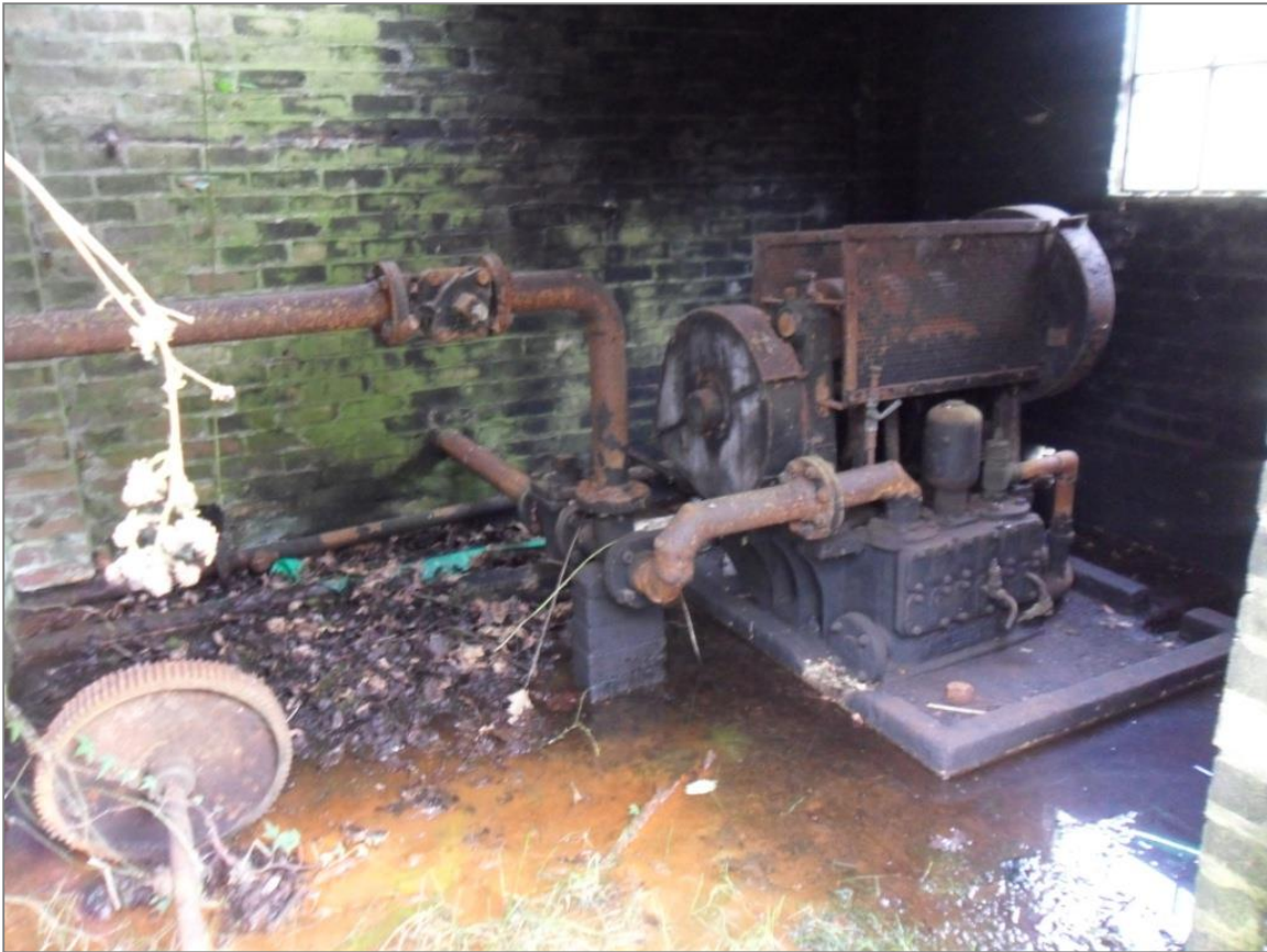
Photograph 19: SSR API separator ancillary building and machinery
