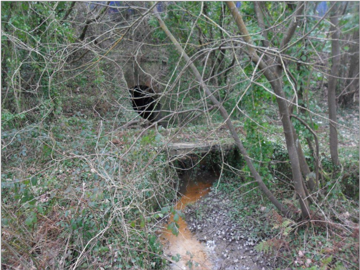
Photograph 23: Ochreous effluent from the SSR separators.
