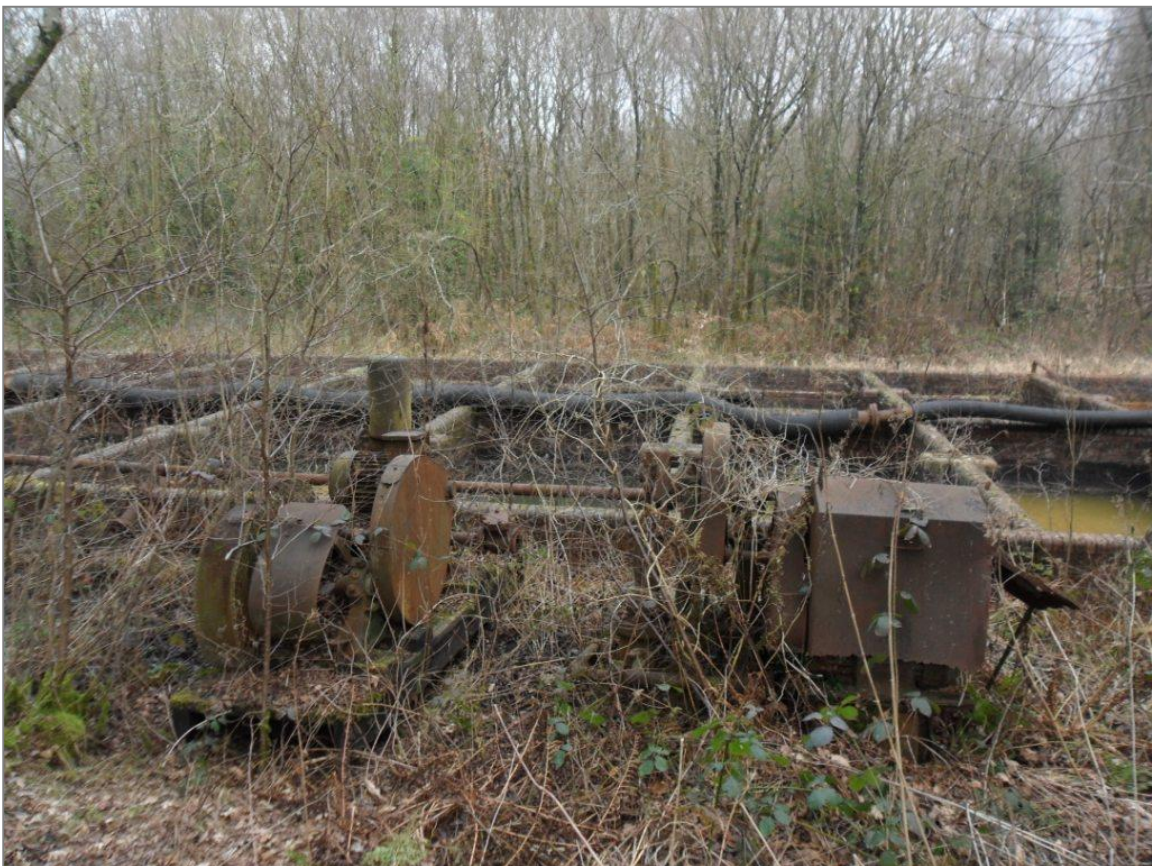
Photograph 20: SSR API separator ancillary building and machinery.
