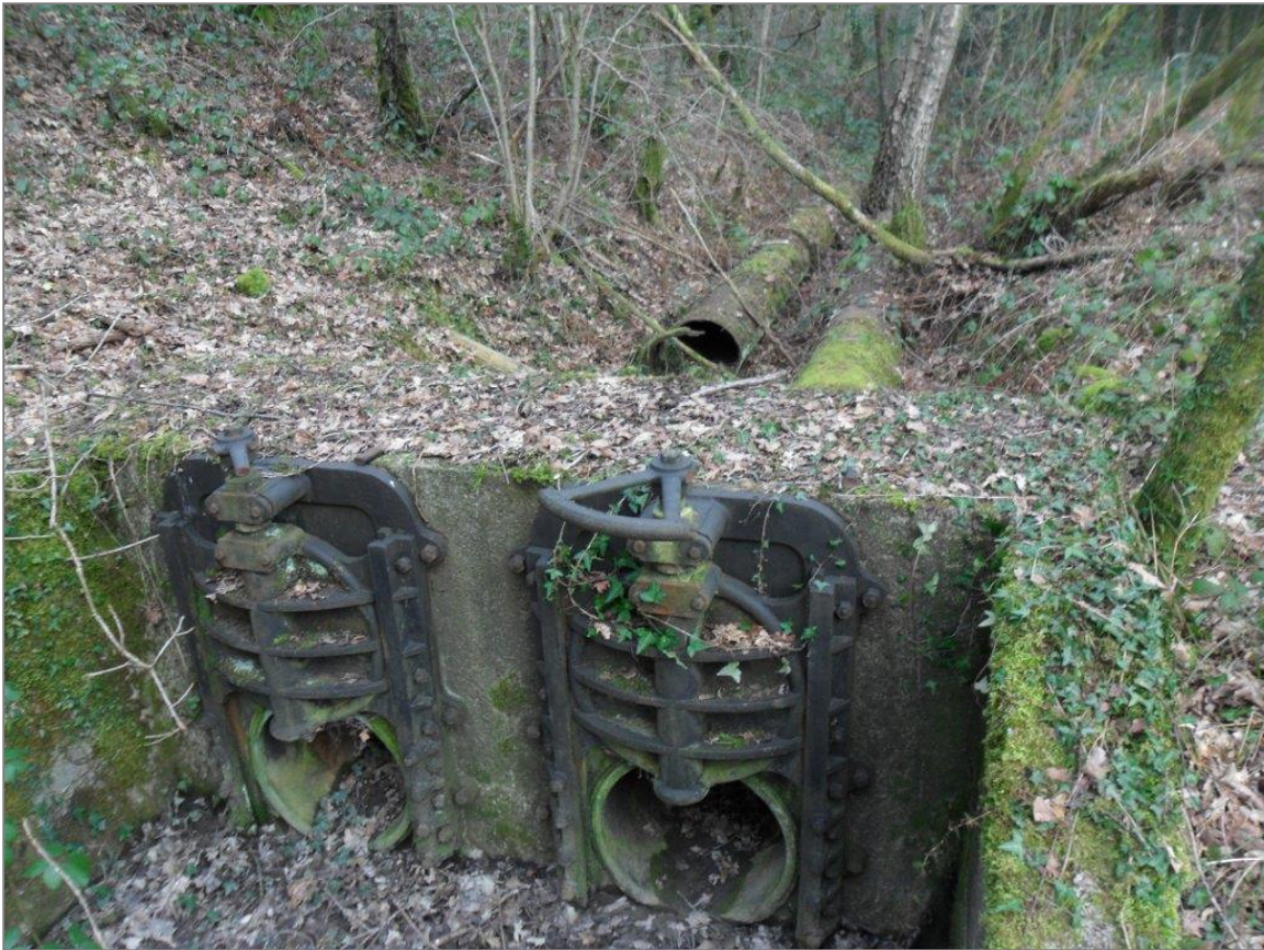
Photograph 21: Valved discharge with steel pipes used to draw down the NSR at times of heavy rainfall.
