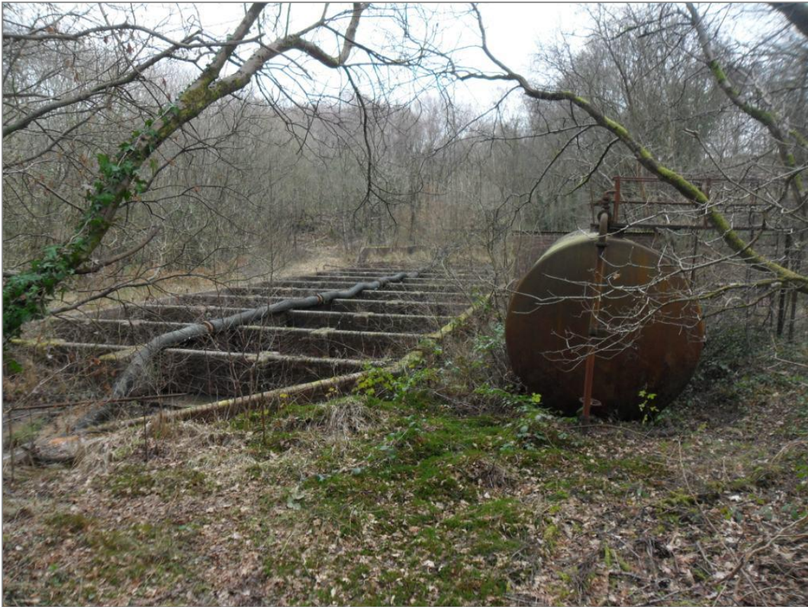
Photograph 17: Operational brick constructed South Site Reservoir (SSR) API separators with ancillary building and above ground storage tank.
