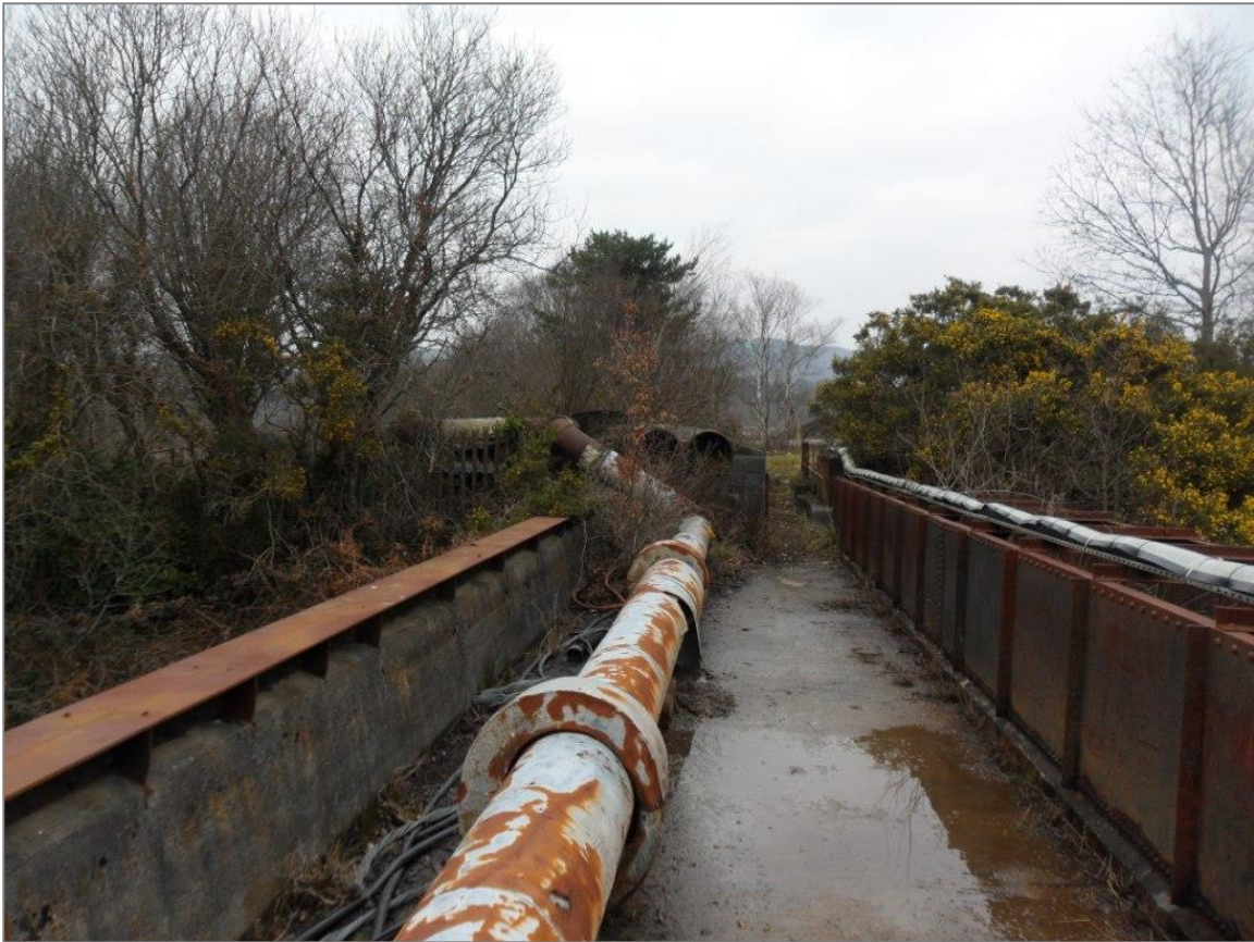
Photograph 9: Northern end of the NSR pumping main. Note where exposed, pipe lagging was identified.
