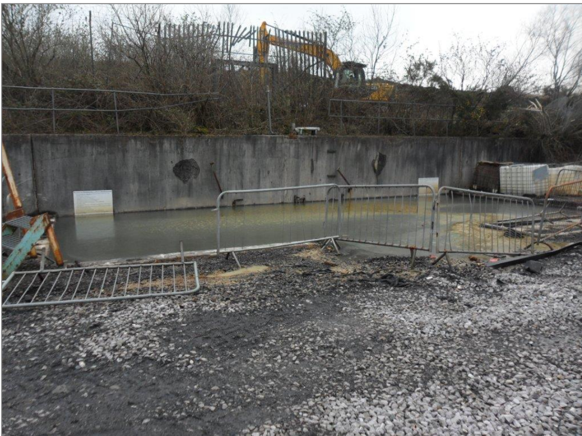
Photograph 16: Flooded former pumping equipment sump.
