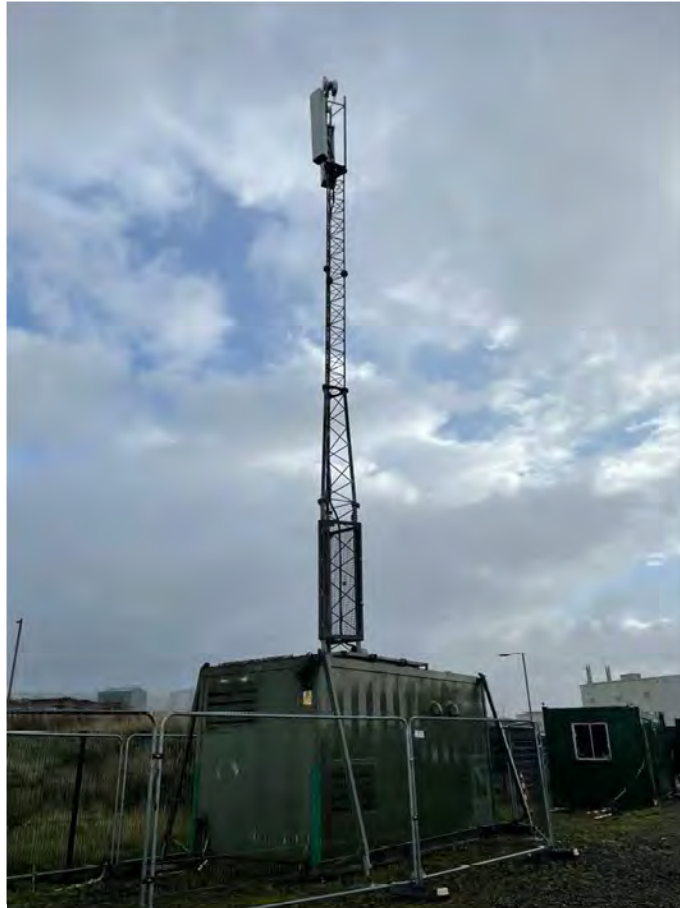
Photograph 7: Temporary telephone mast with associated generator located along the northern boundary of the site, facing south-east.
