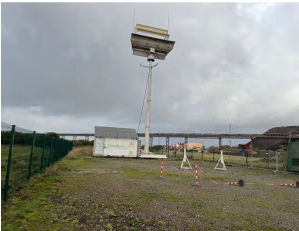
Photograph 6: Existing turbine and generator with 'IES' control container located along the north-western boundary of the site, facing north-west
