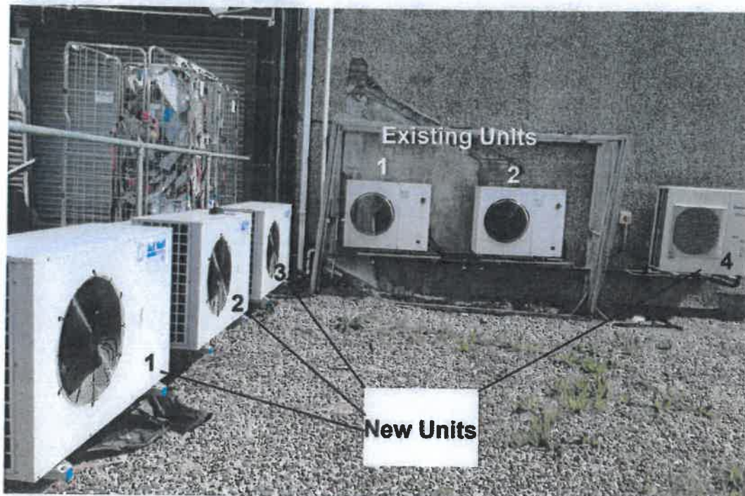
Figure 3.2 – Photo of A/C Units
