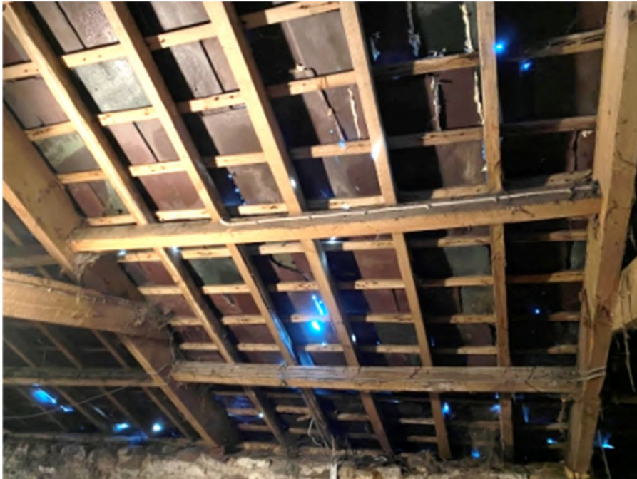
Photograph 40 : Daylight can be seen at numerous locations through the slate roof finishes allowing rainwater to penetrate the barn.
