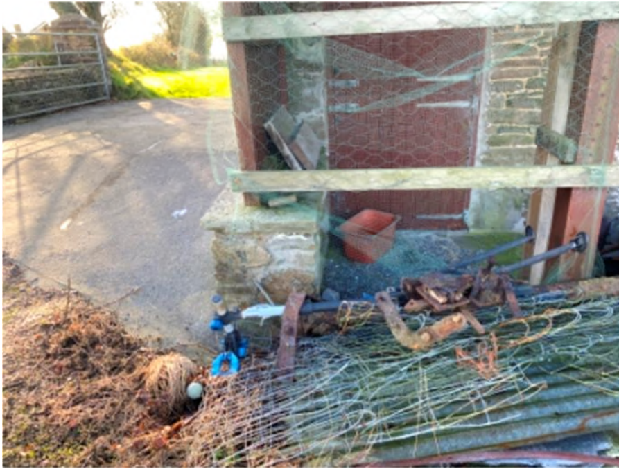
Photograph 37: View showing difference in levels between barn floor and external levels along east gable elevation. External levels are higher along this elevation.
