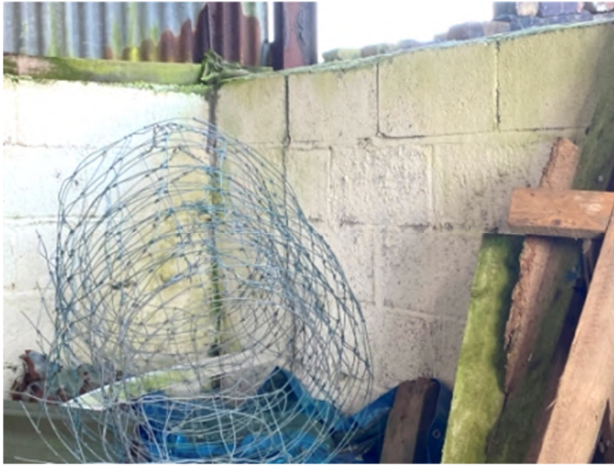
Photograph 25 : View of vertical crack, full height of blockwork, on Dutch barn north elevation.
