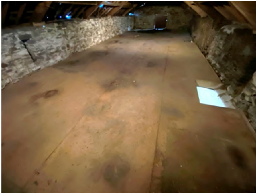
Photograph 44: Areas of first floor timber decking have decayed due to prolonged ingress of rainwater.
