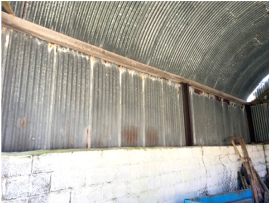
Photograph 22: Internal view of Dutch barn south elevation. No bracing members provided to structure.
