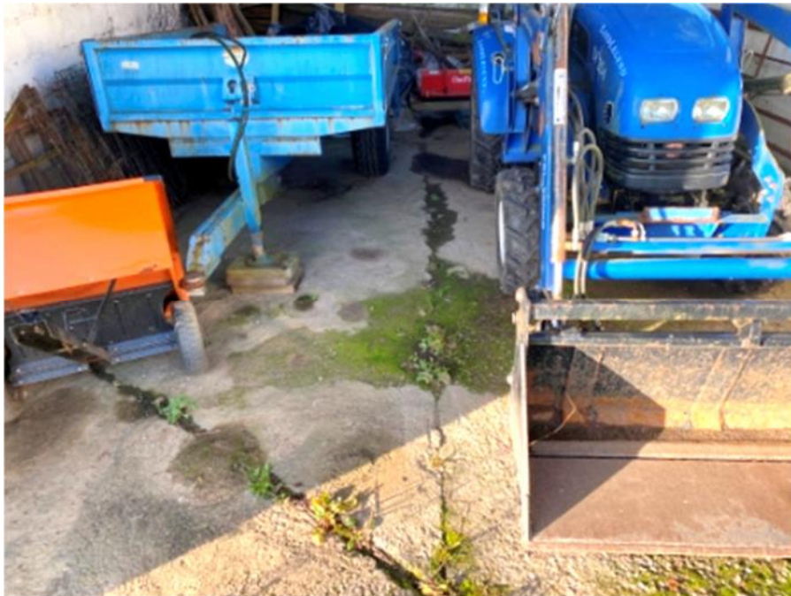
Photograph 20: Crack noted along central joint. Each half of concrete slab has suffered from differential settlement.
