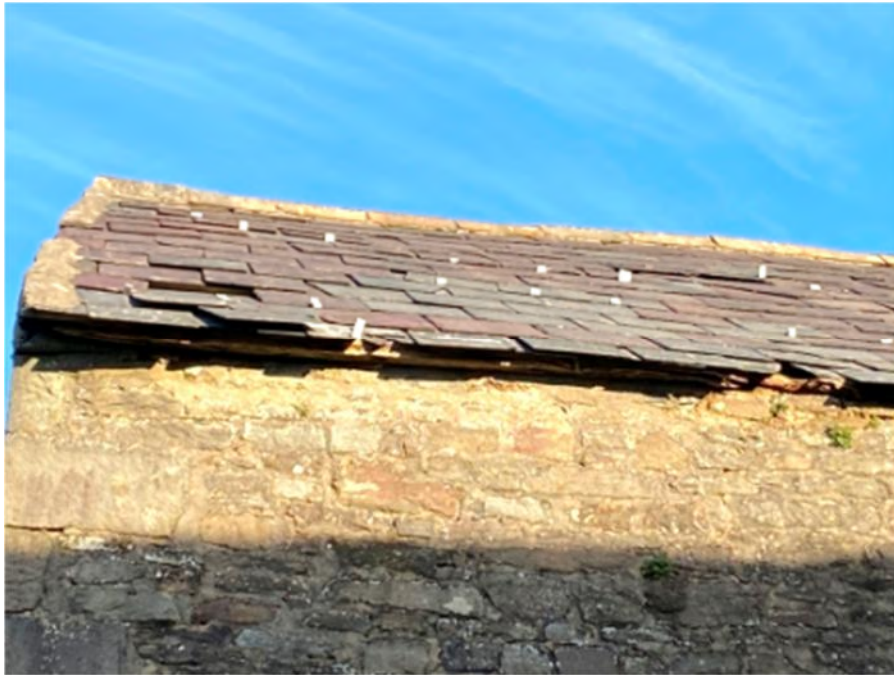
Photograph 15: View of barn roof on southern roof slope. Missing and dislodged slates noted.
