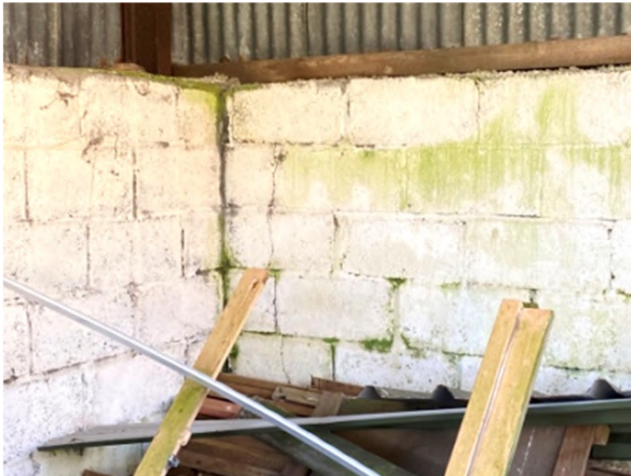
Photograph 26 : View of vertical crack within blockwork, on Dutch barn west elevation.
