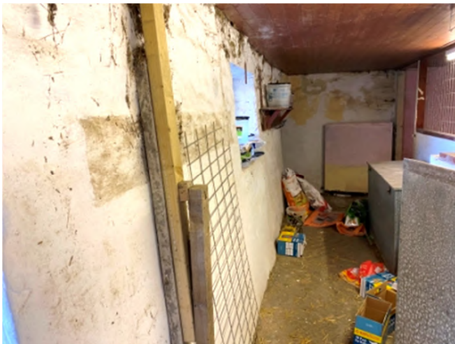
Photograph 46: Internal view of north elevation barn wall shows a significant outwards bow.
