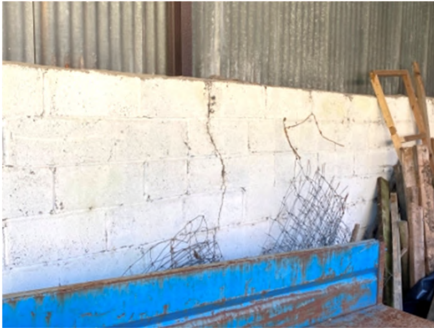
Photograph 23 : View of vertical crack, full height of blockwork, on Dutch barn south elevation.
