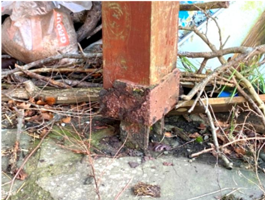
Photograph 54: View of decayed steel post shoe support. Steel shoe shows significant amount of rust.
