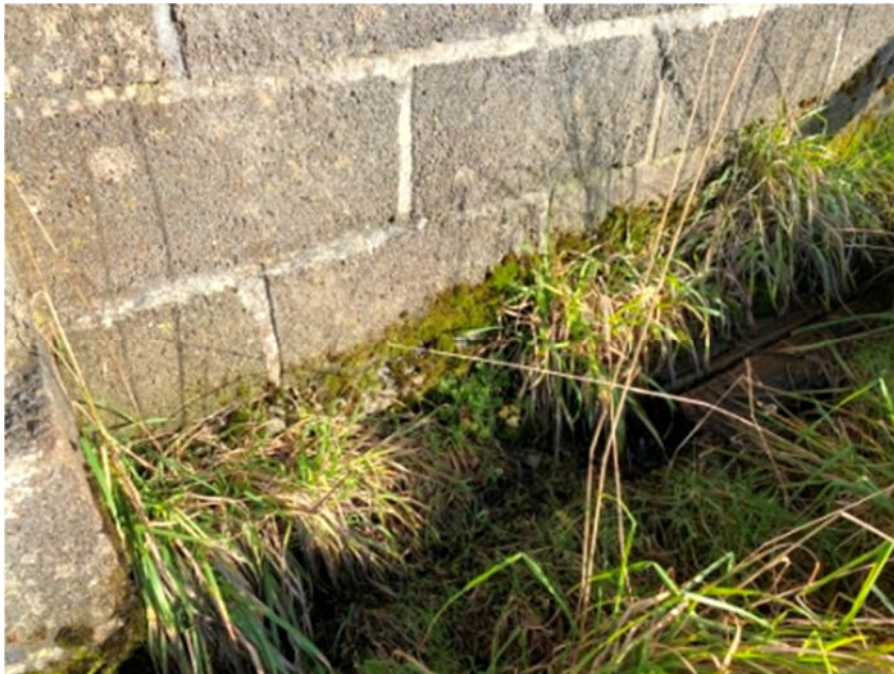
Photograph 18: .Perimeter walls of Dutch barn appear to have been constructed off perimeter of concrete floor slab. Concrete edge is exposed along the southern elevation.
