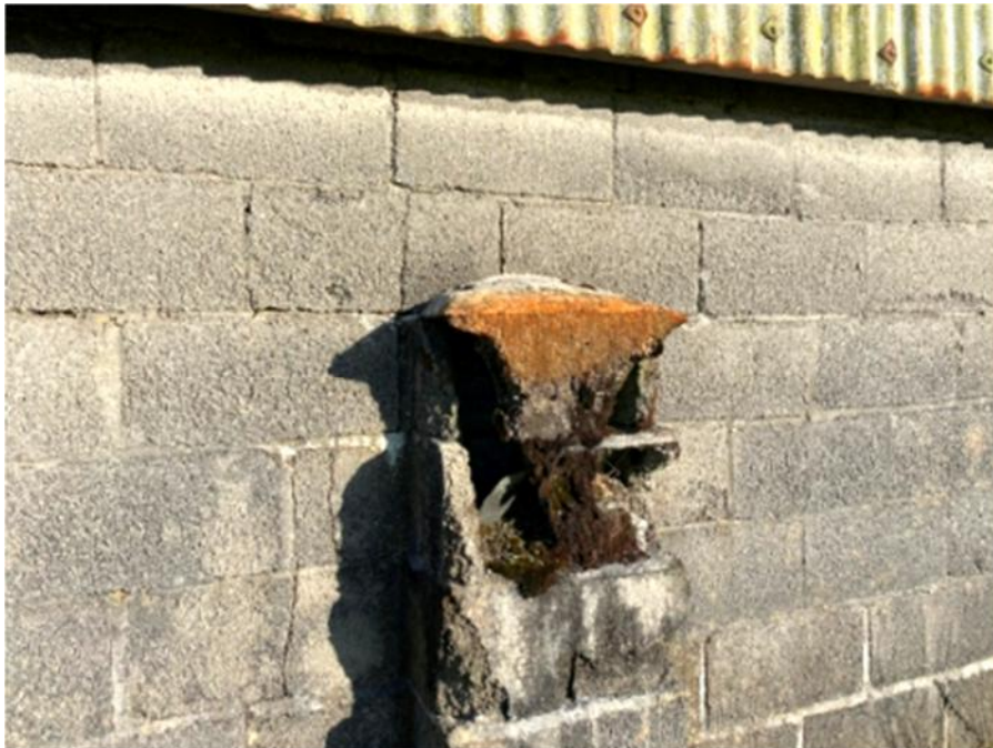
Photograph 16: External blockwork pillars on south elevation of Dutch barn have decayed.
