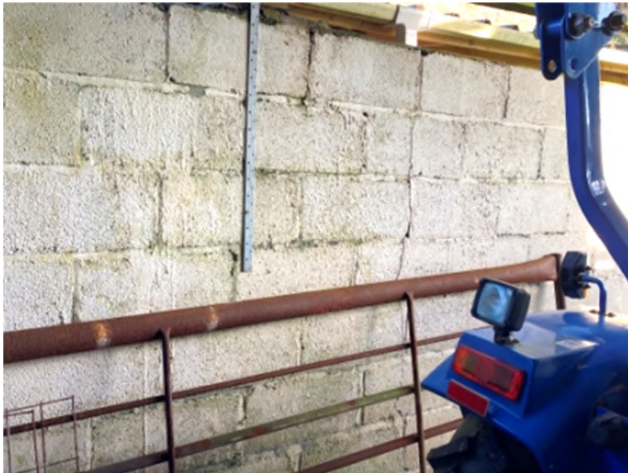
Photograph 24 : View of vertical crack, full height of blockwork, on Dutch barn north elevation.
