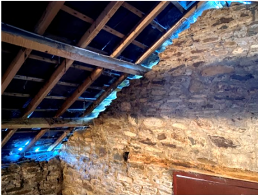
Photograph 43: Timber purlin ends are built over end gable walls and are exposed to the elements.
