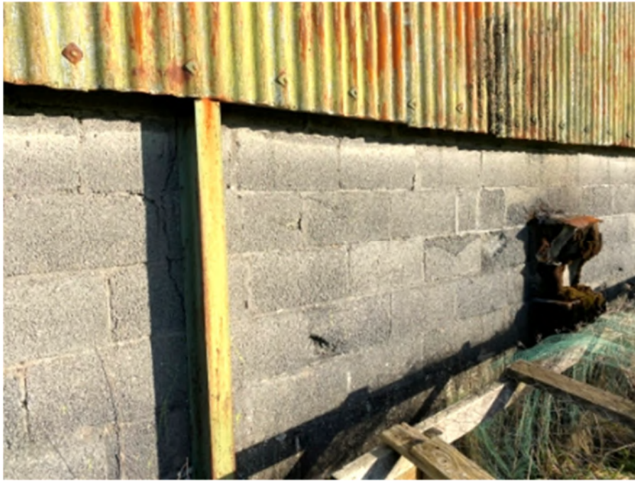
Photograph 17: Dutch barn support steelwork shows evidence of decay due to exposure.
