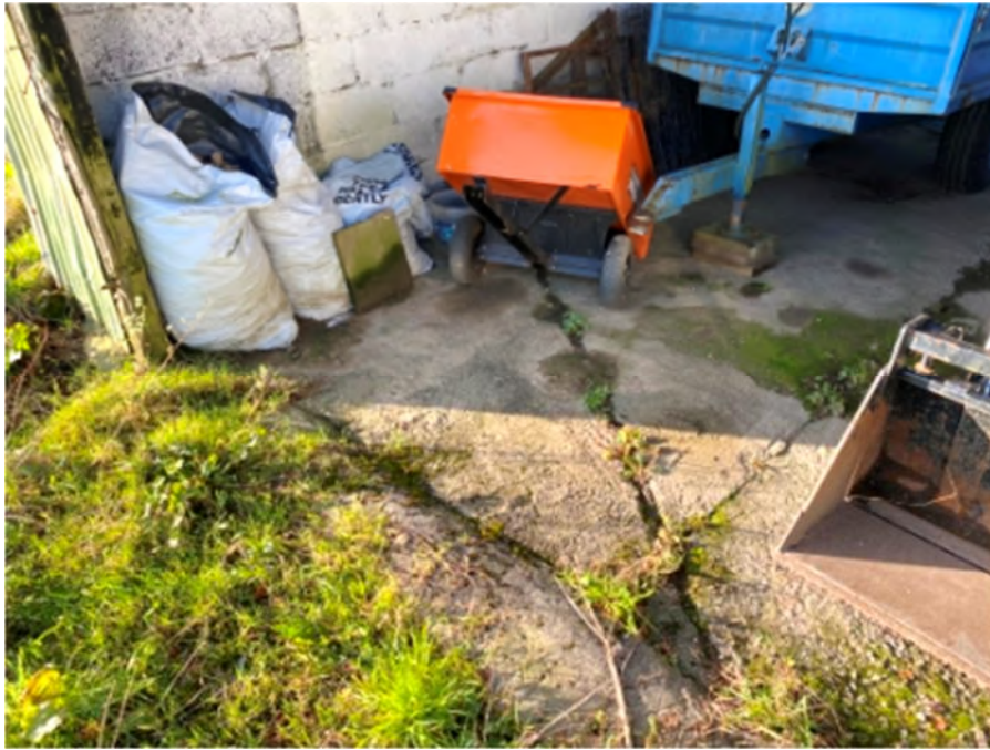
Photograph 19: View of Dutch barn concrete floor slab which has failed at the south east corner.
