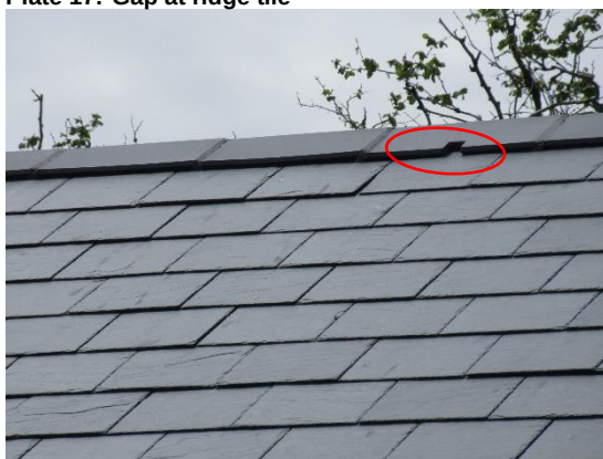
Plate 17: Gap at ridge tile
