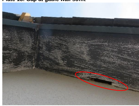
Plate 18: Gap at gable wall soffit
