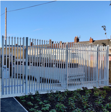
External refrigeration plant cage (Back of House) - Palisade fencing
