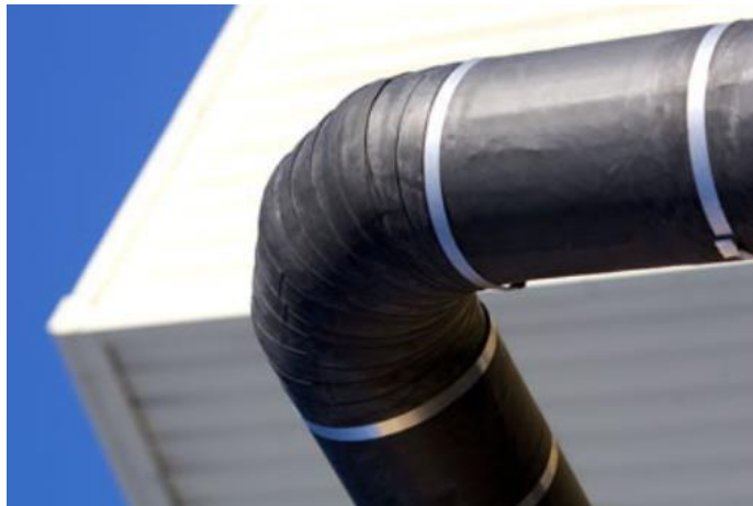
Figure 3 - Typical PIB Pipework finish
