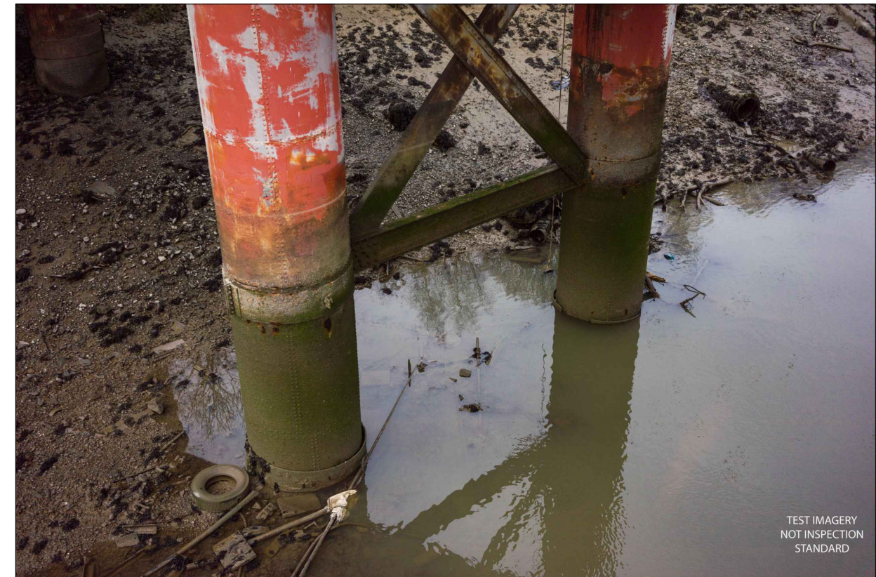
PHOTO - SHOWING DEFECTIVE STRAPPING AT THE BOTTOM OF CAISSONS
