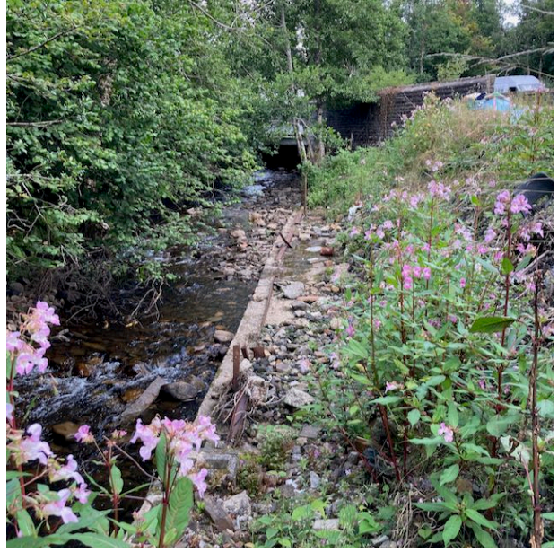
Figure 2. Collapsed bank, looking north.
