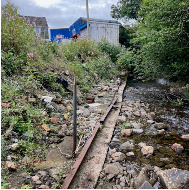
Figure 1. Collapsed bank, looking south.
