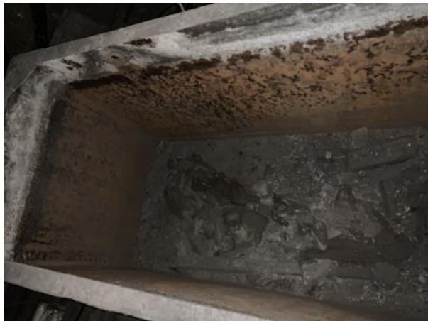
Photo 27: Water Tank in Roof Void Three
