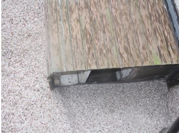
Photo 29: Damage in Foundation of Timber Cladding on North Eastern Extension
