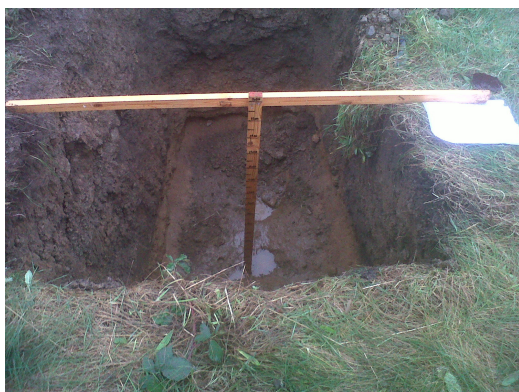
Photograph shows Trial Pit 1 after 120mins with water fully drained away.
