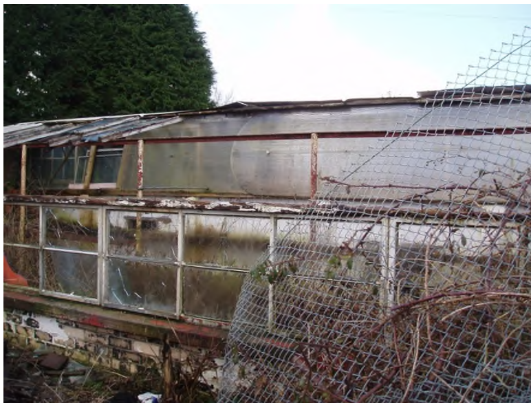
Partially collapsed glasshouse roof (building 1b)
