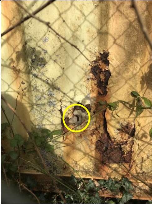
Photograph 30: Example of rusted holes on the south east face of Building 1.
