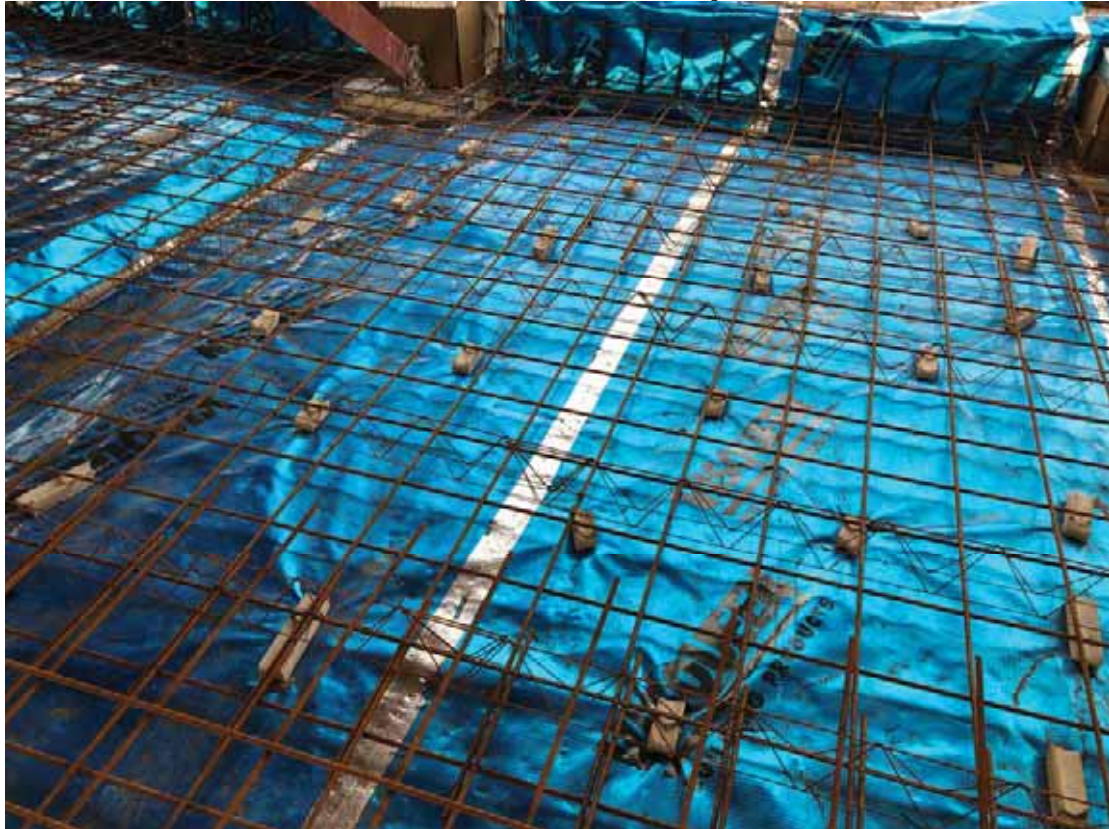
Plate 3 Sealed Joint – Visit 2 (01/04/2021)
